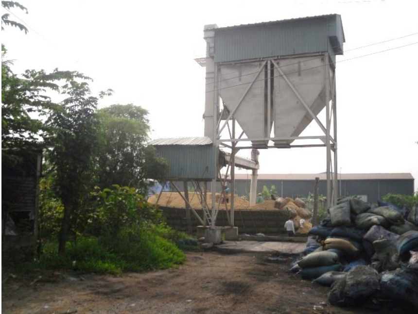
Figure 33. Rice husk unloading system at Din Hai steam power plant (Photo By Duc Vu).
