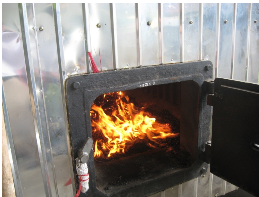
Figure 17. Bagasse pellet boiler in Ben Tre province (Photo by Arvo Leinonen).
