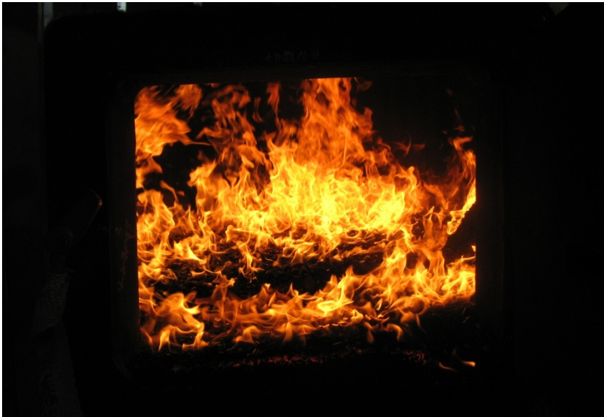
Figure 57. Biomass pellets burning in the steam boiler (Photo by Arvo Leinonen).
