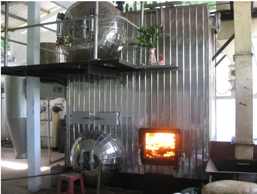
Figure 53. Boiler burning pellets in Chin Thi malt plant (Photo by Duc Vu).
