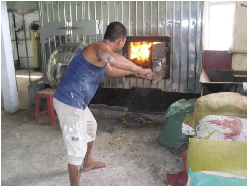
Figure 58. Manual ash disposal from the boiler (Photo by Duc Vu).
