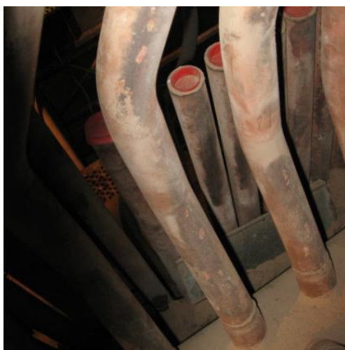
Figure 1. Some of the damaged evaporator tubes.
