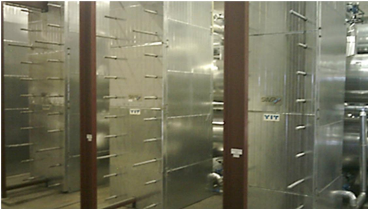
Figure 30. Heat exchangers at Laagna pumping station.
