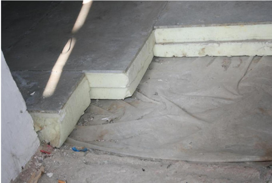
Figure 25. In building II-18, the floor of an attic was also insulated with XPS-based plates.
