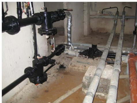
Figure 14. Pipelines in a basement.
