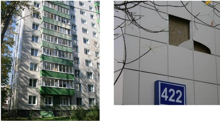
Figure 23. A II-18 building renovated with the ventilated façade renovation system “Gradochist” (“city cleaner” in English).
