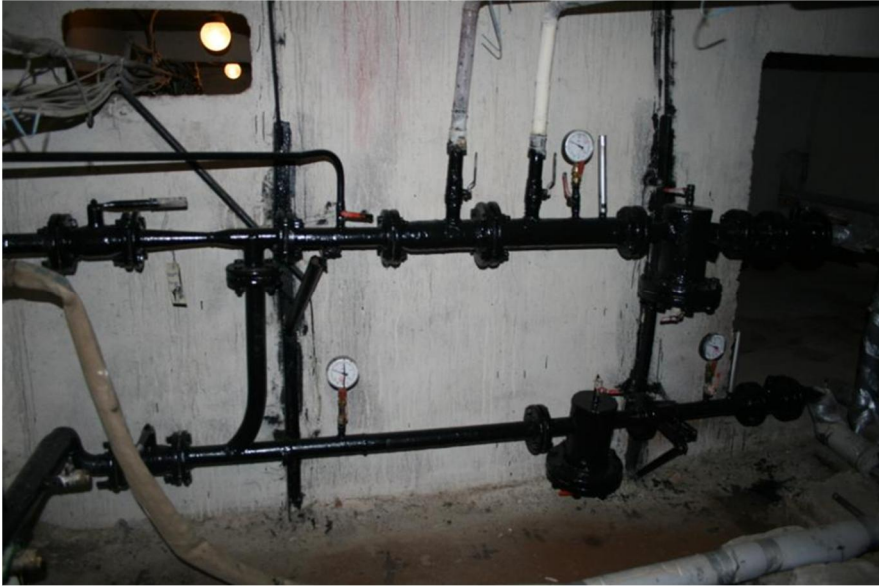
Figure 17. Heat distribution pipes in a building.
