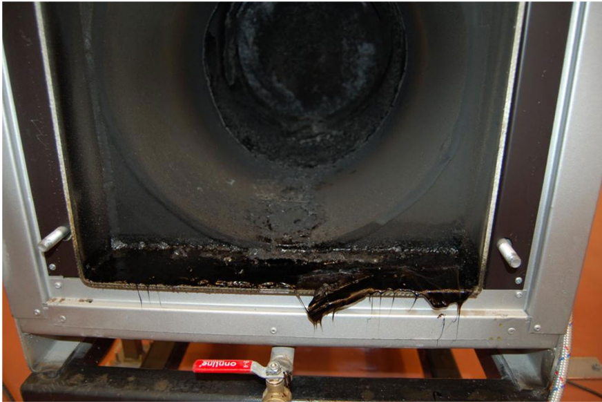
Figure 7.11. Small boiler tested with low quality bio-oil. Coke formation on the walls of the boiler and spill of oil can be seen.
