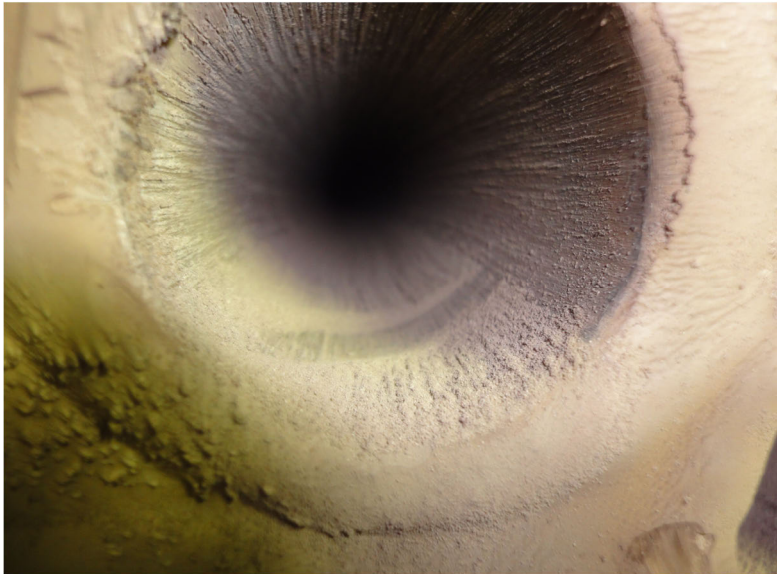
Figure 7.13. Some particle contamination may be seen on the fire tubes of the bio-oil boiler. However, the amount of unburnt in solids is very low.
