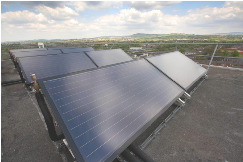
Figure 1. EcoPod Boilers and Solar Thermal Array.
