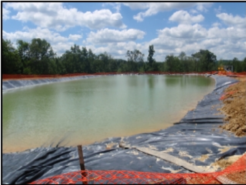
Figure 4.2.3.2. Lined Fresh Water Supply Pit from the Marcellus Shale Development in Pennsylvania (source: ALL Consulting, 2008).
