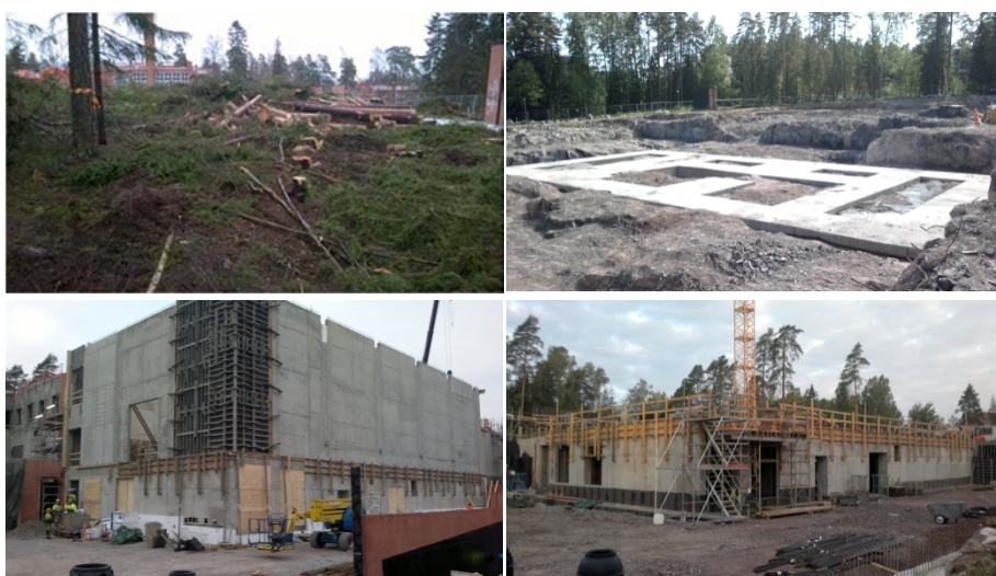
Figure 3: Progress on construction of THE VTT Centre for Nuclear safety in 2014, CW from upper left, January, June, September and December.
