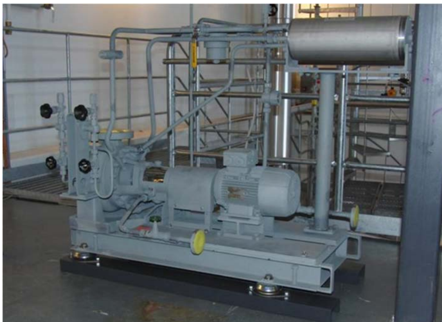
Figure 8. New main circulation pump of the PWR PACTEL test facility.
