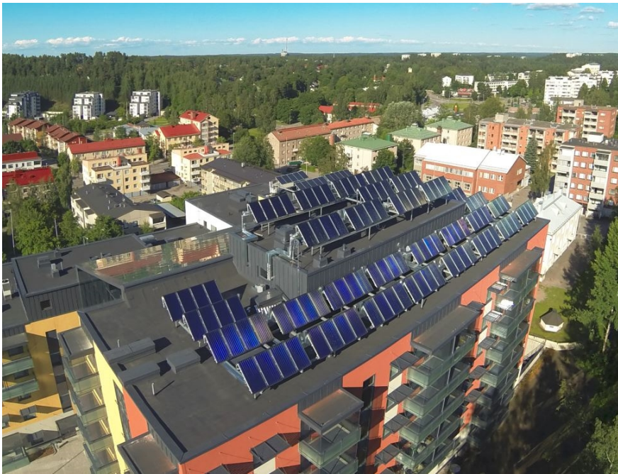
Figure 41. The 240 m 2 collector system installed on the roof of new apartment building in the city of Lahti (Savosolar, 2014).
