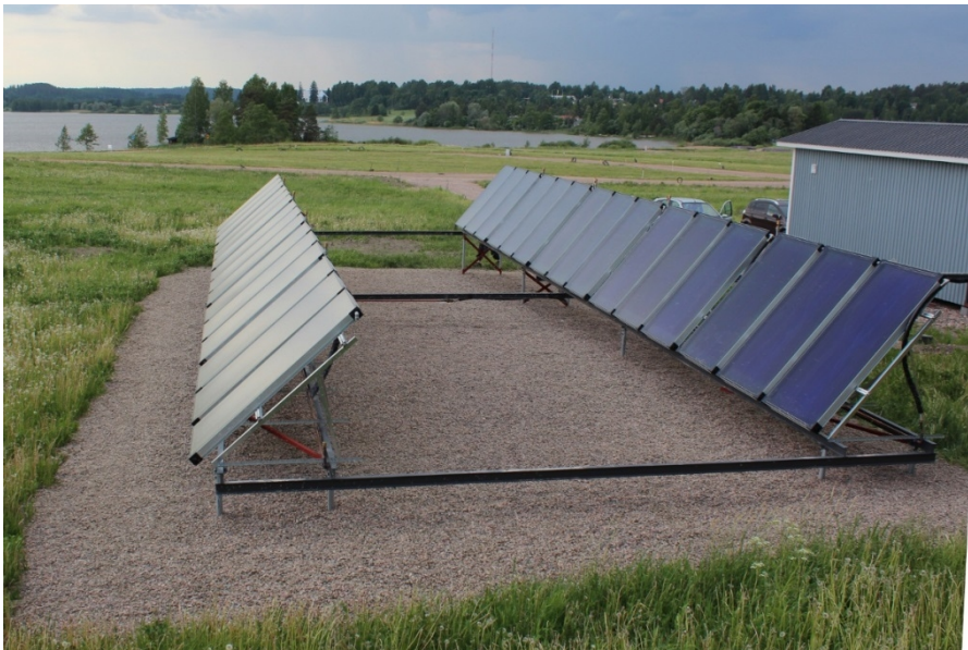
Figure 40. Solar collector field (60 m 2 ) connected to district heat network in Myrskylä, Finland (Savosolar, 2013).
