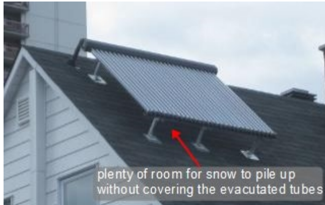
Figure 25. Evacuated tube collector installed with extra space (Rimstar, 2012).
