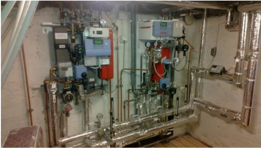
Figure 14. Two apartment level substations for 150 m 2 (left) and 300 m 2 (right) heated areas including both DHW and SH services.
