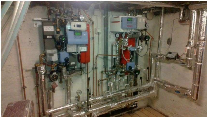
Figure 21. Two apartment level substations for 150 m 2 (left) and 300 m 2 (right) heated areas including both DHW and SH services.
