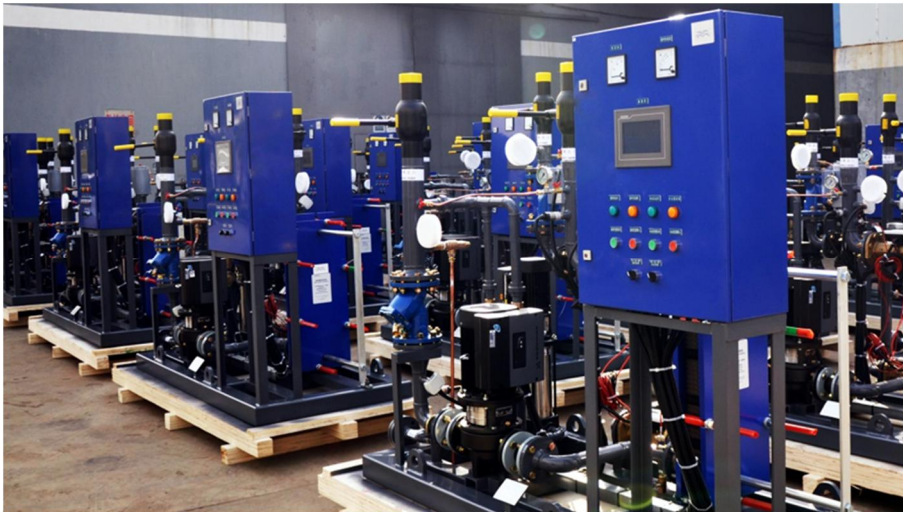
Figure 2. Building level substation (BLS) with capacity of about 10 000 m 2 in the factory ready for shipment to Chengde, Hebei Province, China.
