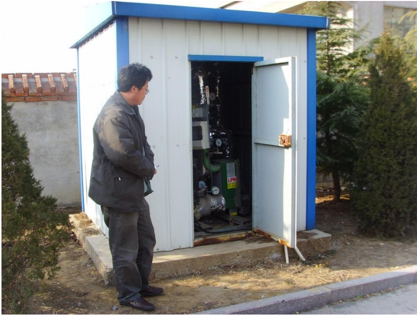
Figure 13. A BLS installed outside the building in a thermally insulated cabin in Weihai, Shandong province in year 2007 (source: A. Nuorkivi).
