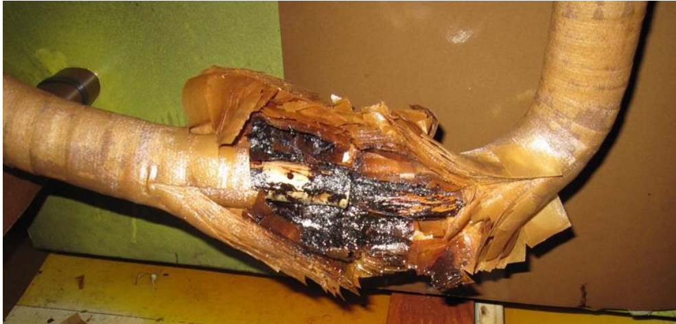
Figure 3. Overheated connection in a transformer.
