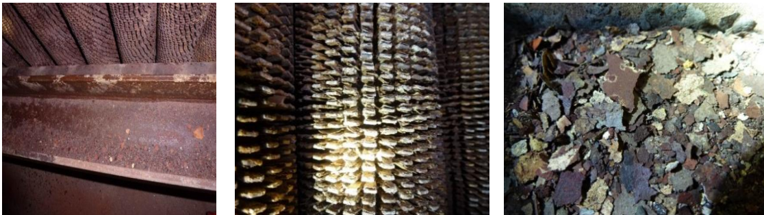
Figure 4. IJmond 1 boiler inspection results. Left: sticky layers. Middle: flakes on fins. Right: flakes collected on flooring.
