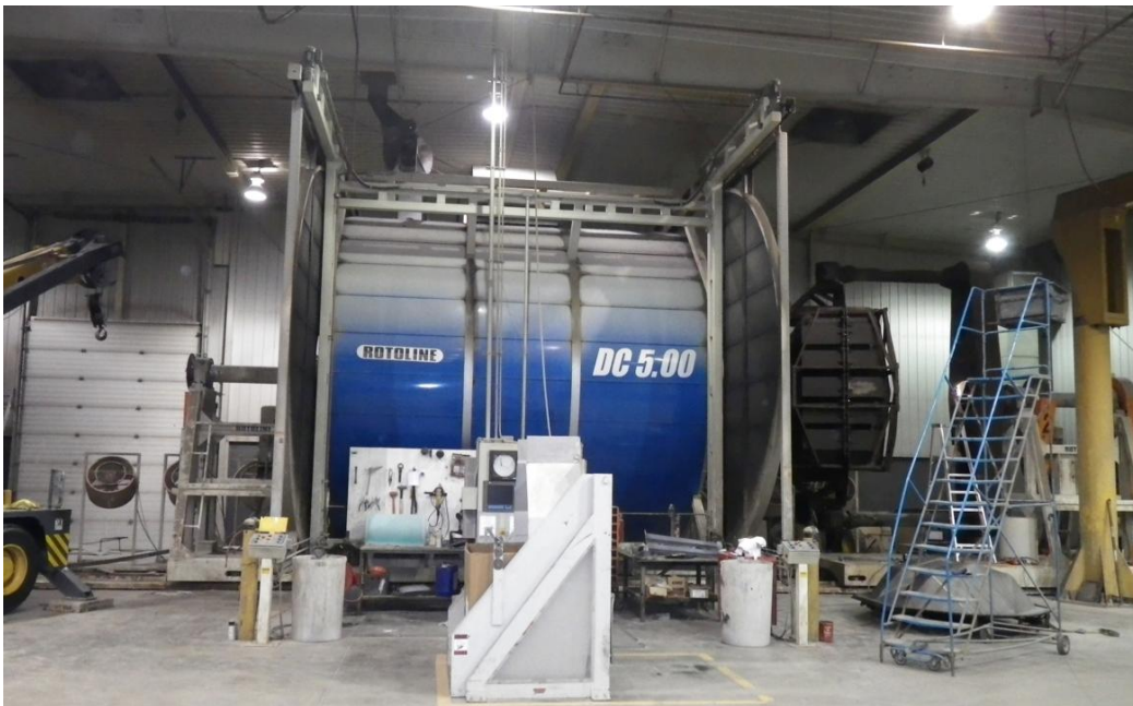
Figure 2. Installation after failure and shut-down.
