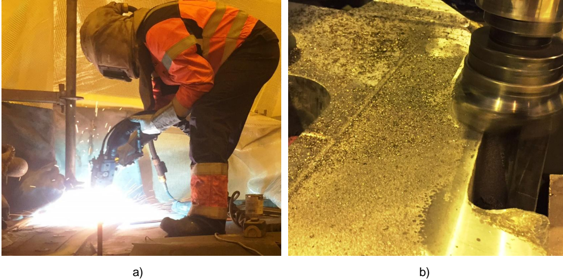
Figure 7. a) Surface restoration by thermal spray; b) machining of the flange surface after coating (photos: J. Sipilä, Telatek Service).
