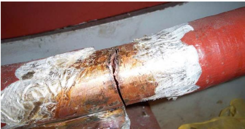
Figure 2. Crack in the stator winding lead.
