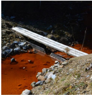
Figure 9. Thompson weir (V-Notch weir) (photo: Tiina Kaipainen, GTK).
