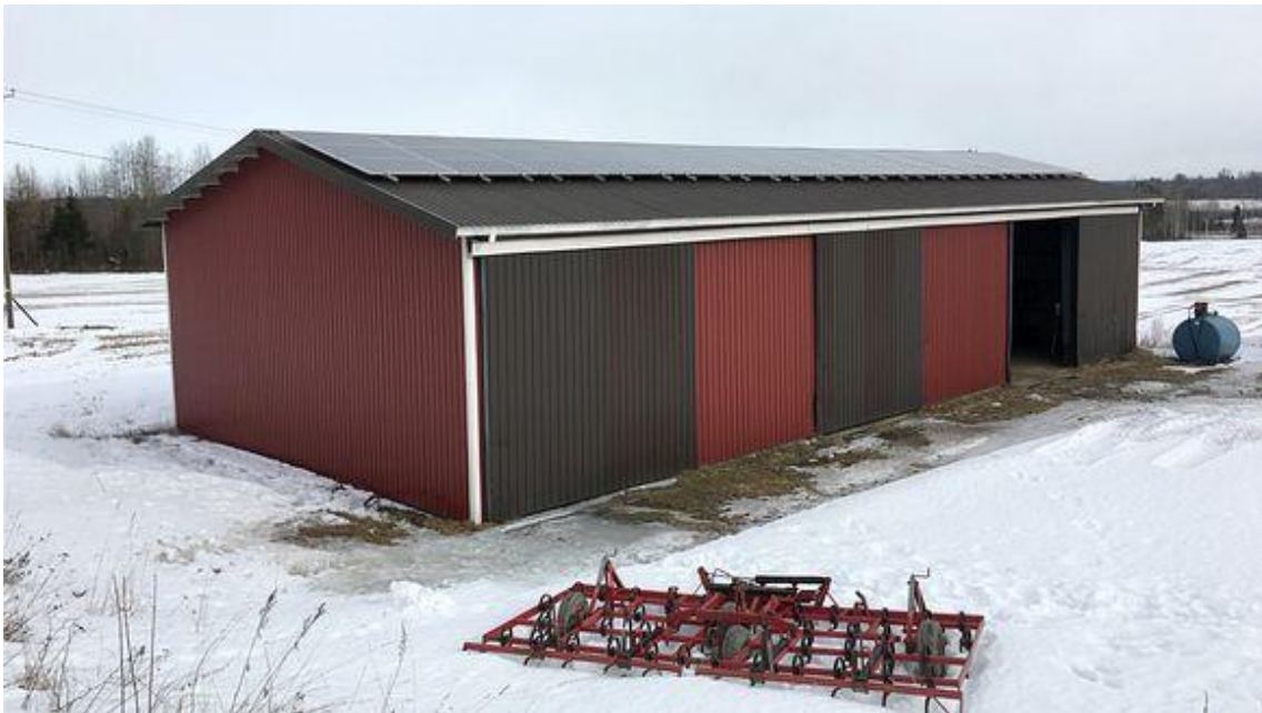
Figure 36. A PV system (peak power 11 kW) in the rooftop of a farm in Lappeenranta. The system produces approx. 20% of the annual power consumption of 180 GJ (50 MWh). [133]
