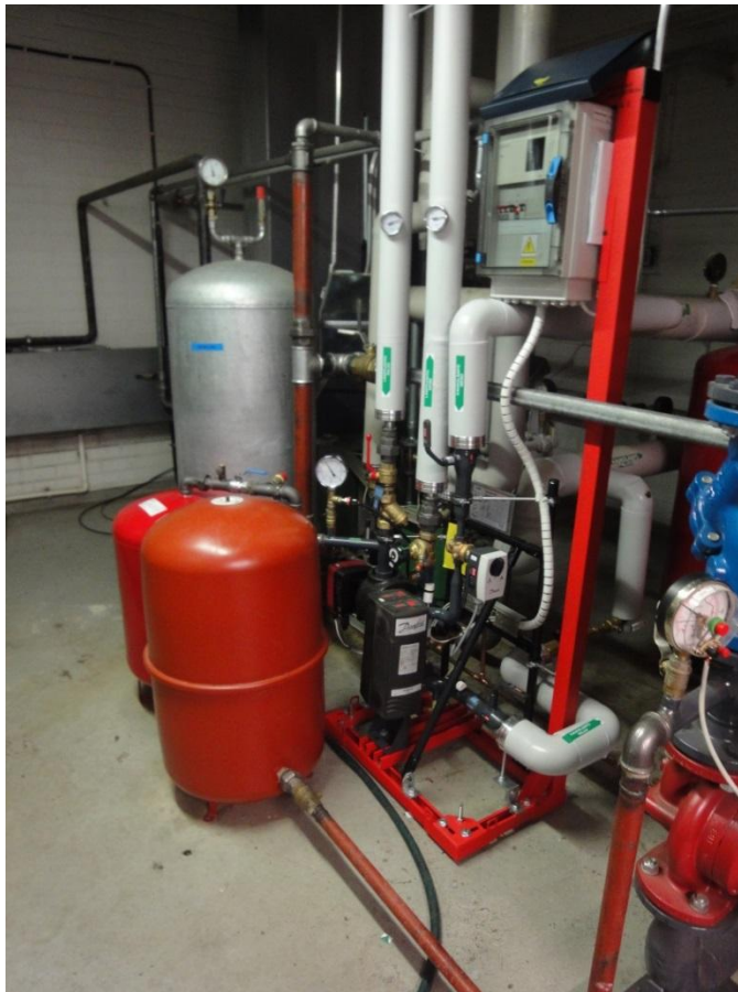
Figure 5.6. District heating substation.
