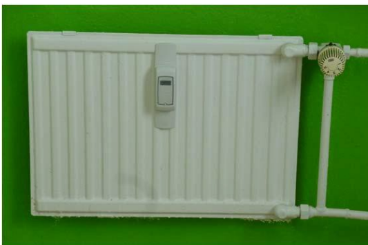
Figure 11. The heat cost allocator on a radiator.
