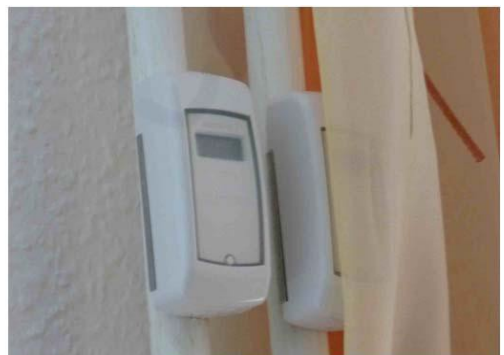
Figure 12. Heat cost allocator on radiator pipes.
