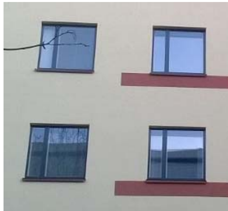
Figure 4. Typical Finnish windows. This is a year 2013 model which replaced a similar window from 1972.
