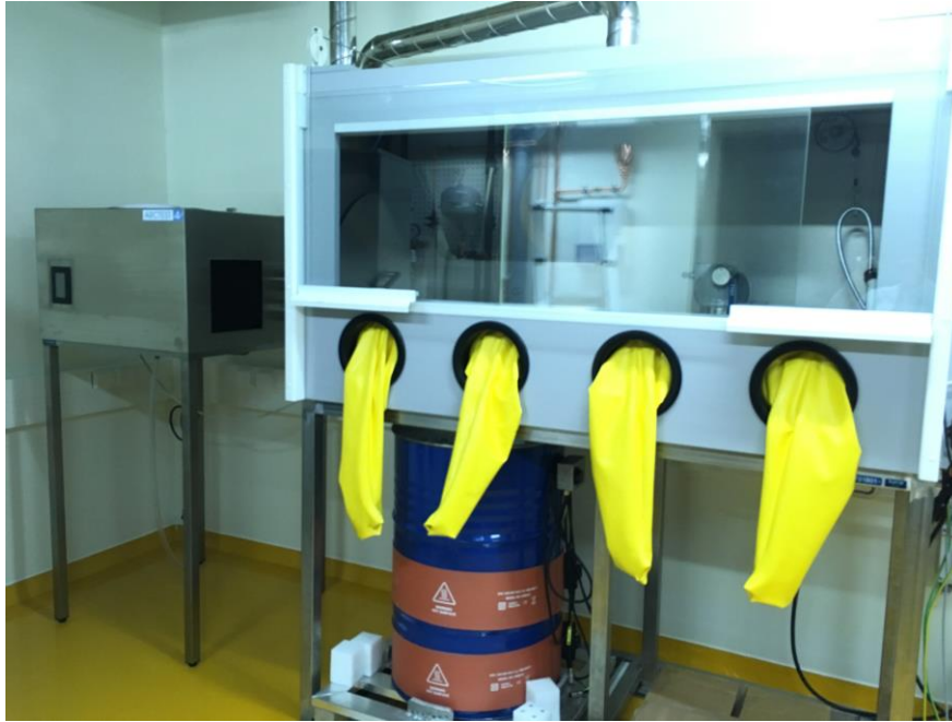
Figure 24. The wet-waste handling cabinet is comprised of two gloved work-stations; the one on the left is for docking a 200 liter barrel that can be heated by the application of thermal bands to facilitate evaporation of water, and the one on the right is a table-top with a mixer for cementation, and space for setting up an ion-exchange resin filter tower.
