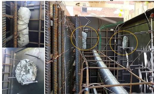
Figure 7. View of the placement of two distinct types of honeycombing – long “sausage” type and flat, round type honeycombing.
