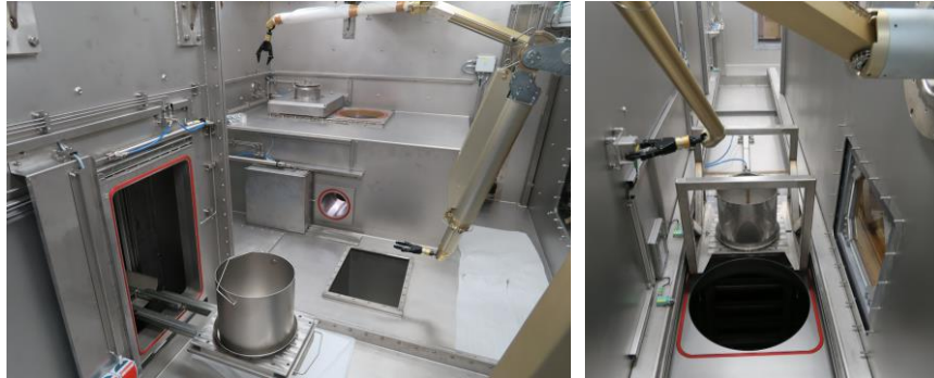
Figure 7. The horizontal conveyor (right) and vertical conveyor (left) work integrally to transport a pail or box containing radioactive specimens between Cells 1.3, 1.6 and 3.1 via Cell 1.7. It has air-tight doors at the top and bottom, so it functions as an airlock between 1.7 and 3.1.
