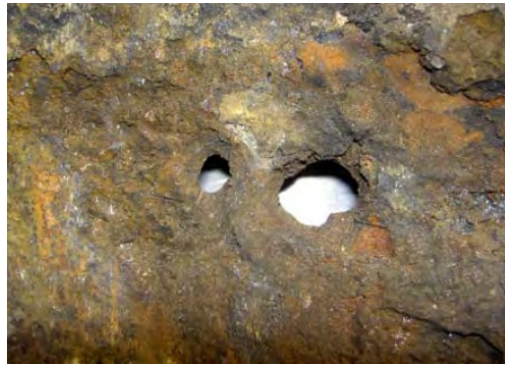
Figure 7. Corrosion damage in the steel liner from Ringhals 2 [Aghili, 2007].
