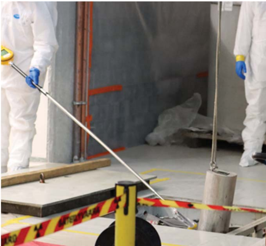
Figure 35. Working methods are developed to minimize radiation exposure risk of the workers.
