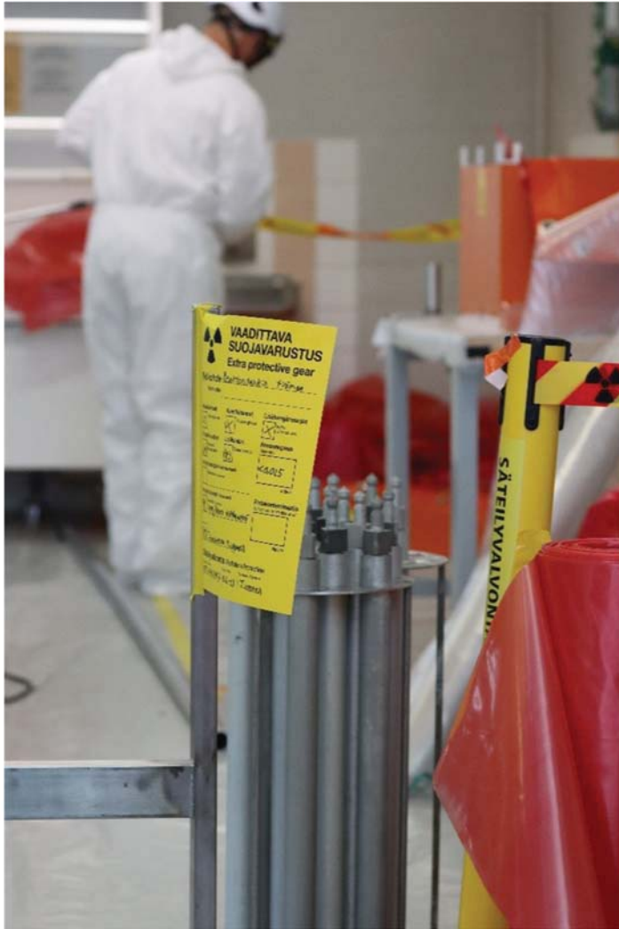
Figure 21. Each radioactive waste component and container requires marking and documentation.
