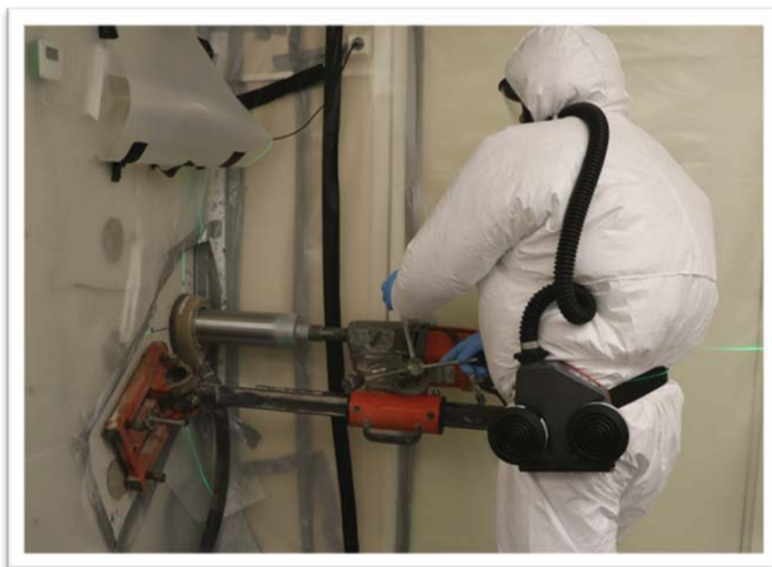
Figure 19. Drilling of activated concrete samples from the biological shield of the FiR 1 research reactor.
