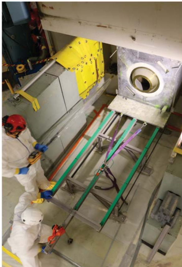
Figure 18. Boron neutron capture therapy (BNCT) station's structures under decommissioning at the FIR 1 research reactor.
