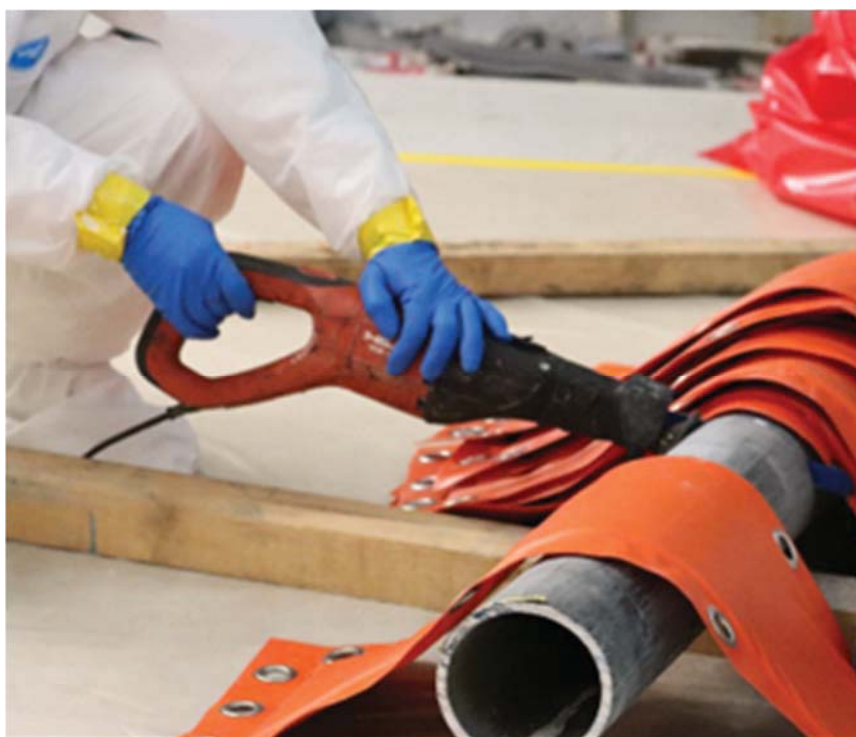
Figure 20. Lead blankets are widely used as a quick way to set up shielding for the dismantling of activated components.
