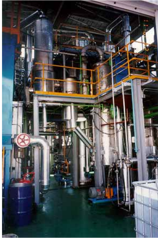
Figure 4. ENEL-RTP Bastardo fast pyrolysis plant (Ensyn Technologies Inc.).
