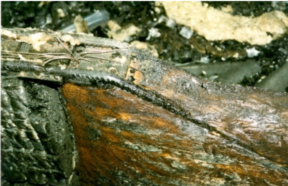
Figure 15. The connection of Beam 2 after removal of the fire protection and the char.
