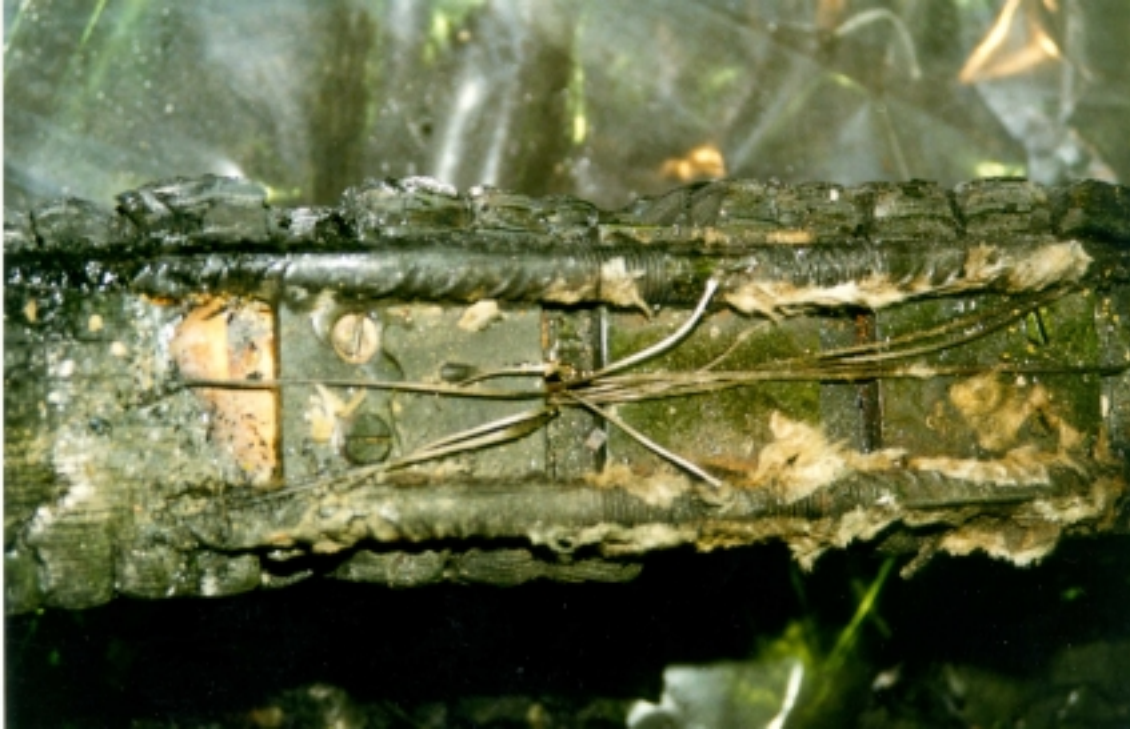
Figure 16. The steel plate of Beam 2 moved about 10 mm when the failure occurred.
