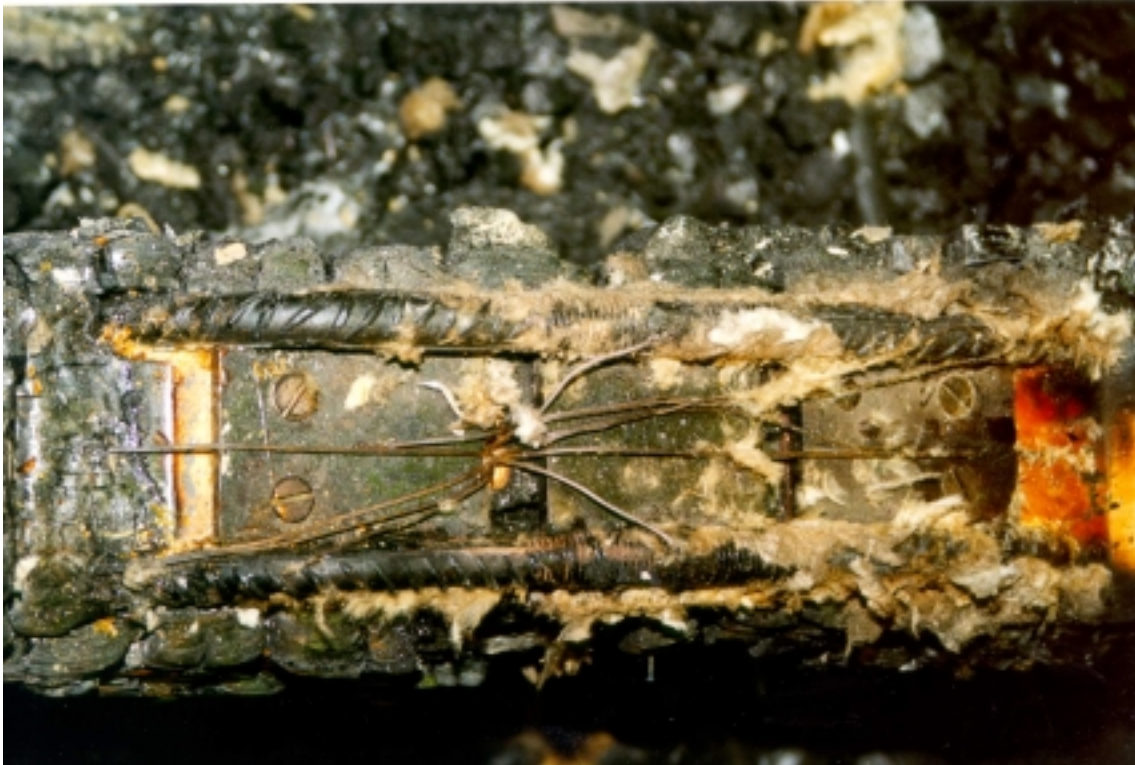
Figure 20. The connection of Beam 3 after removal of the fire protection. The steel plate moved about 10 mm when the failure occurred. The type of failure was like in Beam 2.
