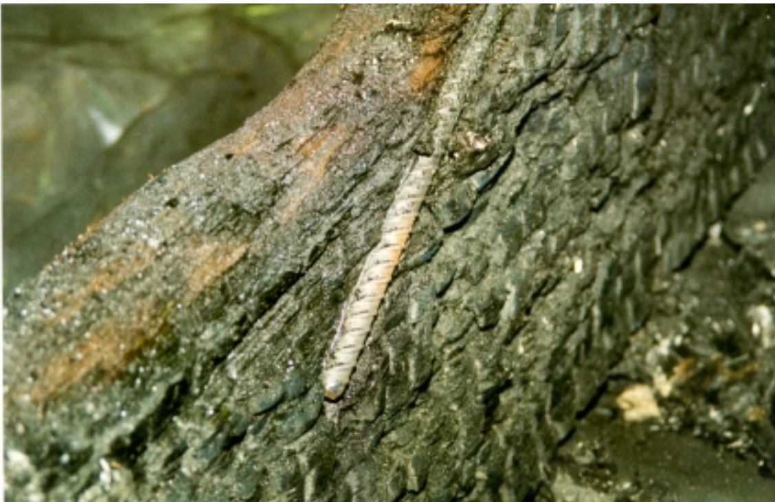
Figure 19. Bare rod in Beam 2.
