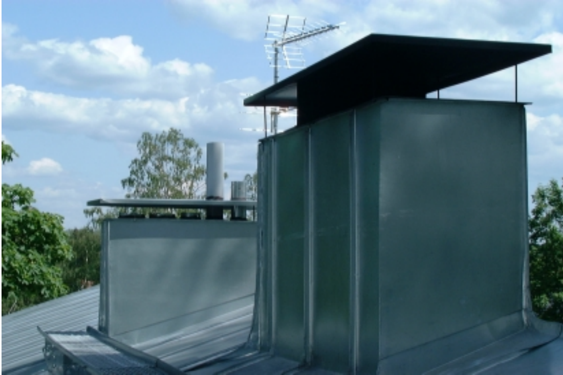
Figure 68. Chimneys and natural ventilation exhaust ducts on the roof.
