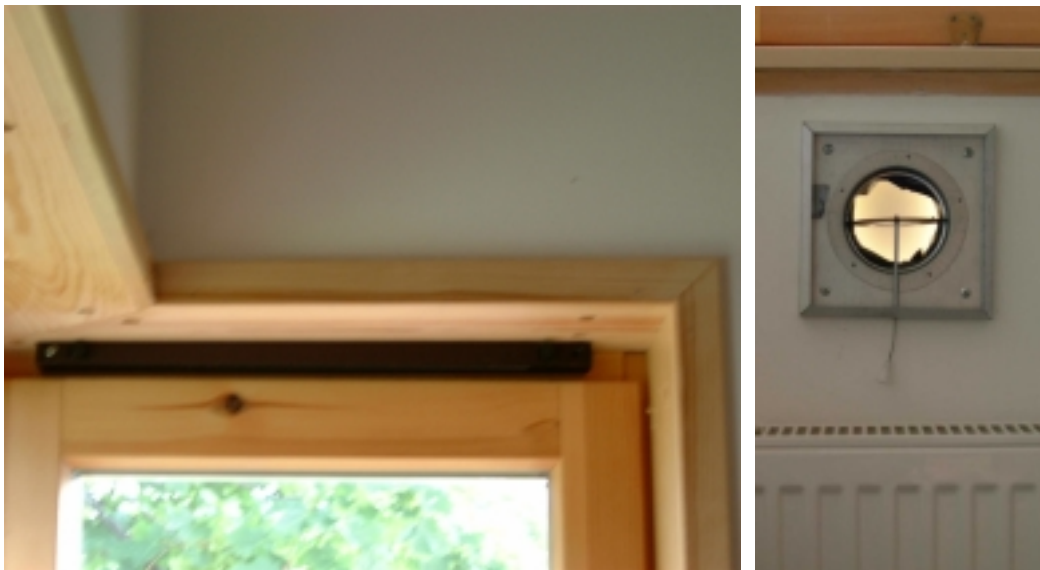
Figure 67. Supply vents located in the window frame (a) and exterior wall (b).
