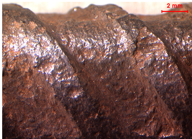
Figure 51. Wire brushed rebar, \varnothing 12 mm, of corrosion class 3.
