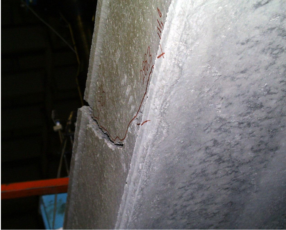
Fig. 37. PT400B. Detail of soffit after failure
