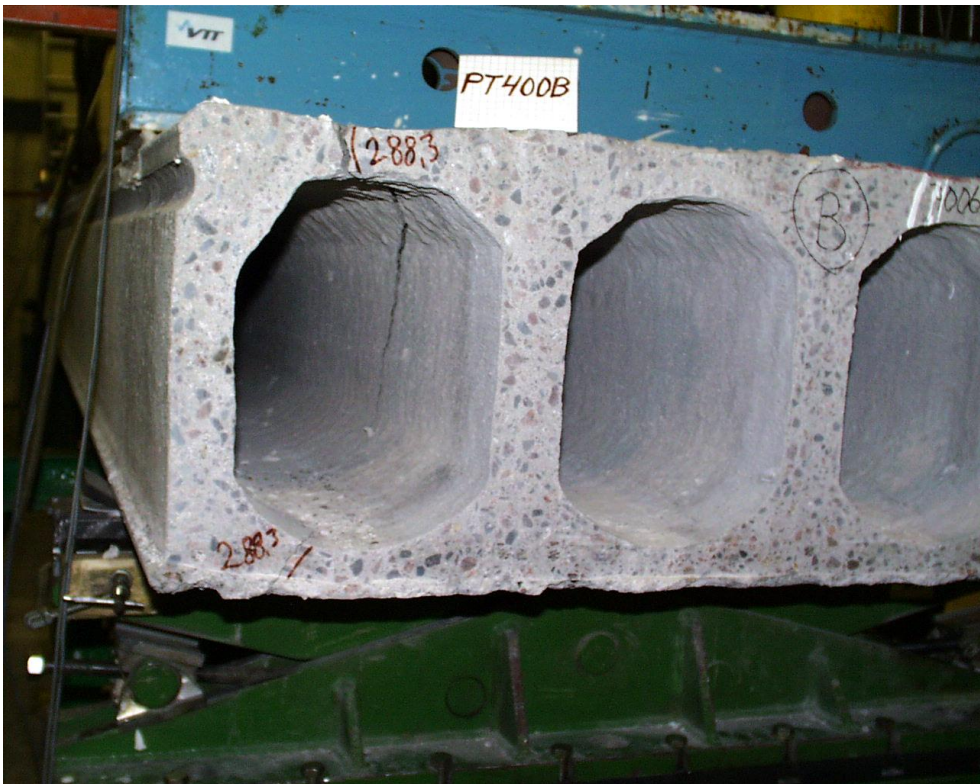
Fig. 34. PT400B. Cracking of the cantilevered end.
