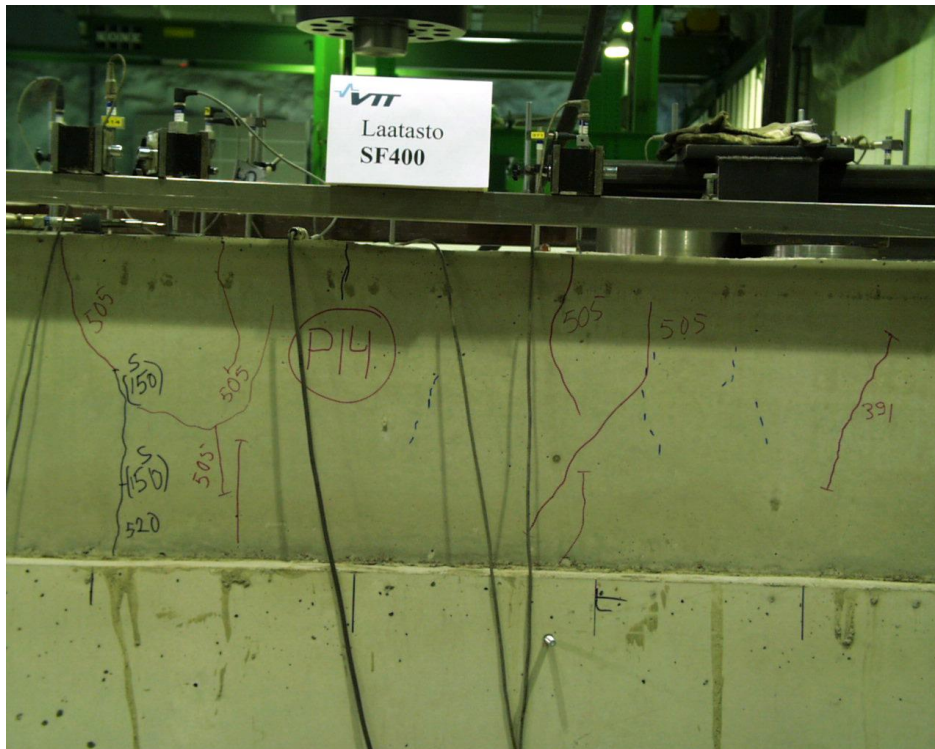
Fig. 18. PF400:14. Cracks in tie beam at the loaded end shown in red colour.
