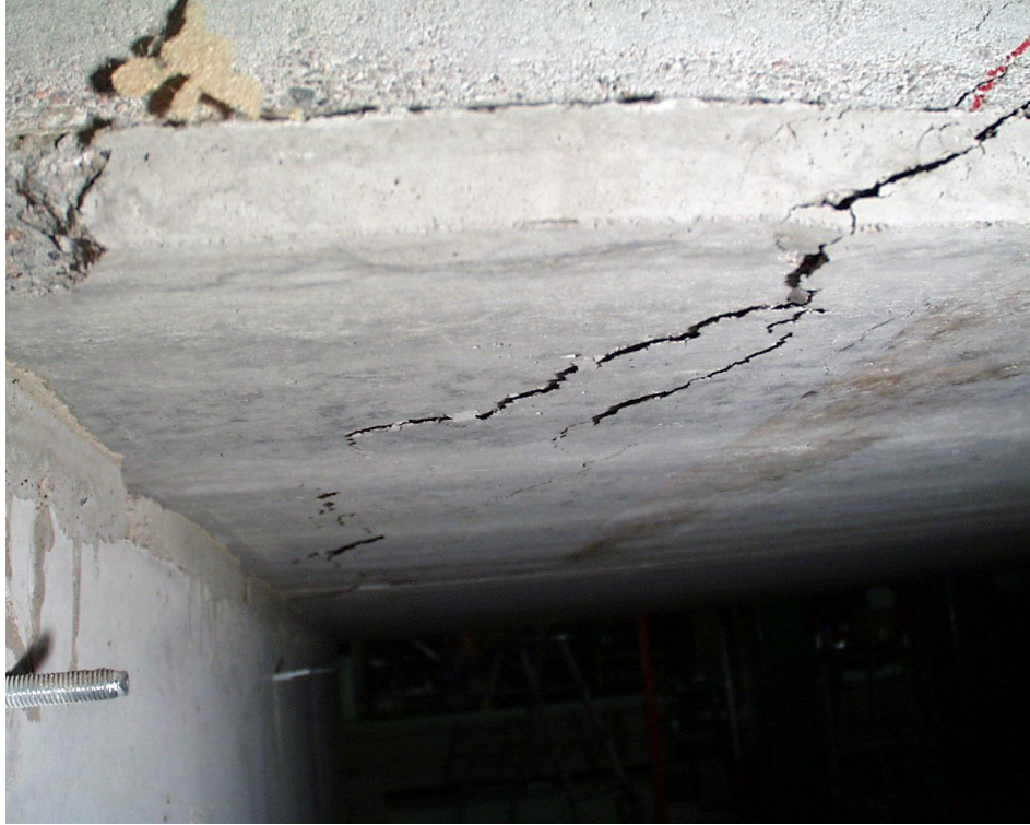
Fig. 31. PF400:15. Soffit of slab 4 after failure.
