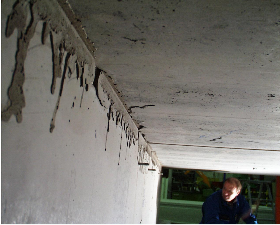
Fig. 13. PF400:13. Cracks in soffit of slab 3 after failure.
