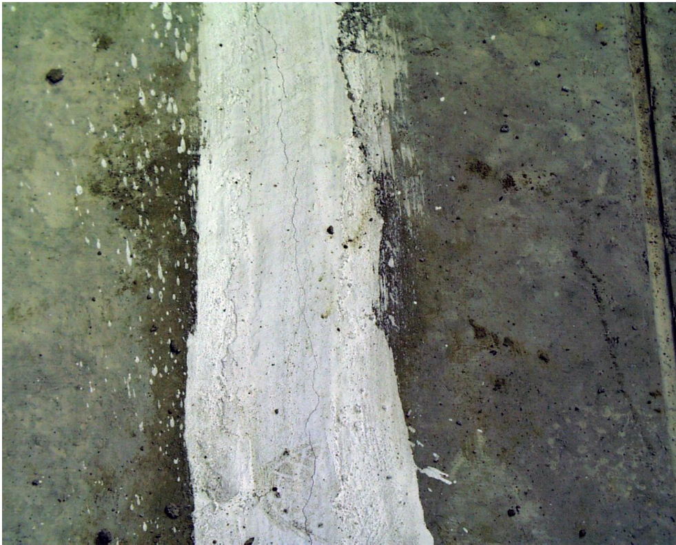
Fig. 4. Crack in joint due to wedging.
