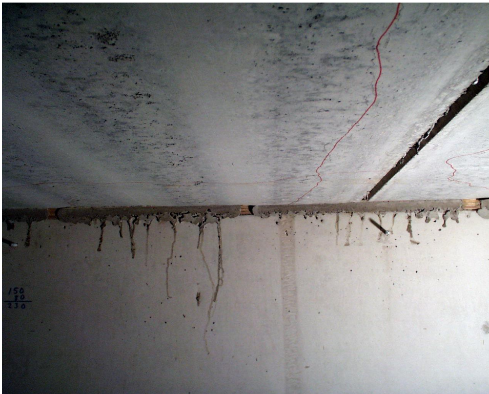
Fig. 24. PF400:14. Soffit after failure. Slab 2 on the left, slab 1 on the right.
