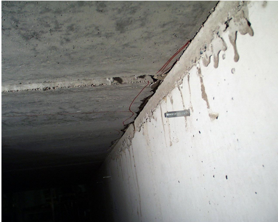
Fig. 25. PF400:14. Soffit after failure. Slab 1 in the front.
