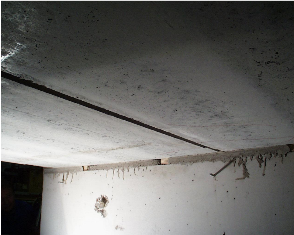
Fig. 33. PF400:15. Soffit of slabs 4 (on the left) and 3 after failure.
