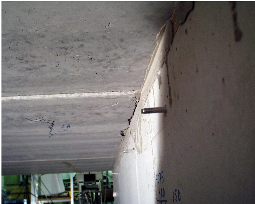
Fig. 12. PF400:13. Cracks in soffit of slab 3 after failure.
