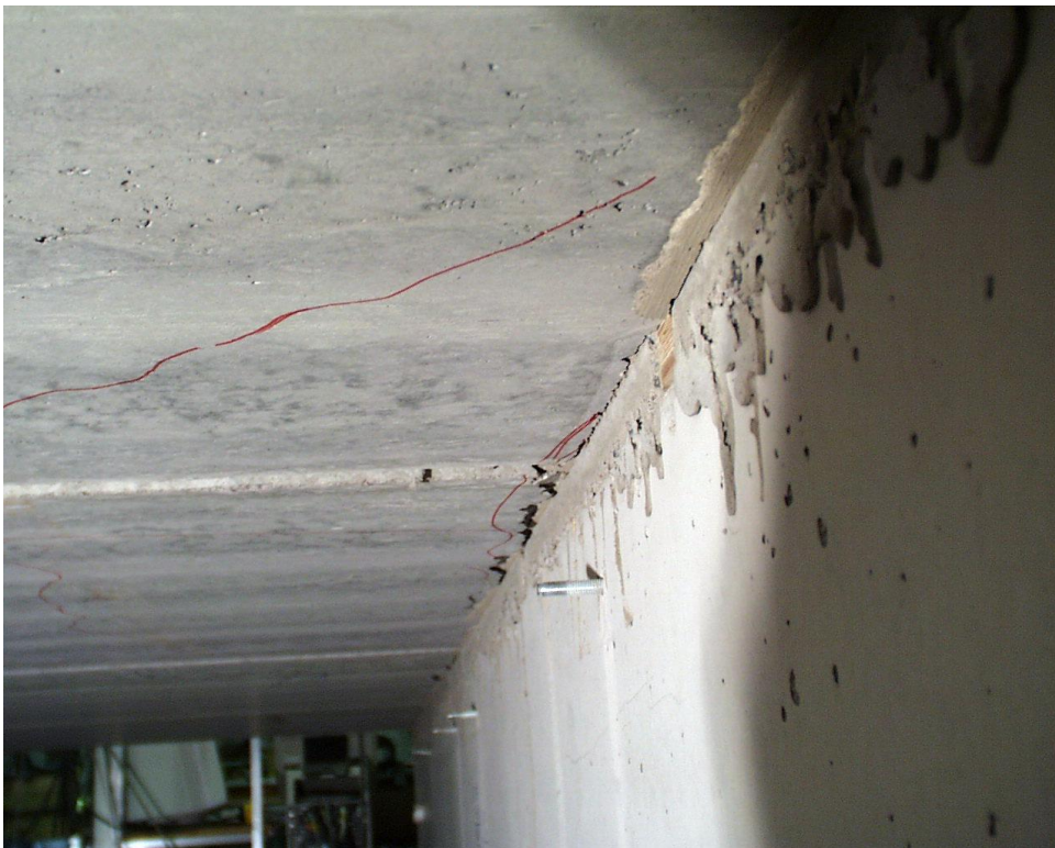
Fig. 22. PF400:14. Soffit after failure. Slab 1 in the front.
