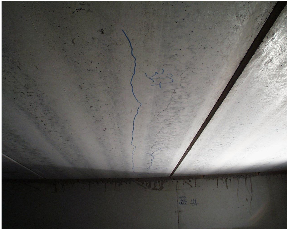
Fig. 14. PF400:13. Longitudinal cracks in soffit of slab 3 after failure.
