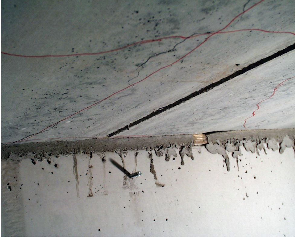
Fig. 23. PF400:14. Soffit after failure. Slab 2 on the left, slab 1 on the right.
