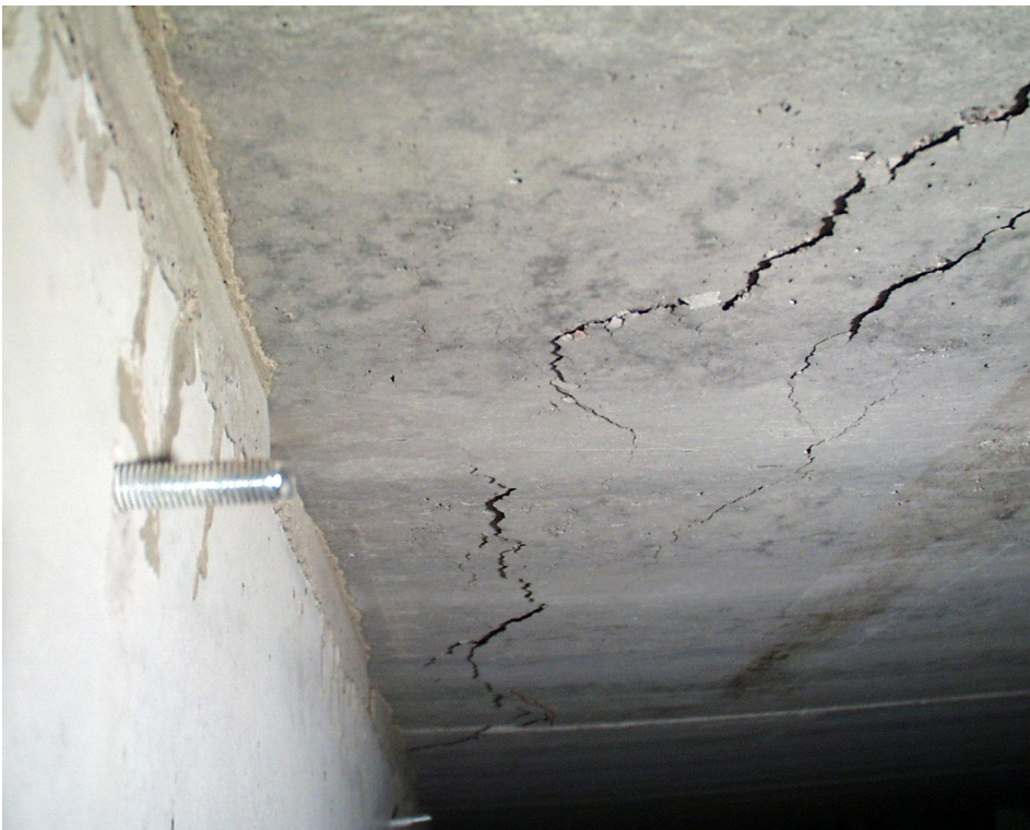
Fig. 32. PF400:15. Soffit of slabs 4 and 3 (in the rear) after failure.
