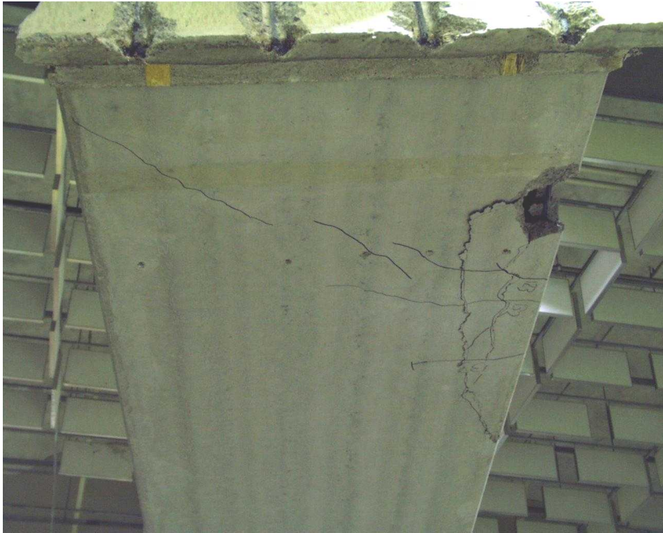
Fig. 59. ST200E2M. Cracking pattern after failure.
