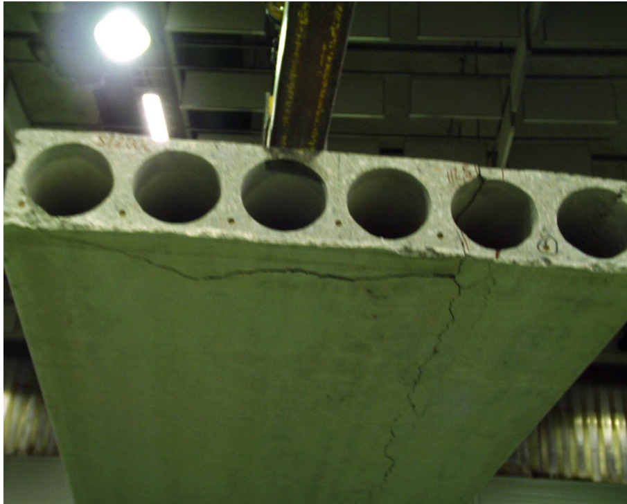
Fig. 9. ST200C. Cracking of soffit.
