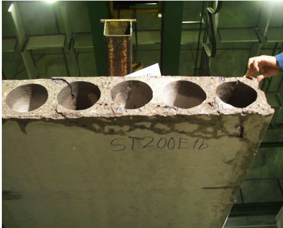
Fig. 17. ST200E1b. Cracking pattern in soffit.
