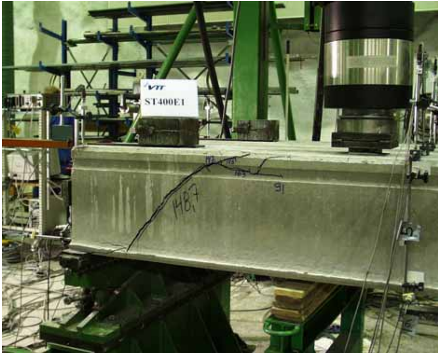
Fig. 17. ST400E1. Northern edge after failure.
