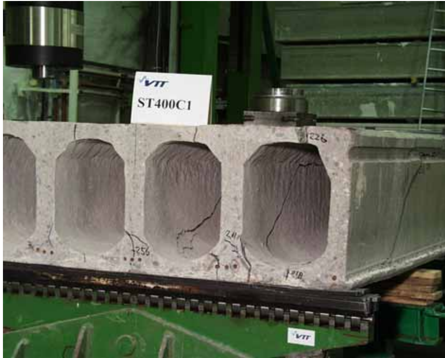
Fig. 3. ST400C1. Cracks in webs after failure.
