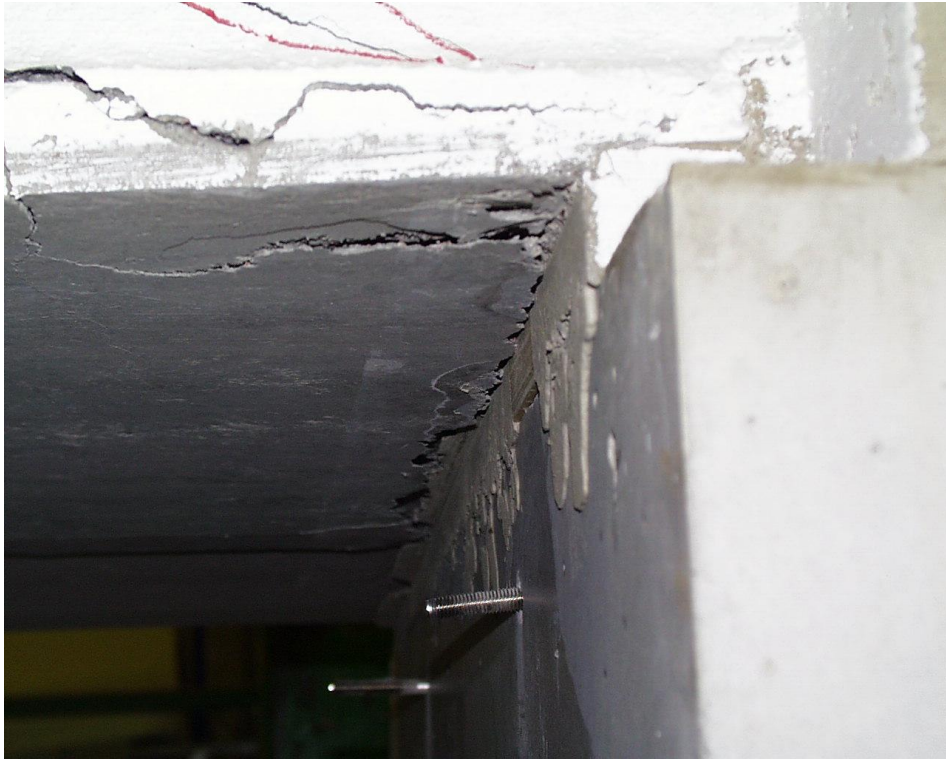
Fig. 47. ST200E1M. Transverse cracking of soffit next to support.
