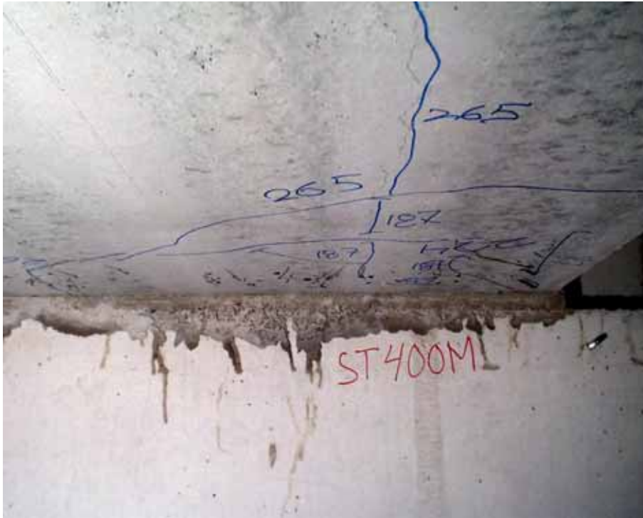
Fig. 41. ST400E1M. Cracking of soffit after unloading.
