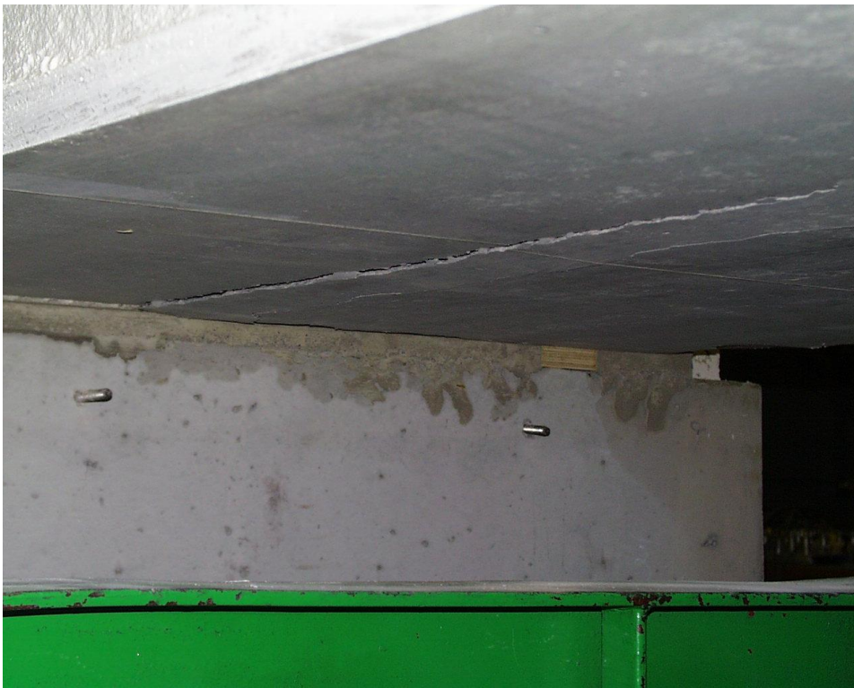
Fig. 46. ST200E1M. Soffit after failure.
