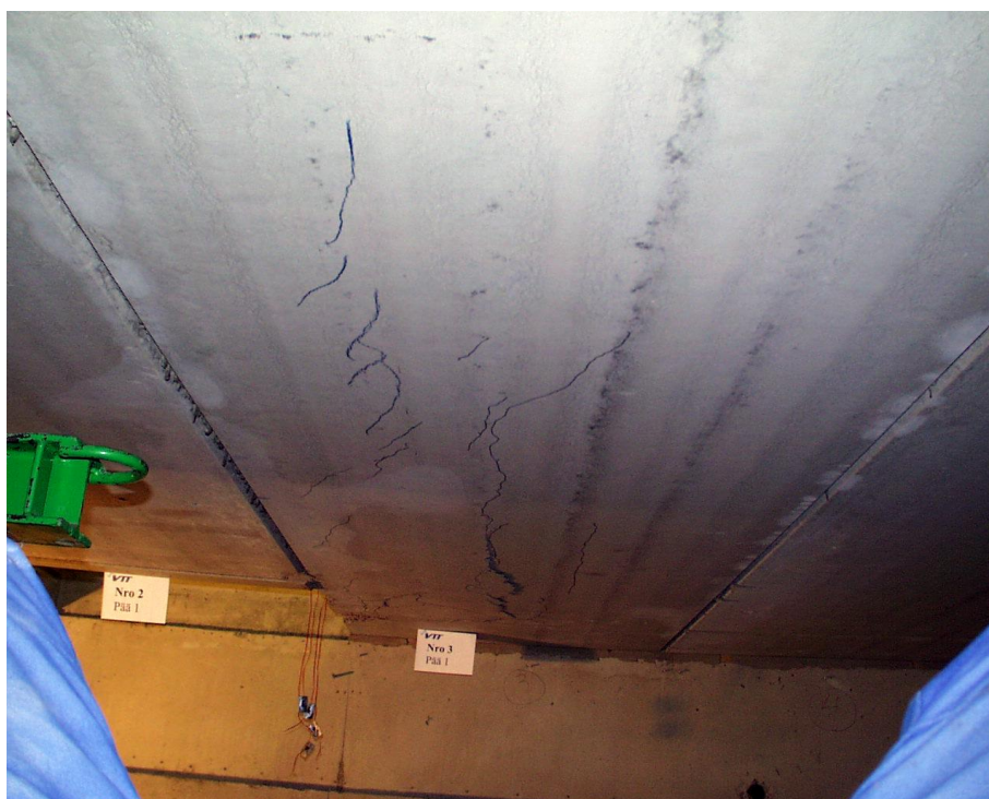
Fig. 32. FT200:12. Cracks on soffit of slab 3 after failure.
