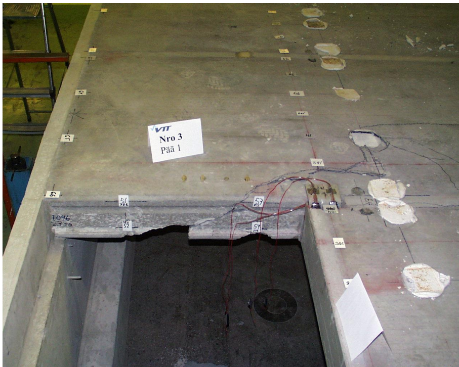
Fig. 28. FT200:12. Cracks on edge of slab 3 after failure.
