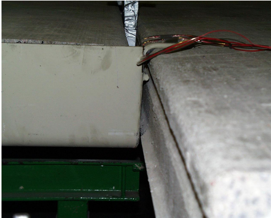
Fig. 3. Notching of slab to eliminate contact between trimmer beam and edge of slab.
