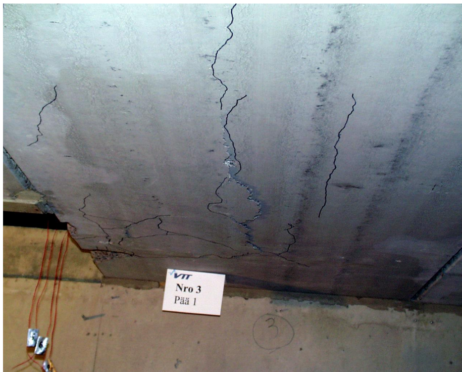
Fig. 31. FT200:12. Cracks on soffit of slab 3 after failure.
