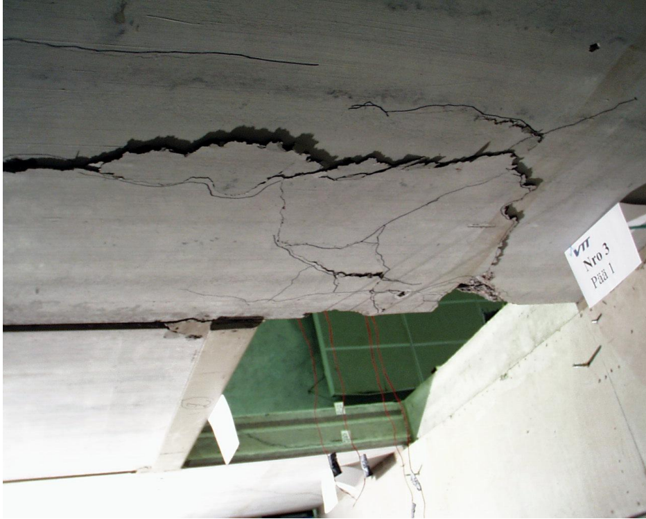
Fig. 33. FT200:12. Cracks on soffit of slab 3 after failure.
