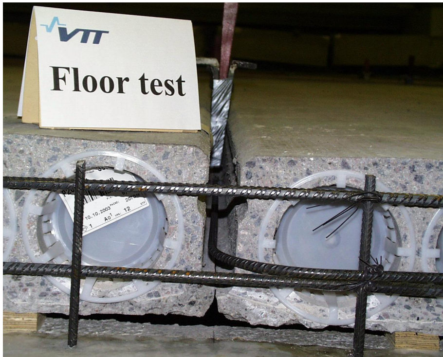
Fig. 5. Tie bar in longitudinal joint. Note also wrapped wedges in the joint used later for precracking of joint.
