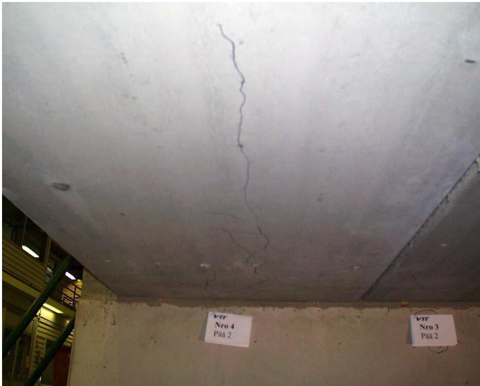
Fig. 34. FT200:11. Cracks on soffit of slab 4 after failure.
