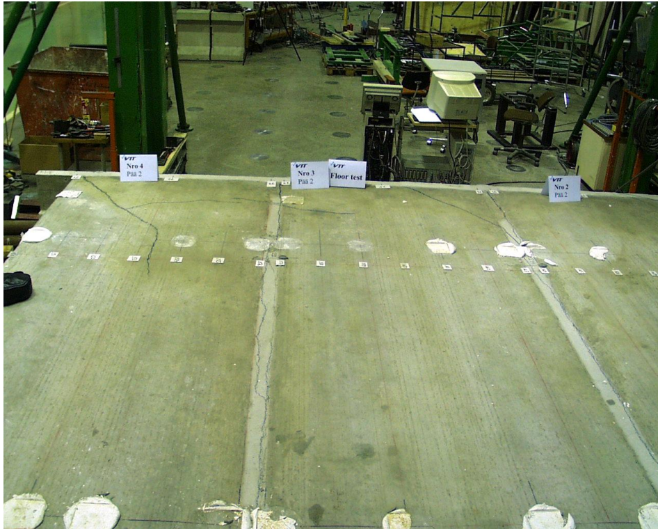
Fig. 17. FT200:11. Overview on cracks on top surface after failure. Slab 4 on the left.
