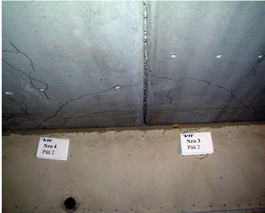
Fig. 35. FT200:11. Cracks on soffit of slabs 4 (on the left) and 3 after failure.
