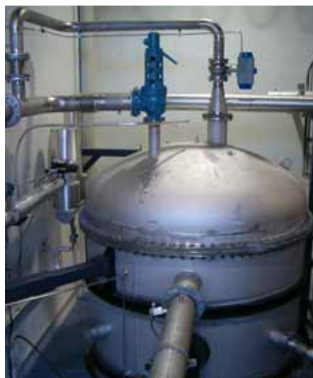
Figure 14.2.1. Dry well compartment of the PPOOLEX test facility.
