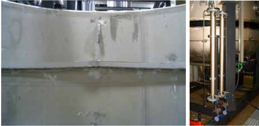
Figure 14.2.2. Drain gutters and condensate tanks for collecting condensate from dry well walls.
