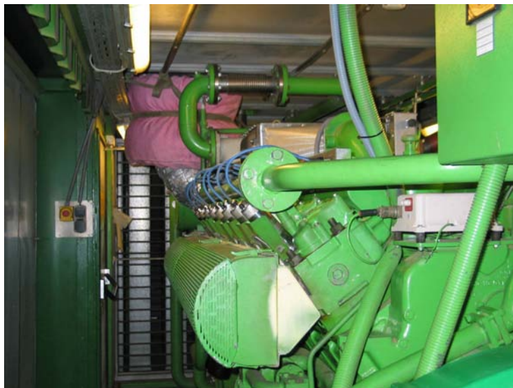
Figure 25. Biogas engine operating at the waste water treatment plant (site 4).
