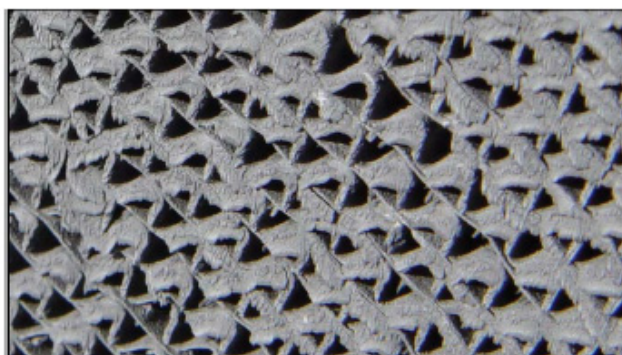
Figure 7. Silicate layers on a catalytic after-burner (Pierce 2005).
