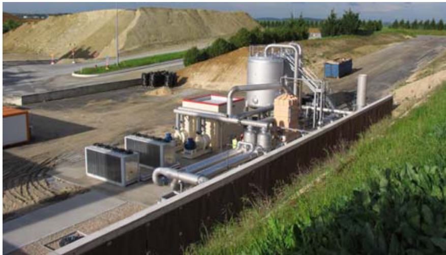
Figure 16. Claye-Souille siloxane removal equipment.
