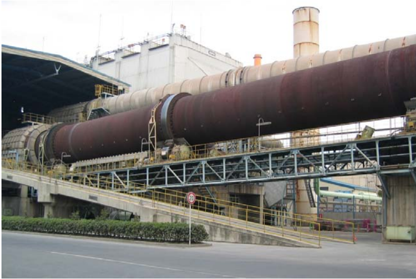
Figure 53. Rotary drums remain among the best available technologies in the process industry.
