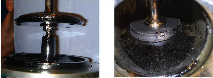
Figure 11. With tar blocked parts of the gas train.
