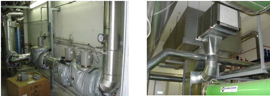
Figure 12. Adjusted gas train and preheated engine inlet air.
