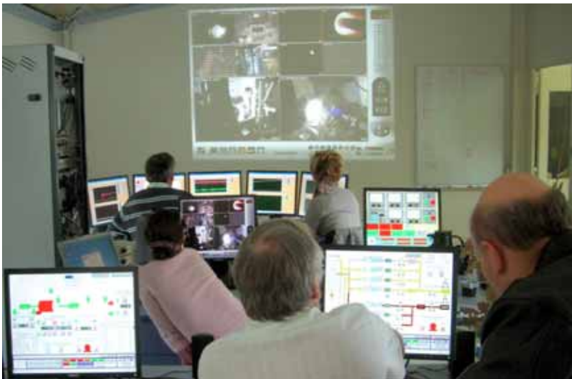
Figure 4. Control room of the VULCANO facility.
