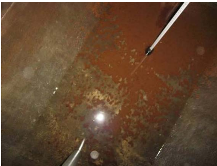
Figure 14.4. The inside of a 100 % HVO storage tank. The fuel is still completely clear after 8 months. The surface rust on the tank walls existed already before switching to HVO.
