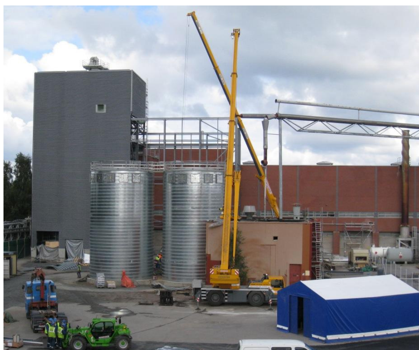
Figure 12. A photograph from the construction site of the NSE Biofuels demonstration facility at Varkaus.
