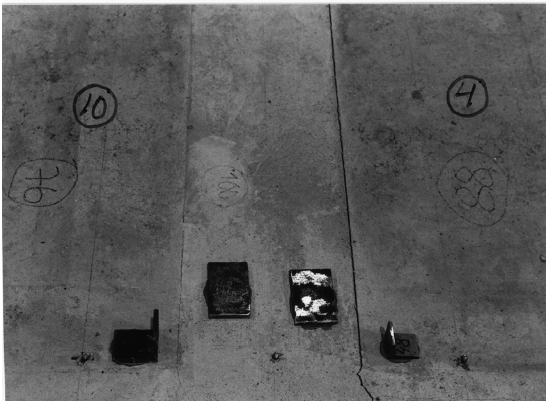
Fig. 14. Cracks between the slab ends and joint concrete.
