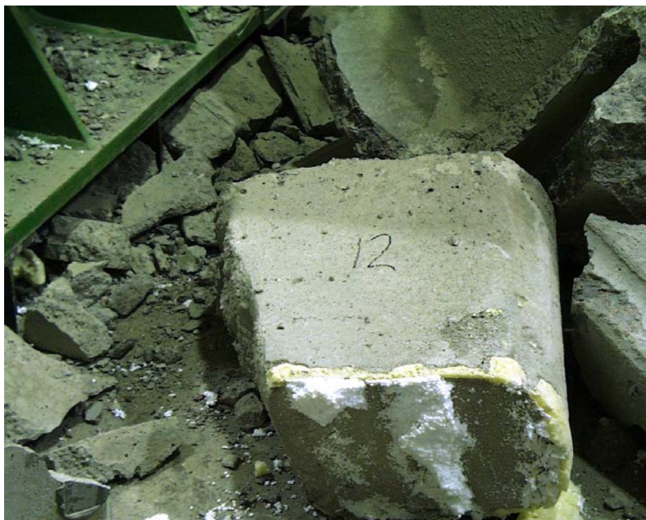
Fig. 49. Concrete filling taken from one core of slab 12.
