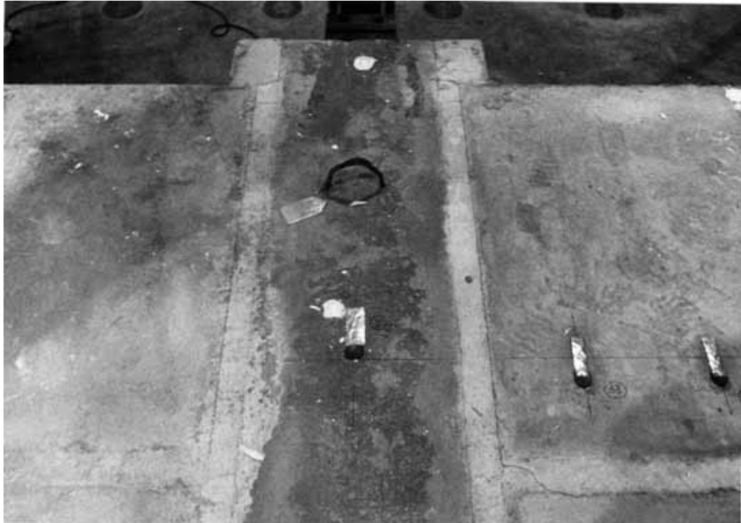
Fig. 20. Cracks parallel to beam in joint concrete. North end of middle beam.
