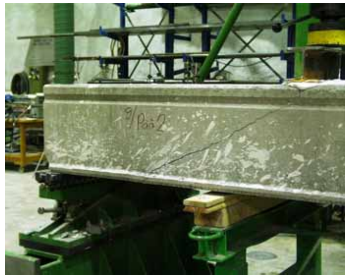
Fig. 30. Reference test R2. Northern side of slab after failure.
