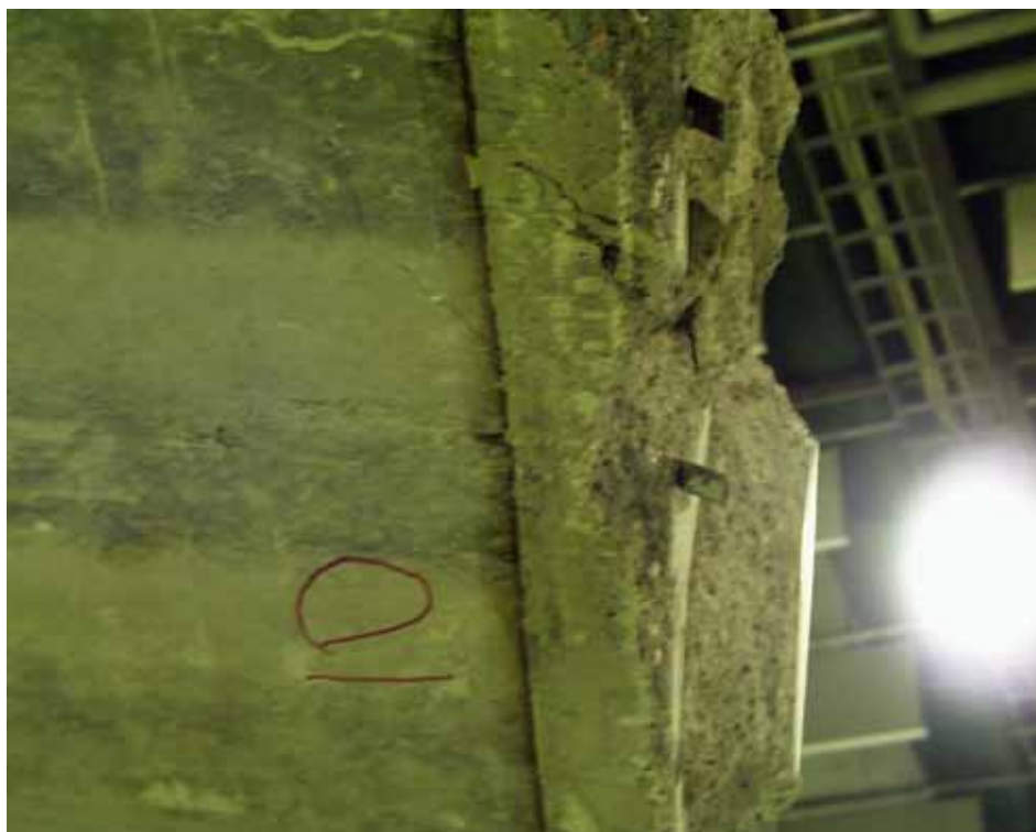
Fig. 27. Cast-in-situ concrete below slab end. Good bond with slab, weaker bond with beam.
