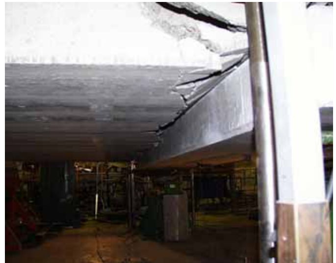
Fig. 14. Soffit of slabs 5-8 after failure.
