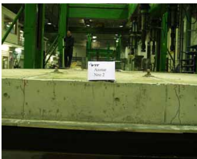
Fig. 29. Cracks in Western tie beam after failure. Slabs 2 and 3.
