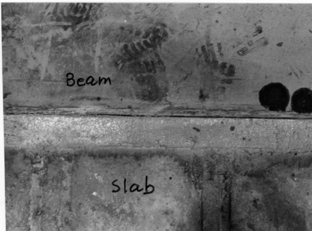
Fig. 6. Cracking of the joint concrete along the beam at stage 2.
