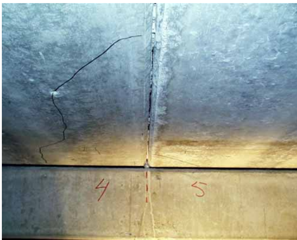
Fig. 20. Cracks in soffit of slabs 4 and 5 after failure.
