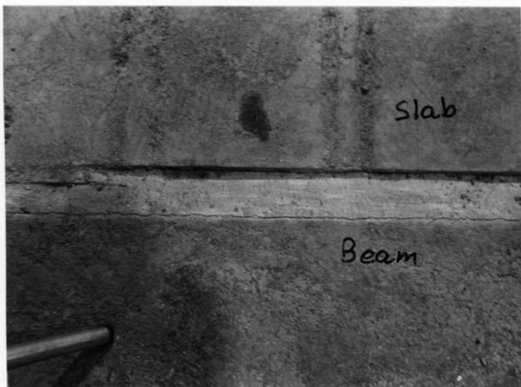
Fig. 13. Cracking of joint concrete along edge of middle beam.
