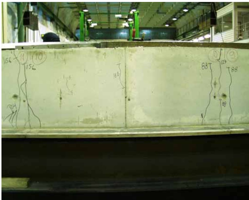
Fig. 33. Eastern end beam. Cracks in cast in-situ concrete at the end of slabs 9–11.
