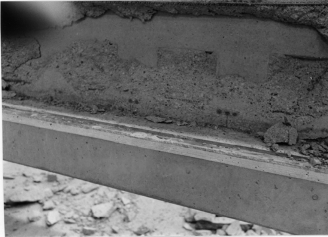
Fig. 11. Cracking of joint concrete along middle beam. Note the cracking of the shear keys.
