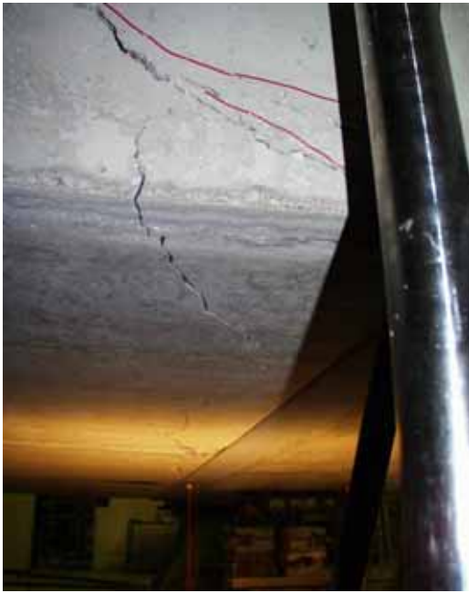
Fig. 21. Failed ends of slabs 3–4 after failure.
