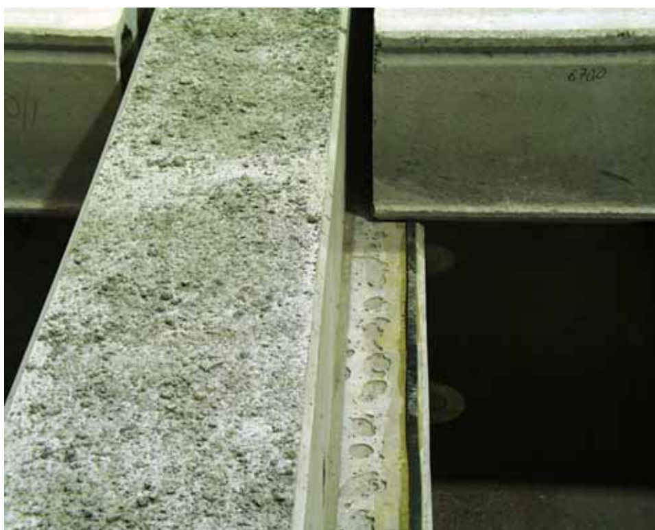
Fig. 4. Uneven surface of concrete beam due to air bubbles.
