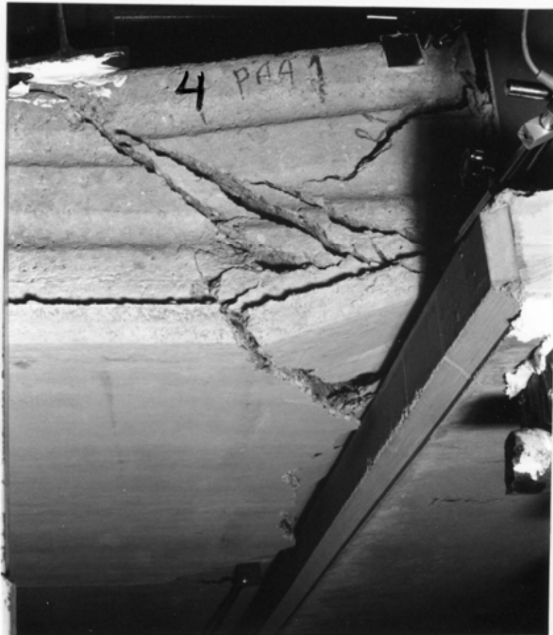
Fig. 9. Failure of slab unit no 4.
