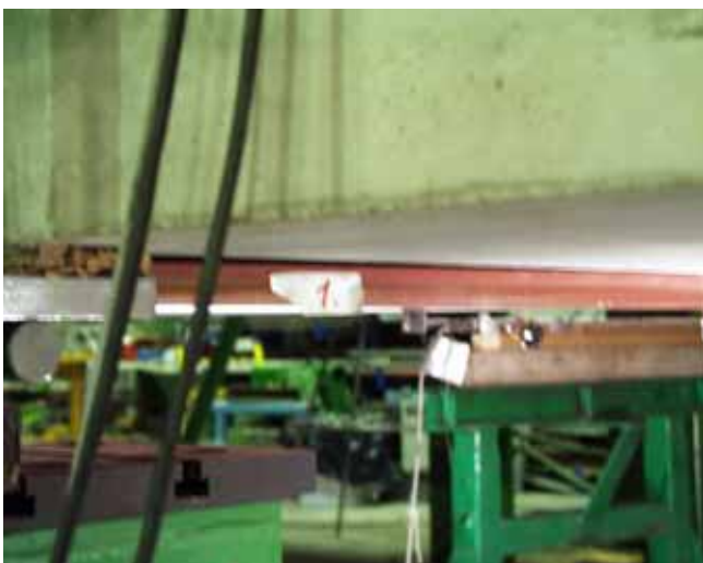
Fig. 17. Gap between soffit of slab 1 and bottom flange of middle beam.
