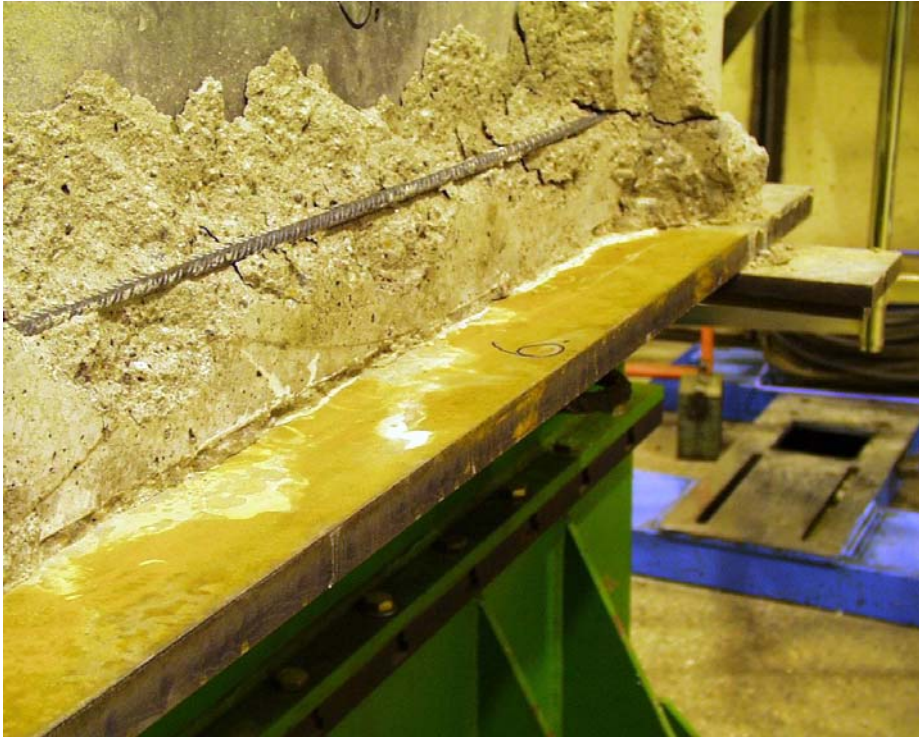
Fig. 55. Thin layers of grout as well as changes in colour on the flange below slab 1 due to the grout intruding into the gap between the soffit of the slab and the steel flange.
