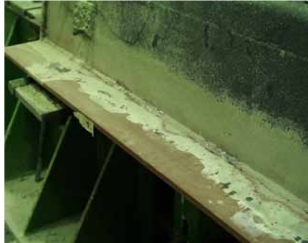
Fig. 44. A-beam after failure. Note the cement paste which has partly filled the gap between the soffit of slab 1 and the ledge of the beam.
