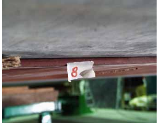
Fig. 20. Good contact between soffit of slab 8 and bottom flange of middle beam.
