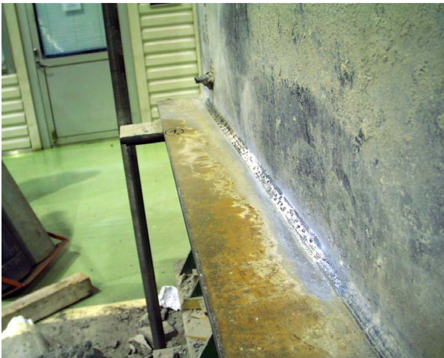
Fig. 54. Thin layers of grout as well as changes in colour on the flange below slab 1 due to the grout intruding into the gap between the soffit of the slab and the steel flange.
