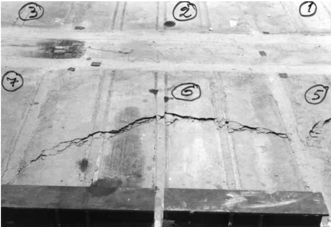
Fig. 19. Top surface of slab unit 6 after failure.
