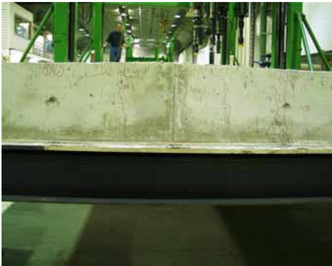
Fig. 15. Cracks in Western tie beam after failure. Slabs 1-3.
