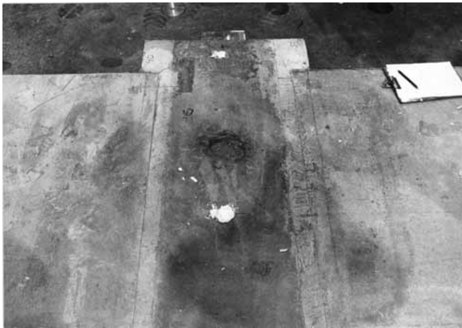
Fig. 15. Cracks parallel to beam. South end of middle beam.
