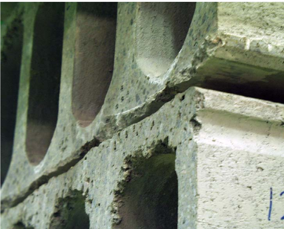
Fig. 52. Rough surface at slab end below even, saw-cut surface.
