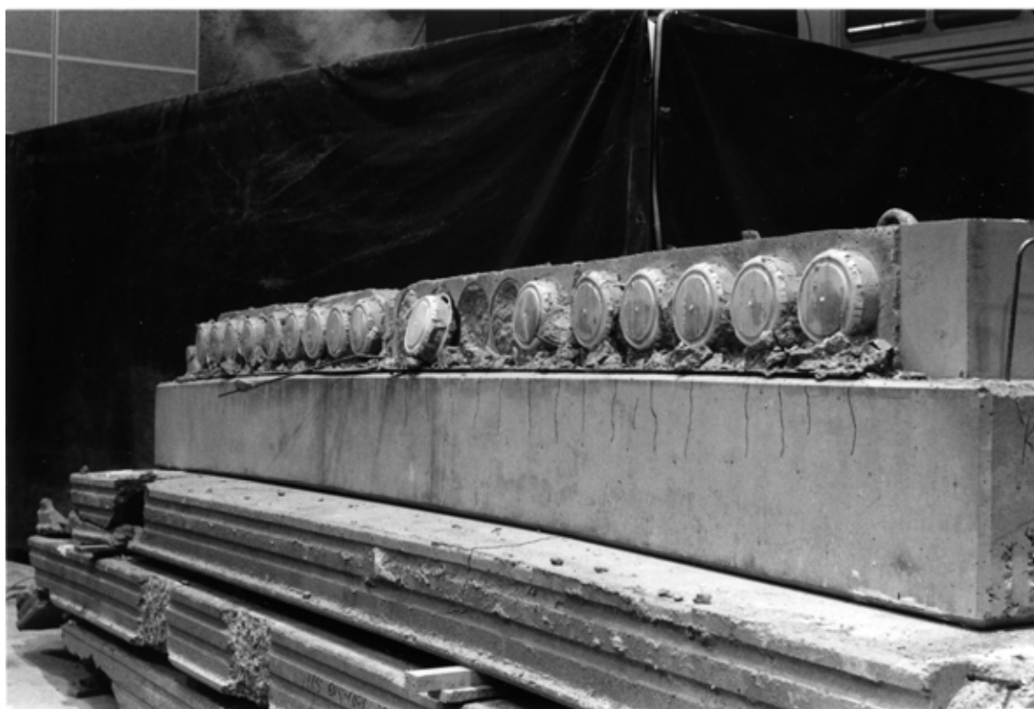
Fig. 12. The middle beam after the loading test, on the edge of the slab units no 1 - 4.
