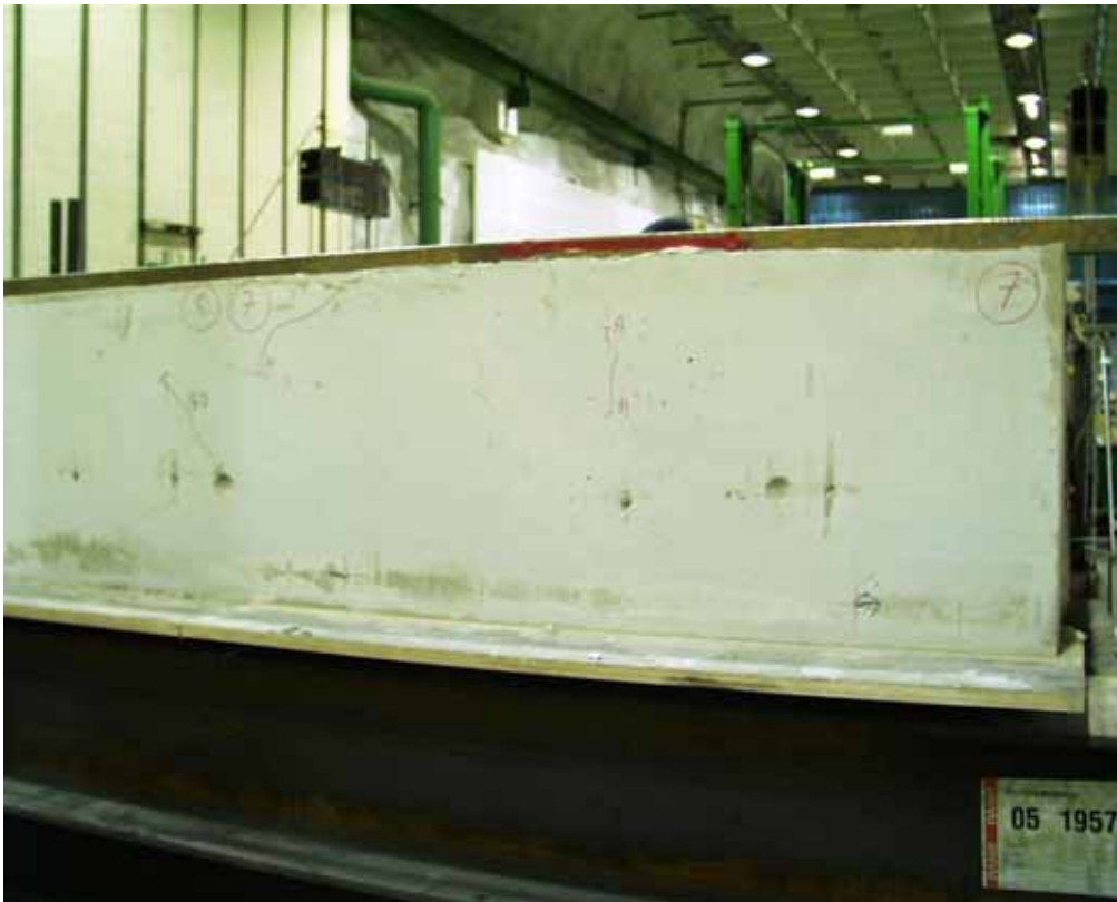
Fig. 31. Eastern end beam. Cracks in cast in-situ concrete at the end of slabs 7–8.
