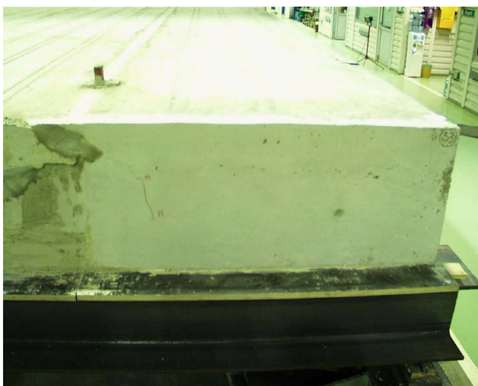
Fig. 34. Slab 7 after test. Cracks in tie beam. The red line and capital A indicate an initial crack.
