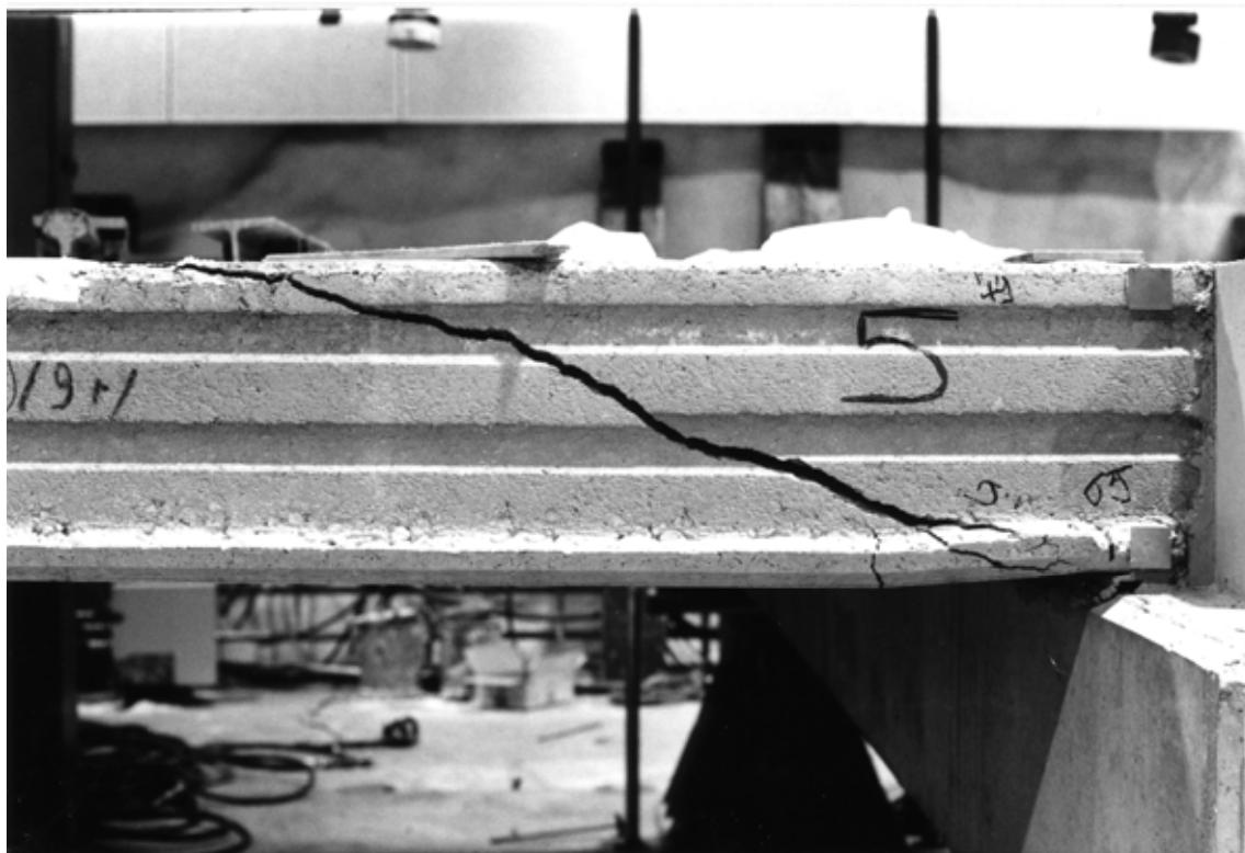
Fig. 8. The cracks in the longitudinal edge of the slab unit no 5, near the middle beam, at failure.
