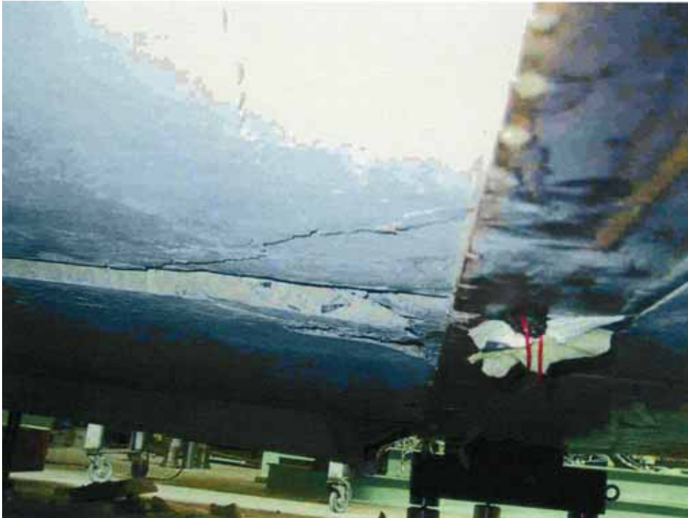
Fig. 5. Soffit after failure. Slab 6 in the front, slabs 7 and 8 in the rear.
