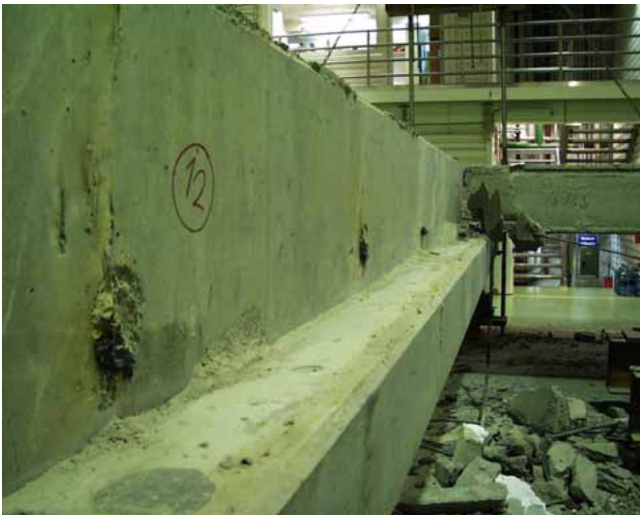
Fig. 30. Vertical cracking at slab ends took place along the web of the beam.
