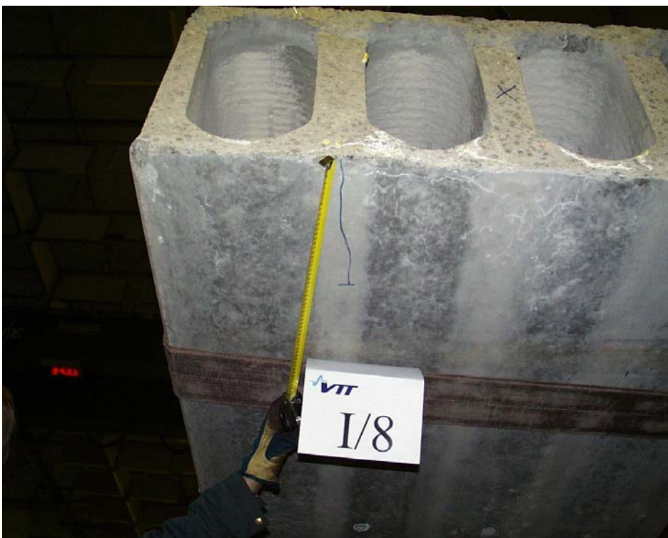
Fig. 8. Initial crack in slab 8.
