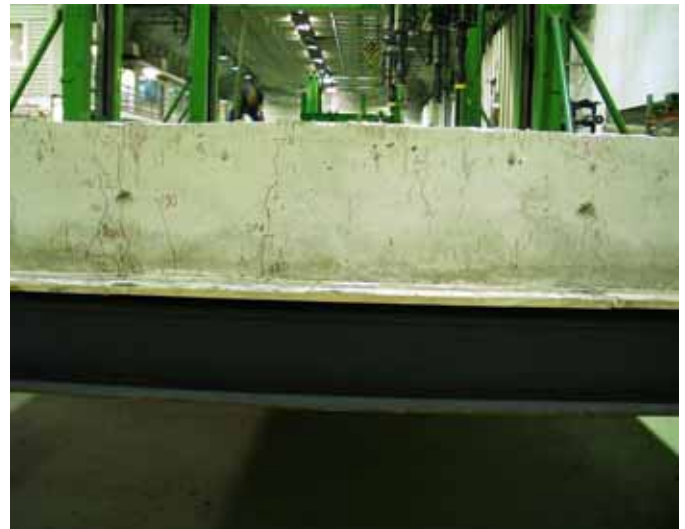
Fig. 16. Cracks in Western tie beam after failure. Slabs 2-4.
