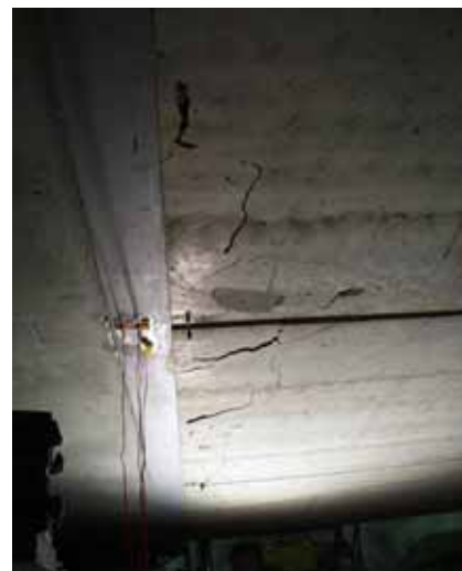
Fig. 16. Cracks in slabs 2-4 after failure.
