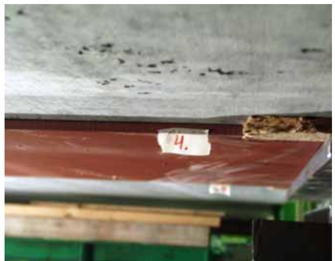
Fig. 18. Good contact between soffit of slab 4 and bottom flange of middle beam.
