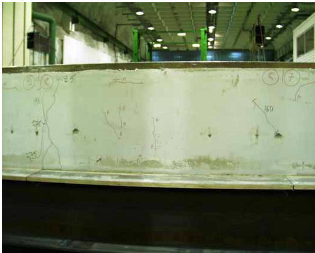
Fig. 30. Eastern end beam. Cracks in cast in-situ concrete at the end of slabs 7-9.
