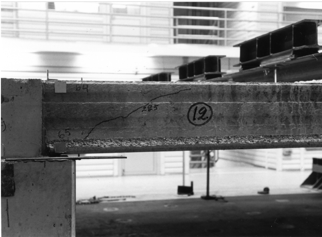
Fig. 11. Cracking pattern of slab unit No. 12 after failure of slab unit No. 7.
