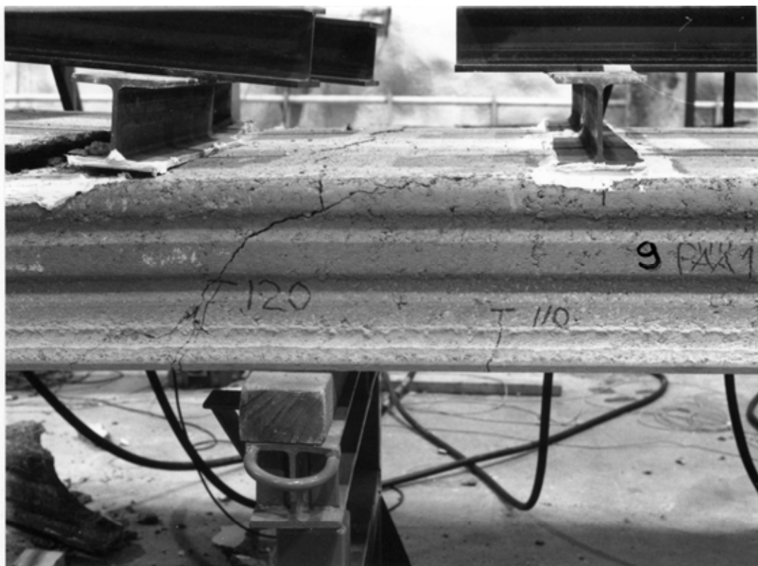
Fig. 26. Reference test R1 (photographed after the failure). The width of the diagonal crack in the figure was several millimetres before the failure took place to the left of the diagonal crack (see Figs 24 and 25).
