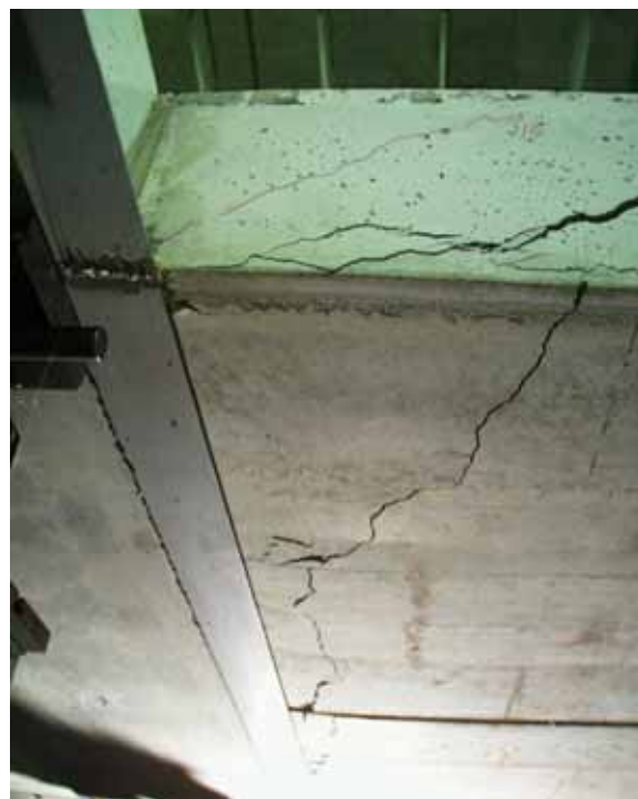
Fig. 20. Soffit of slabs 1-2 after failure.
