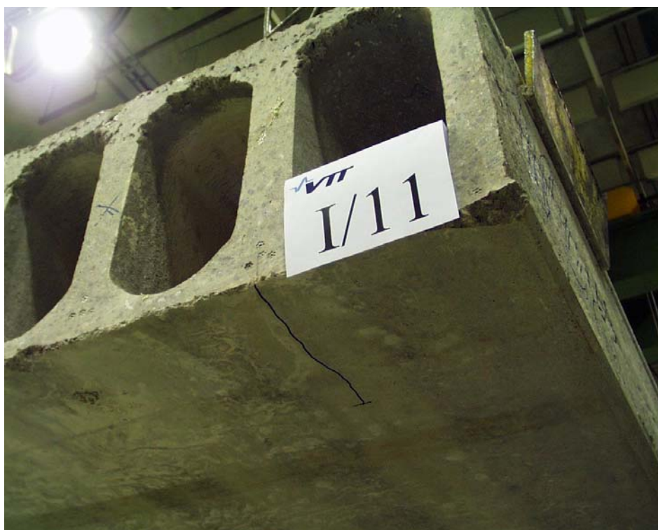
Fig. 10. Initial crack in slab 11.
