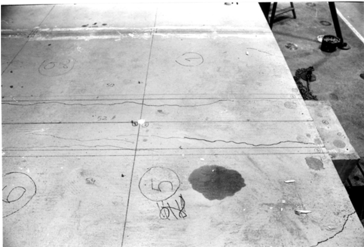
Fig. 14. The cracking of the concrete topping along the joint between the middle beam and the ends of the slab units no 1 - 2 and no 5 - 6.
