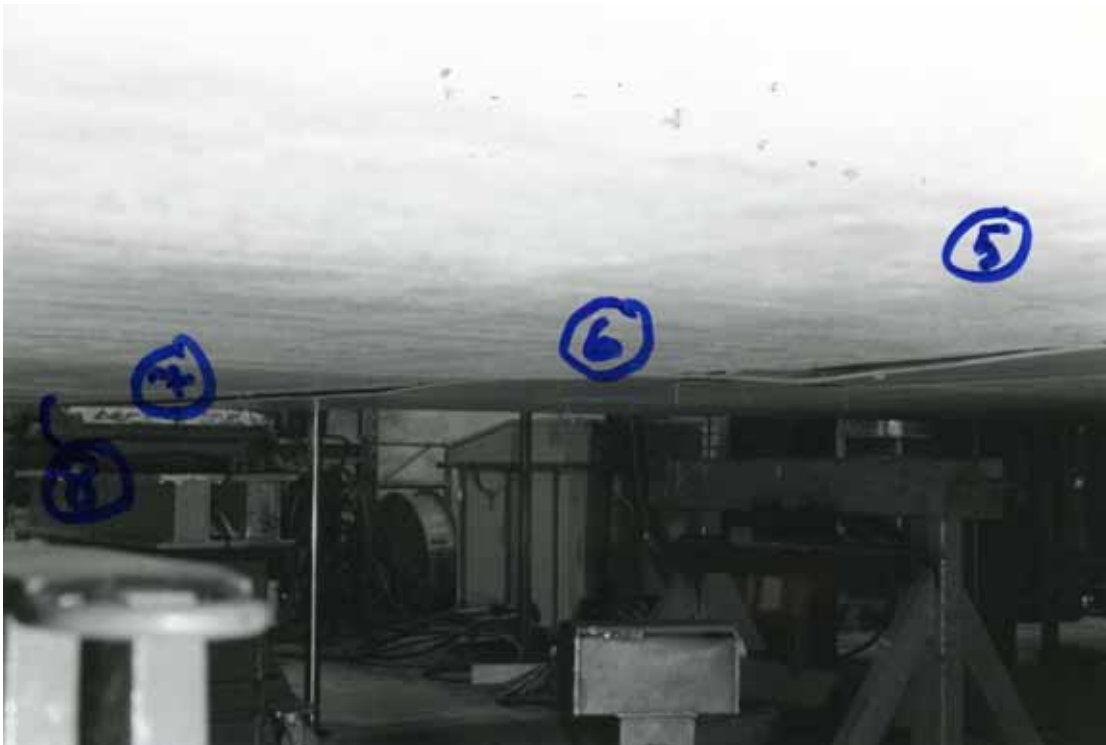
Fig. 15. Deformation of ledge of Delta-beam under slab units 5–8 after failure of the floor.
