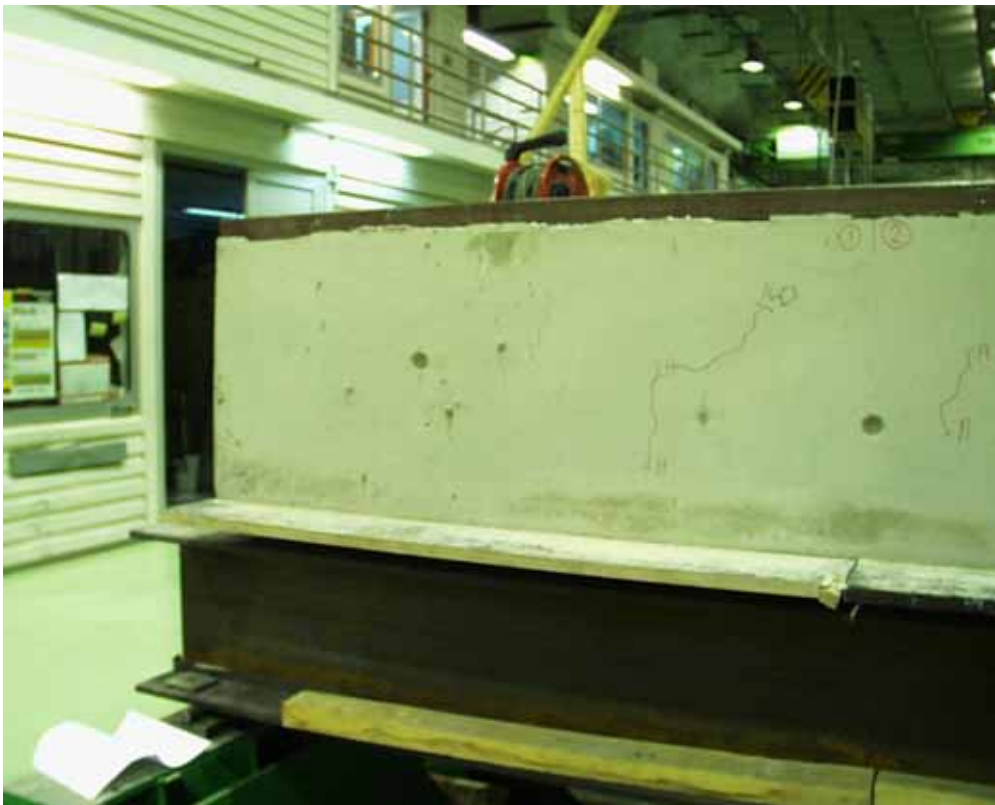
Fig. 24. Western end beam. Cracks in cast in-situ concrete at the end of slabs 1 and 2.
