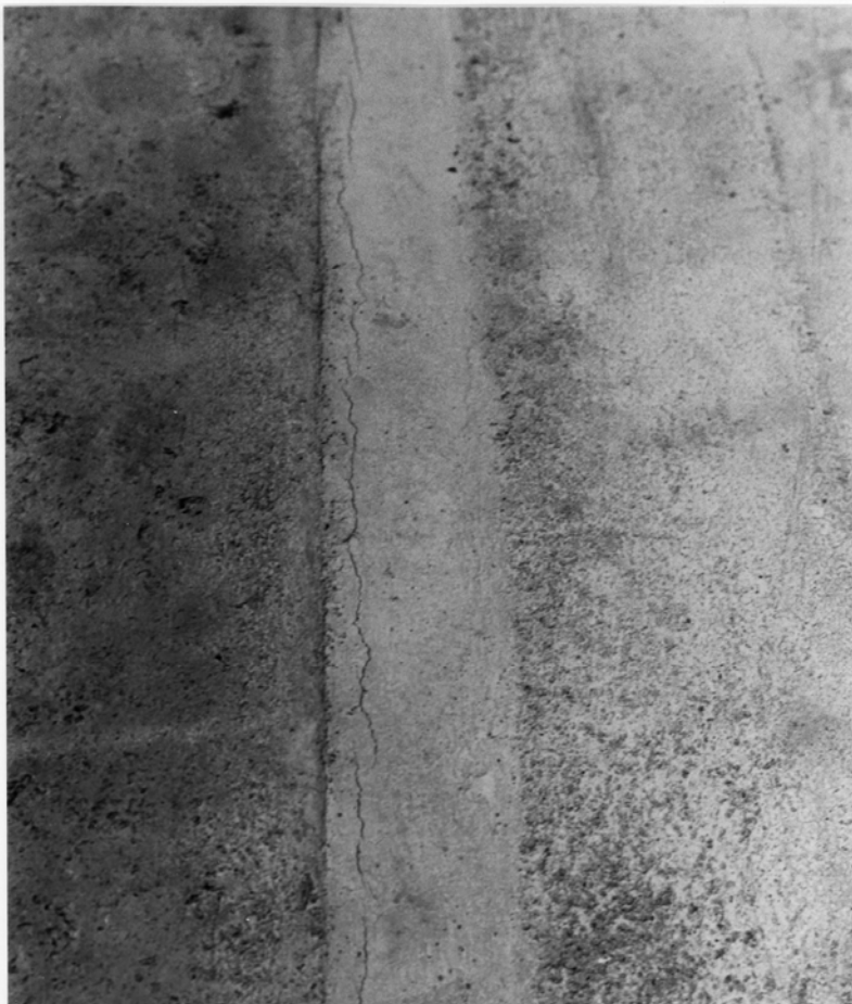
Fig. 16. Cracking along joint between adjacent slab units.
