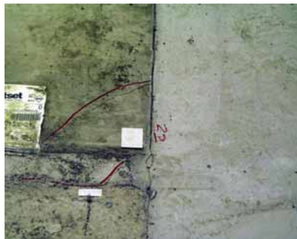
Fig. 18. Cracks in slab 1 after failure.
