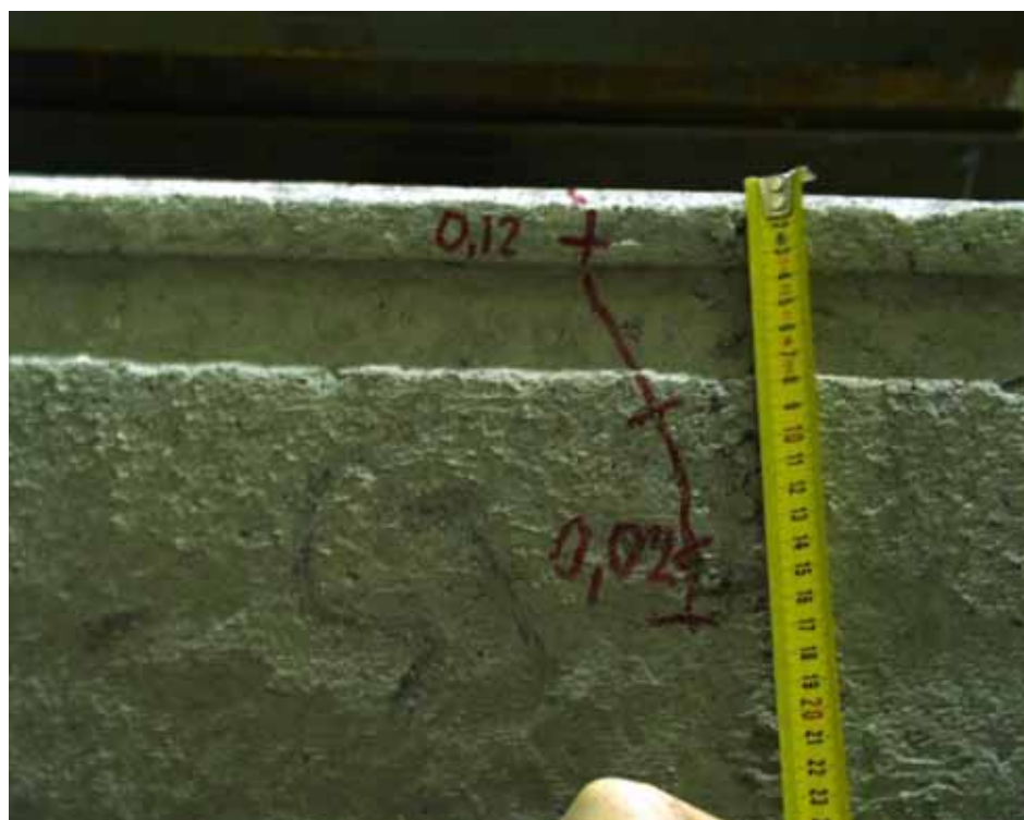
Fig. 12. Initial crack in slab 12.
