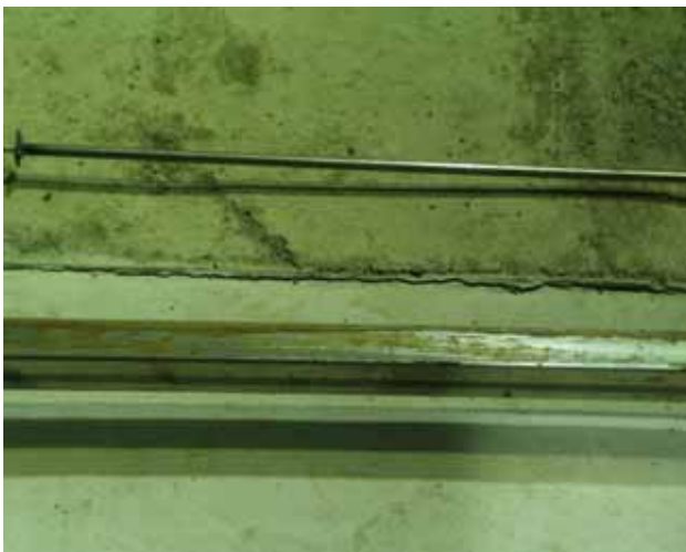
Fig. 13. Wide crack along the western edge of middle beam next to slab 2.
