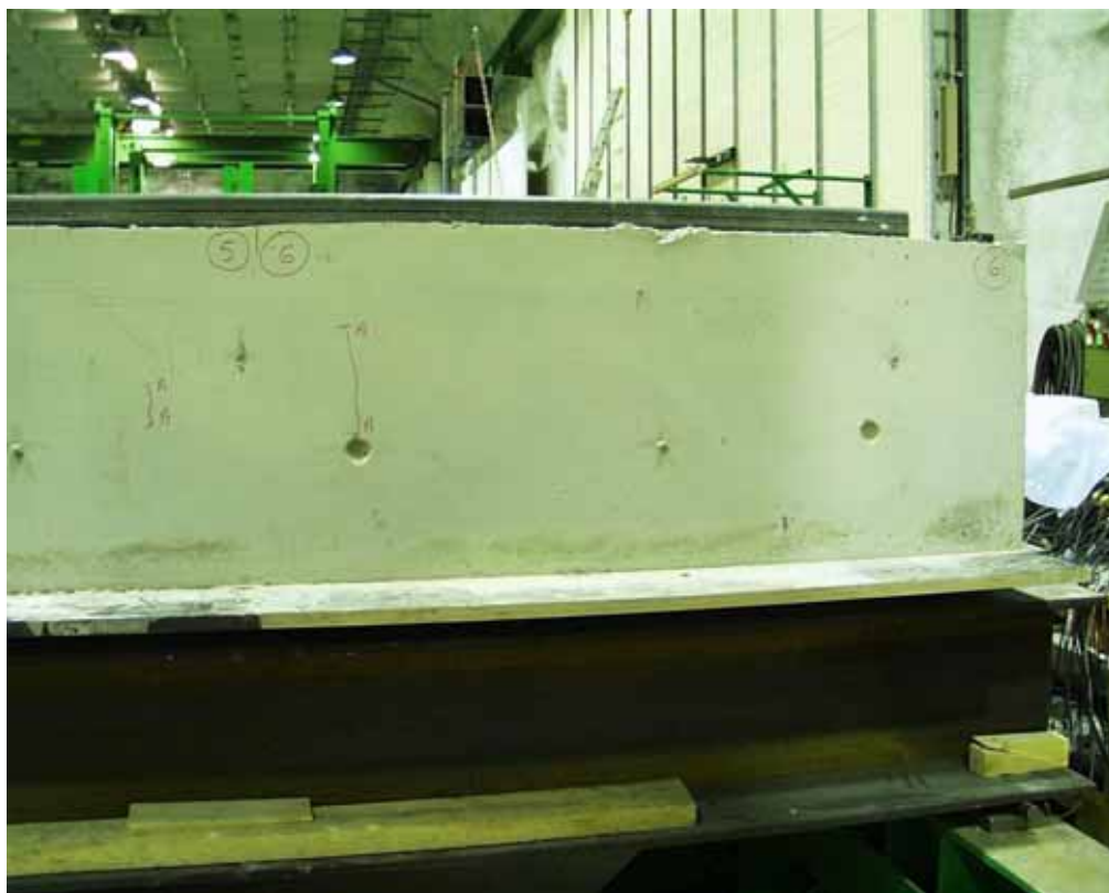
Fig. 29. Western end beam. Cracks in cast in-situ concrete at the end of slabs 5 and 6.
