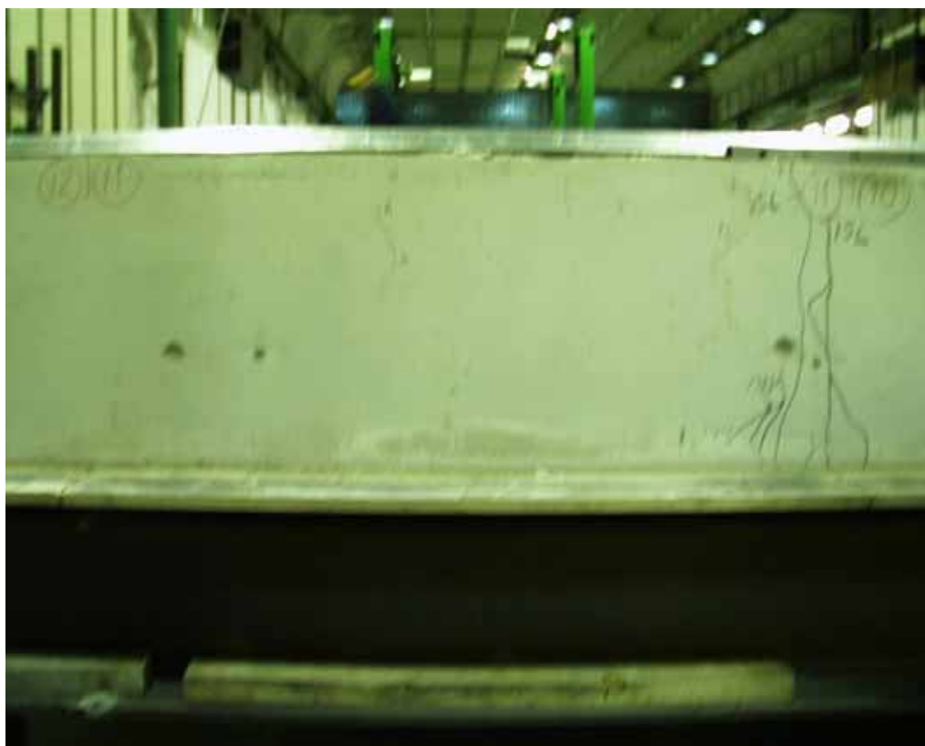
Fig. 34. Eastern end beam. Cracks in cast in-situ concrete at the end of slabs 10–12.
