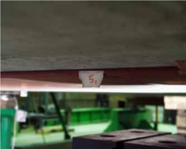
Fig. 19. Good contact between soffit of slab 5 and bottom flange of middle beam.
