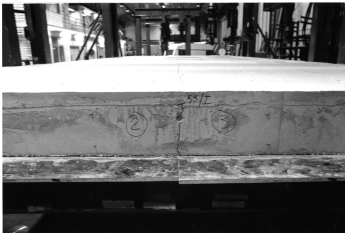
Fig. 8. A crack in the middle of the concrete tie beam, between the slab unit no 2 and 3.
