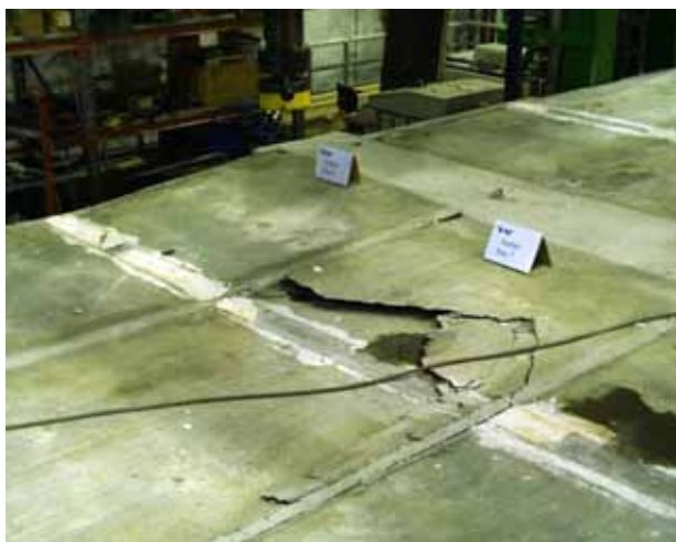
Fig. 39. Failed ends of slabs 7 and 8.
