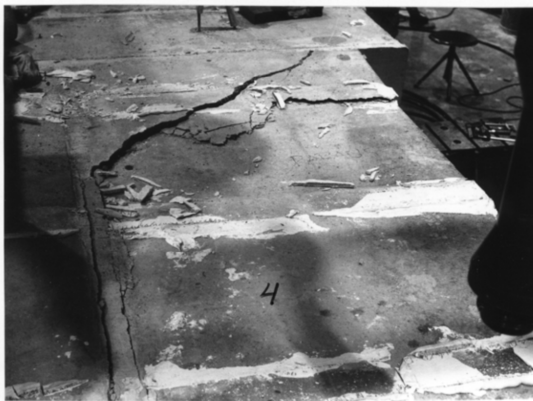
Fig. 12. Failure of slab unit no 4 seen from above.
