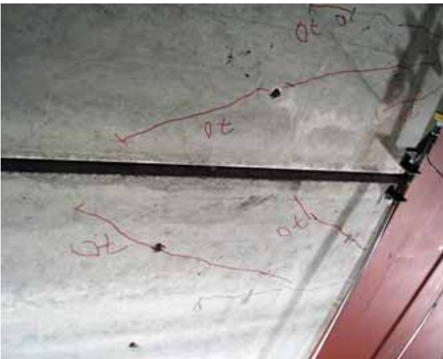
Fig. 21. Service load ( P_{a2} = 70 kN). Cracks below soffit of slabs 2 and 3.
