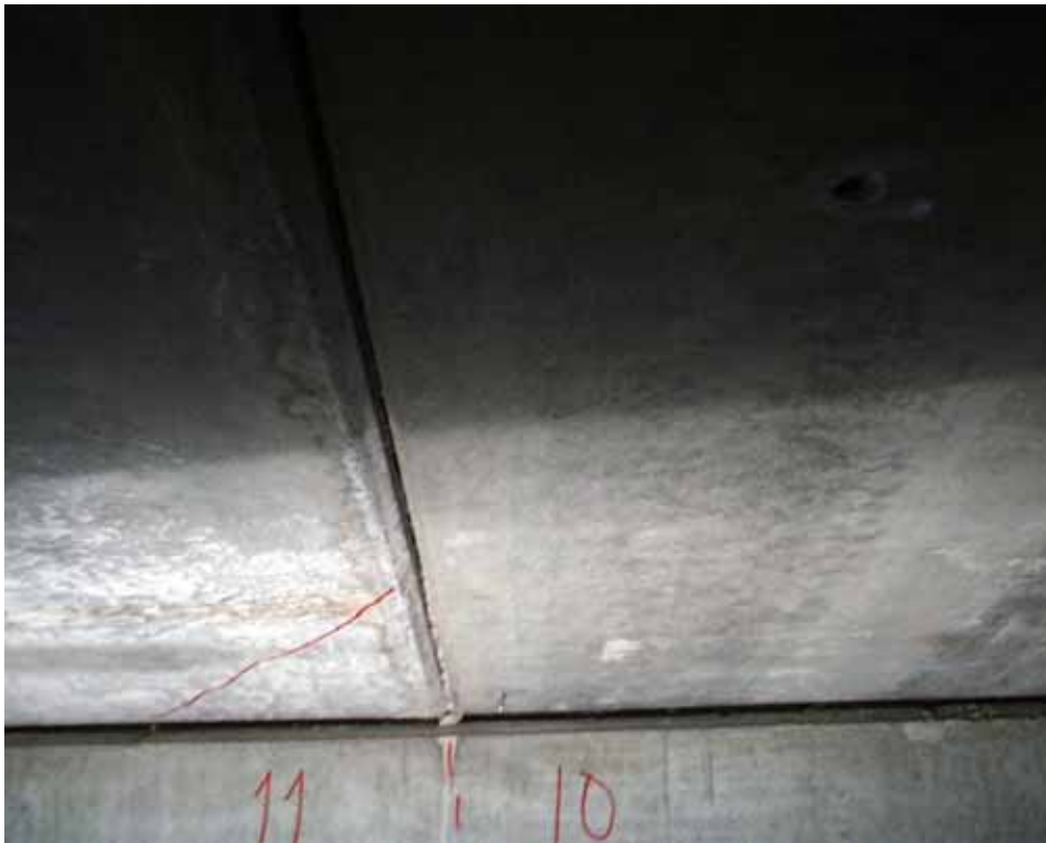
Fig. 21. Crack in soffit of slab 11 after failure.
