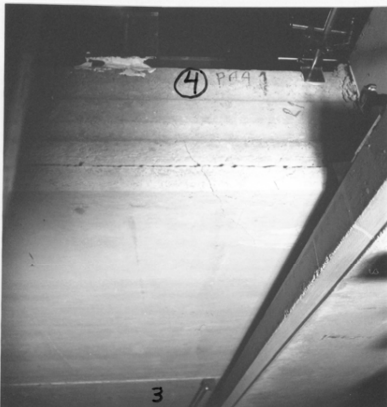
Fig. 6. Flexural cracking of slab unit no 4.
