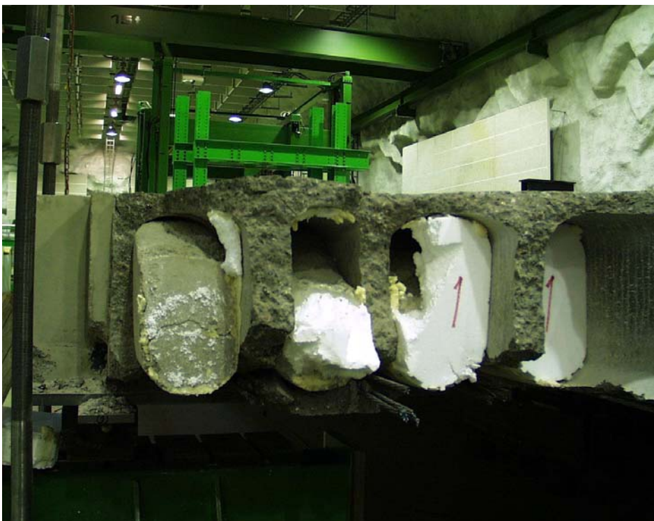
Fig. 48. Failure surface at end of slab 1. Note the incomplete filling of the cores.
