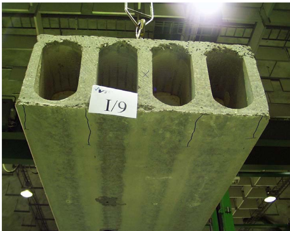
Fig. 9. Initial cracks in slab 9.
