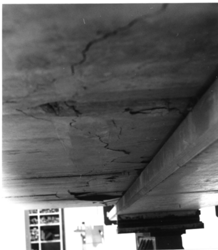
Fig. 10. Failure of slab units nos 1 - 4 seen from below.
