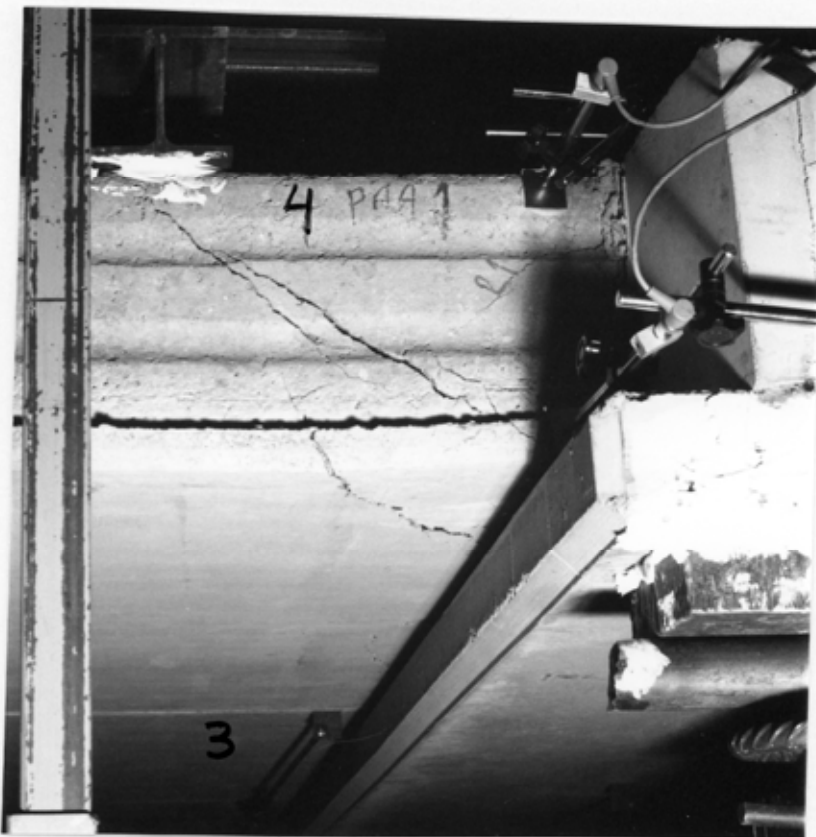
Fig. 8. Cracking pattern of slab unit no 4 before failure.
