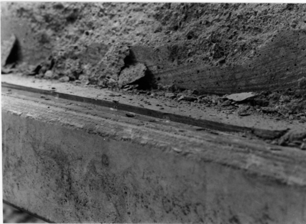
Fig. 12. Concrete filling between hollow core slab and ledger of middle beam. Note the perfect penetration of the concrete under the end of the slab.
