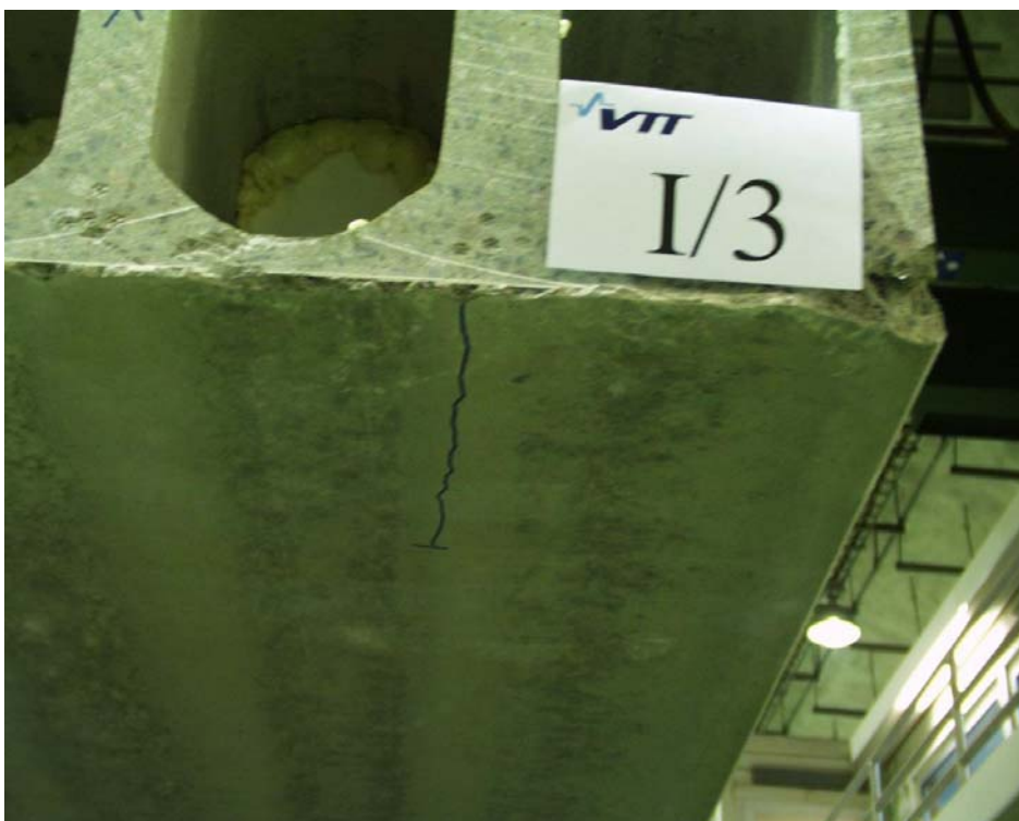
Fig. 4. Initial crack in slab 3.
