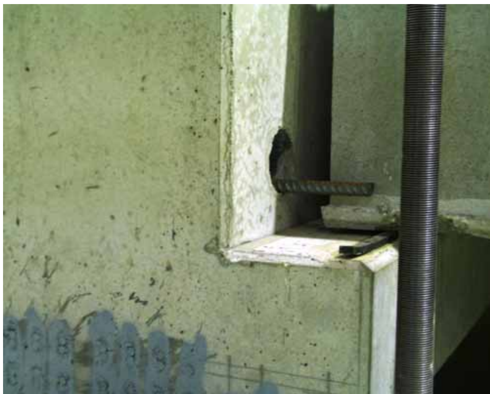
Fig. 9. A short tie bar through beam at support.
