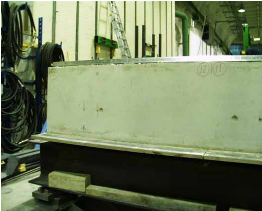
Fig. 35. Eastern end beam. No crack in cast in-situ concrete at the end of slab 12.
