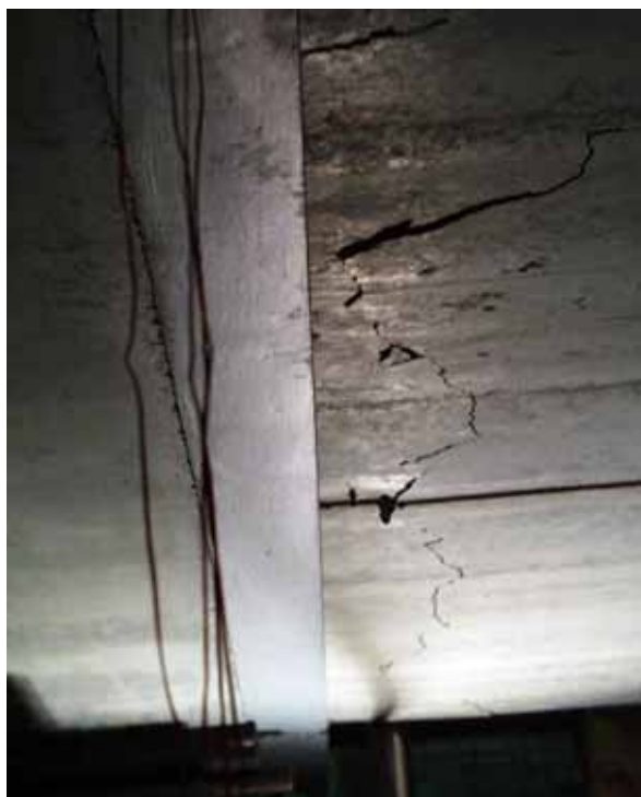
Fig. 19. Soffit of slabs 3 and 4 after failure.
