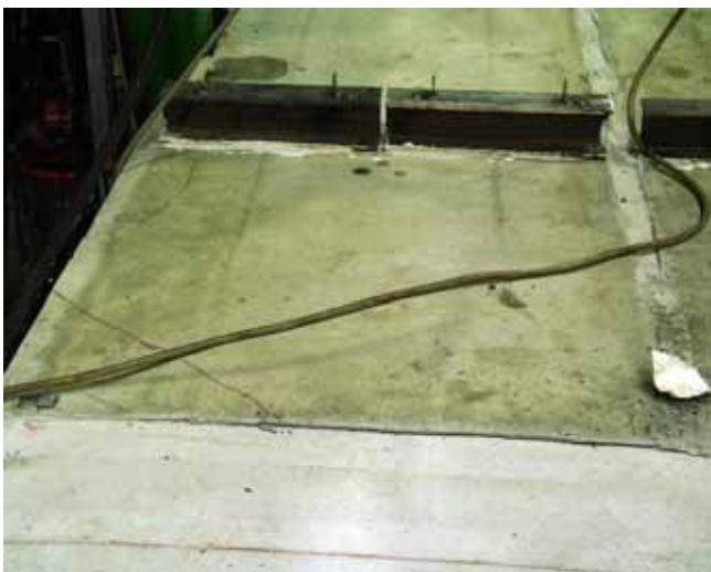
Fig. 15. Cracks in slab 4 after failure.
