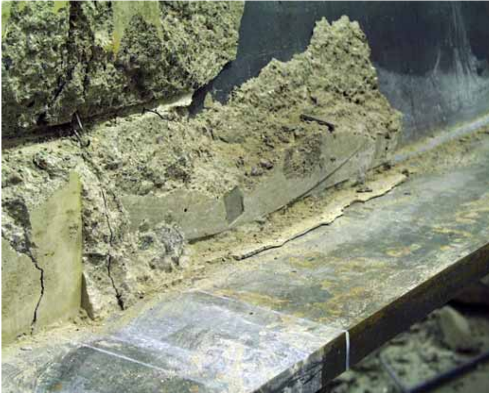
Fig. 23. Cast-in-situ concrete after removing the slabs. Note the grout layer between the slab and the flange of the beam.
