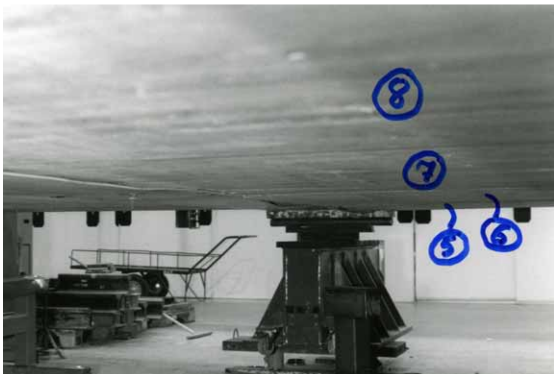
Fig. 14. Deformation of ledge of Delta-beam under slab units 5–8 after failure of the floor.
