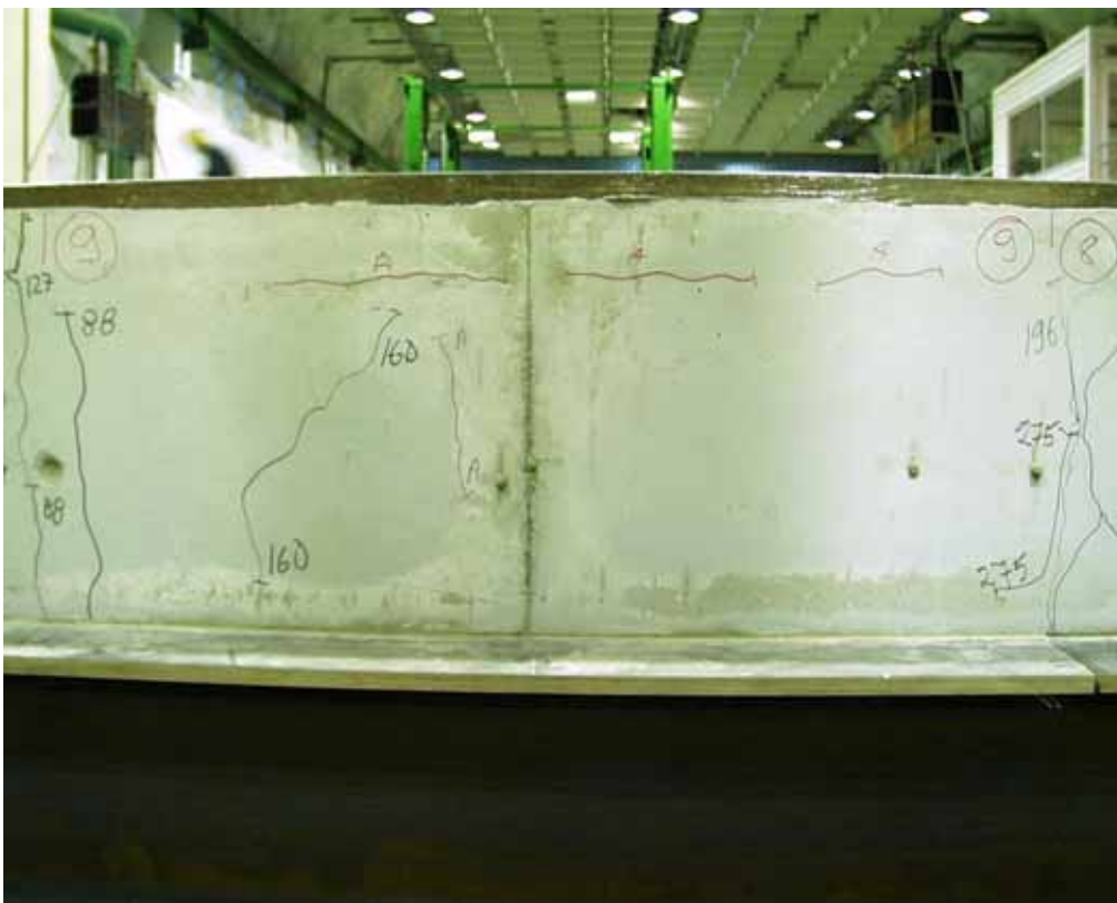
Fig. 32. Eastern end beam. Cracks in cast in-situ concrete at the end of slabs 8–9.
