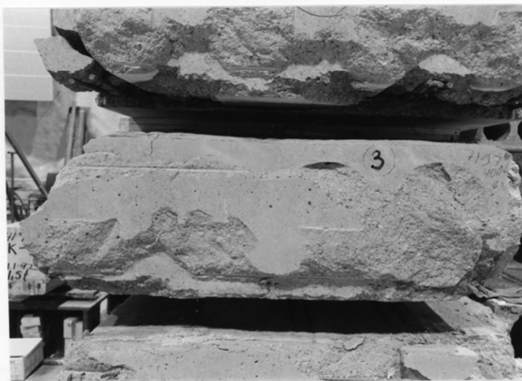
Fig. 10. End of slab unit no 3 after removal. Note the cracking of the shear keys.
