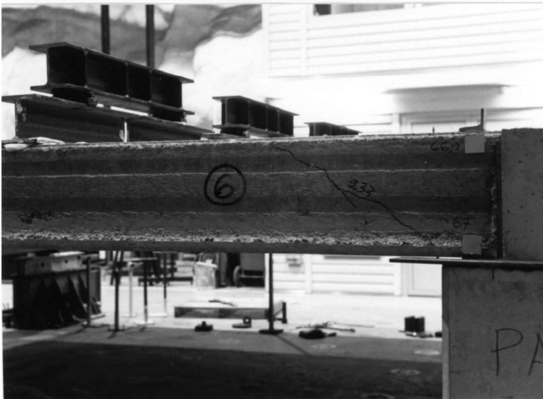
Fig. 12. Cracking pattern of slab unit No. 6 after failure of slab unit No. 7.
