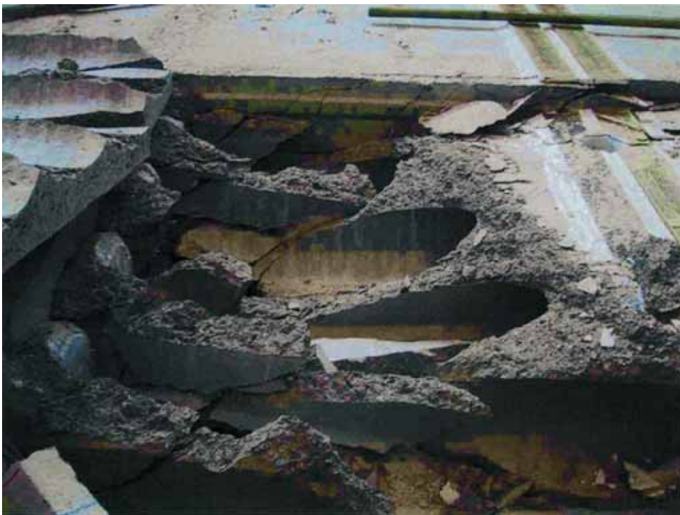
Fig. 6. Slab 8 after failure. The loose top part has been removed.
