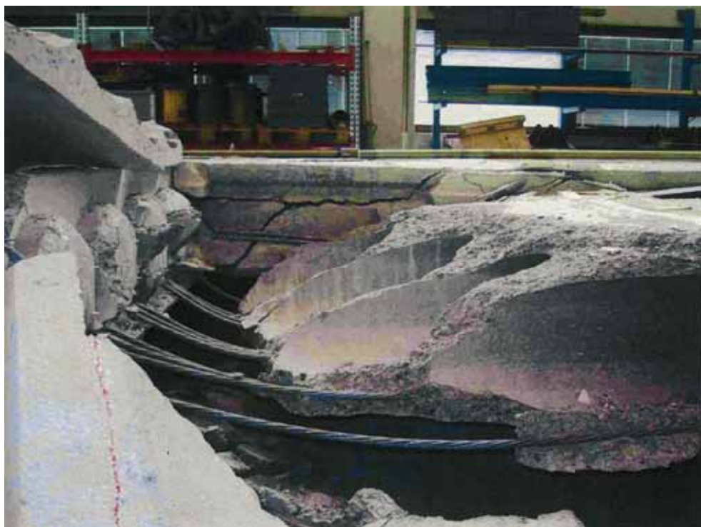
Fig. 7. Slab 8 after failure. All loose concrete material has been removed.
