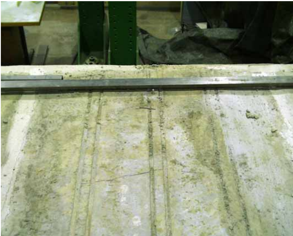
Fig. 15. Initial crack in slab 3 close to end beam.
