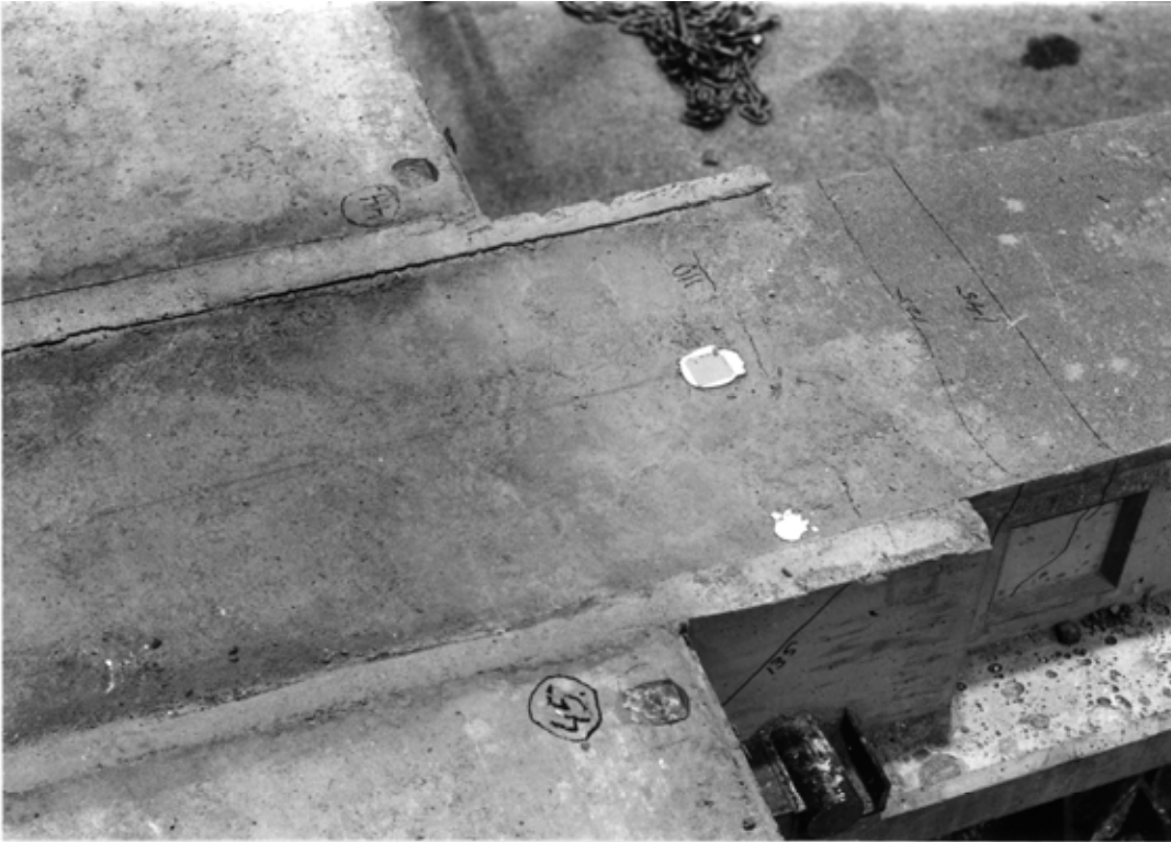
Fig. 11. Cracks in the middle beam and along the joint between the slab ends and the beam.
