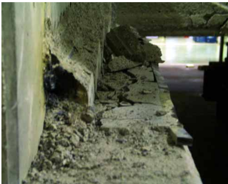
Fig. 24. Grout at support after removal of slab. Note the perfect filling of the gap below the slab end.
