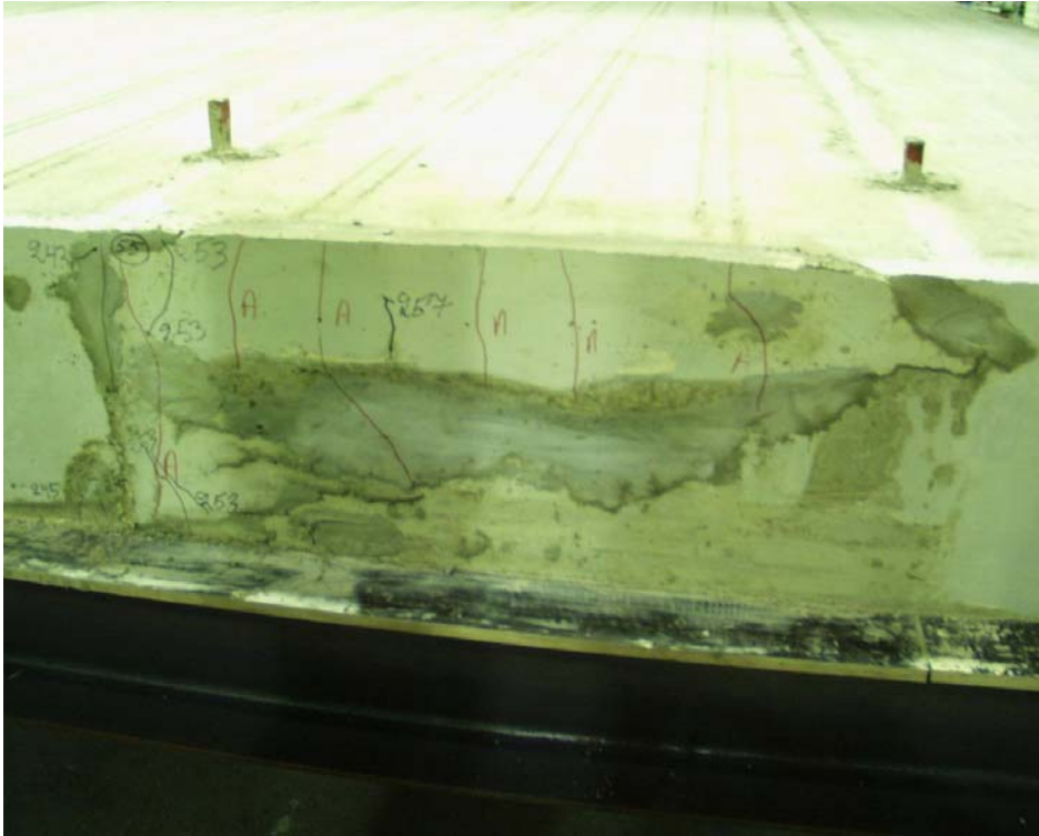
Fig. 35. Slab 8 after test. Cracks in tie beam. The read line and capital A indicate an initial crack. The nonuniform colour is due to a mortar treatment carried out after demolding.
