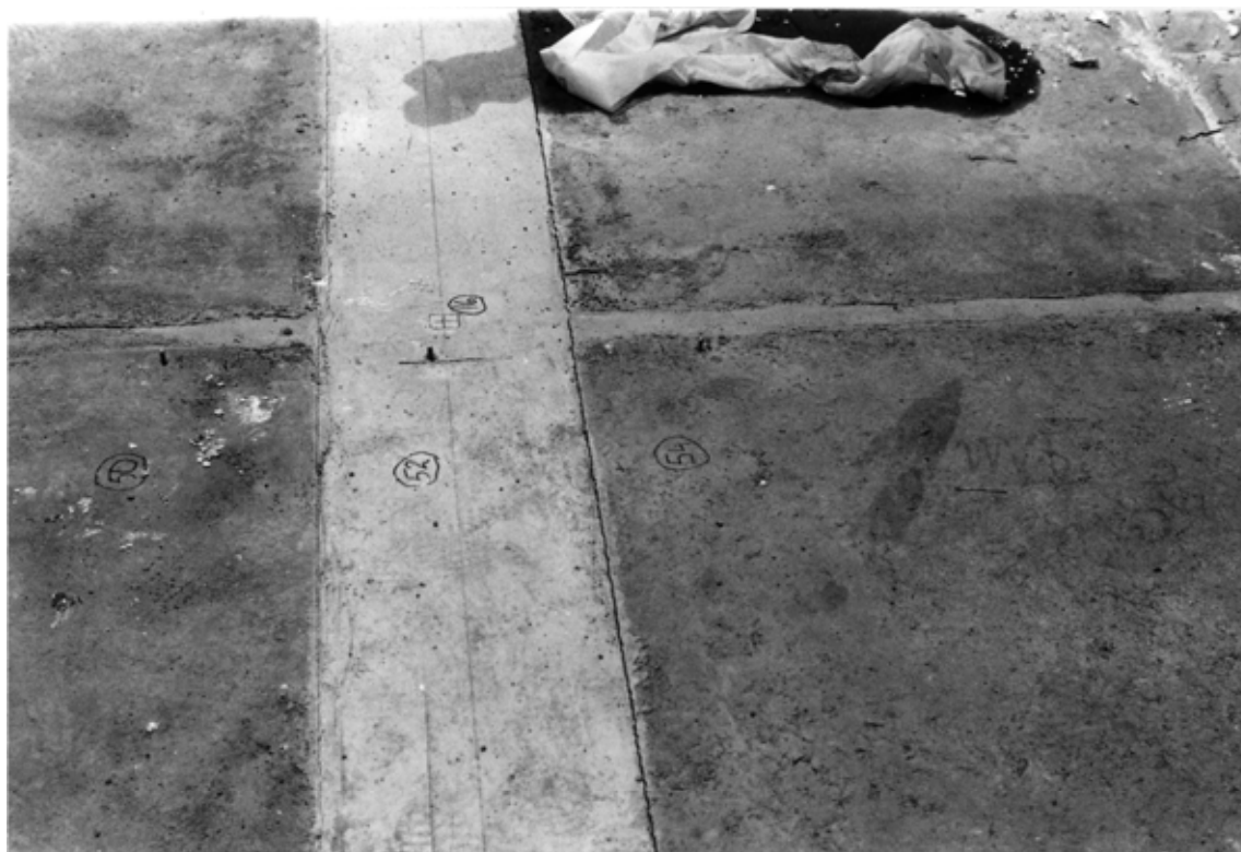
Fig. 11. Cracking of the joint between the cast in situ part of the middle beam and the ends of the slab units.
