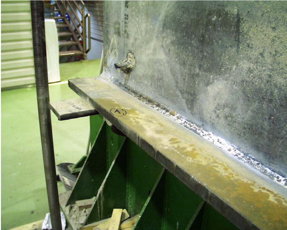
Fig. 53. Changes in colour on the flange below slab 1 due to the concrete or cement paste intruding into the gap between the soffit of the slab and the steel flange. See also the vertical stripes along the vertical edge of the flange.
