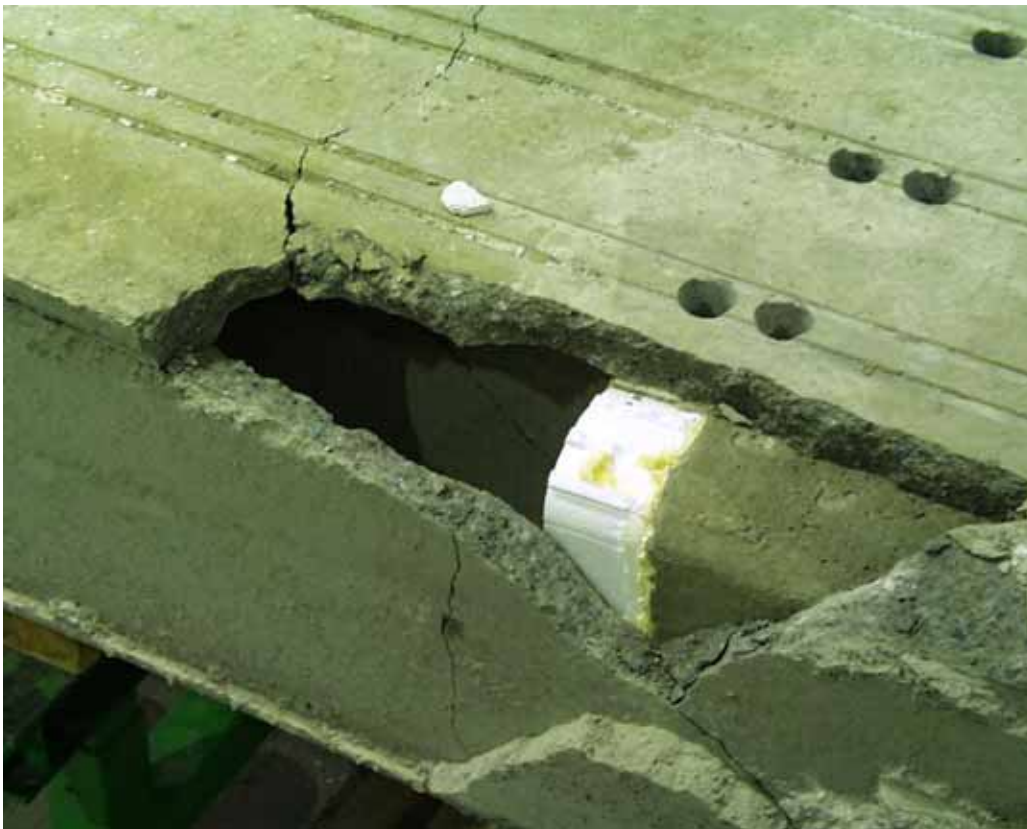
Fig. 22. Perfect filling in a hollow core of slab 1.
