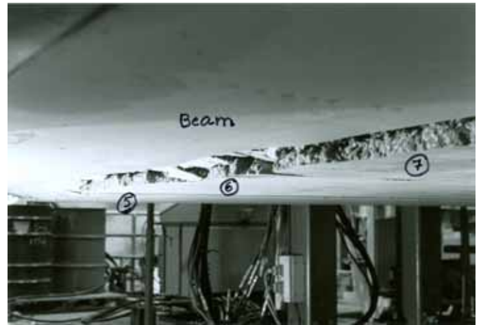
Fig. 14. Failure pattern of slab units 5–7 seen from below.
