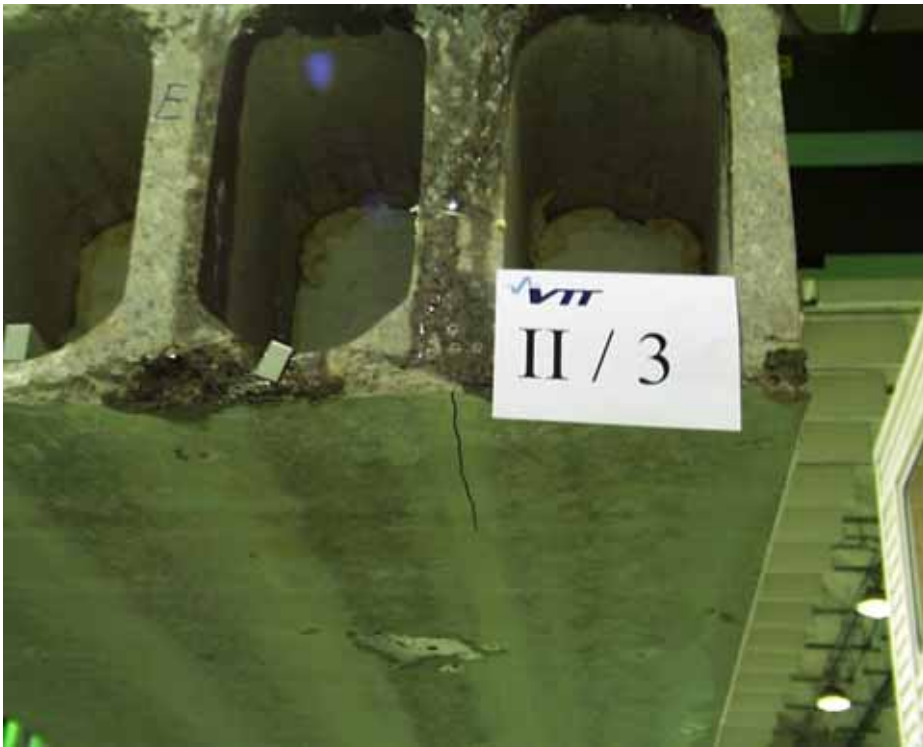
Fig. 5. Initial crack in slab 3.
