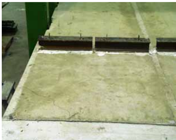
Fig. 17. Cracks in slab 5 after failure.
