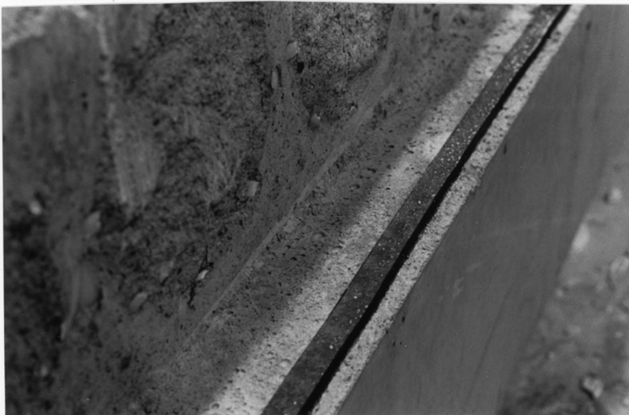
Fig. 22. Concrete infill below the slab ends. Note that the grout has properly filled the space. Note also the pores due to the air bubbles.
