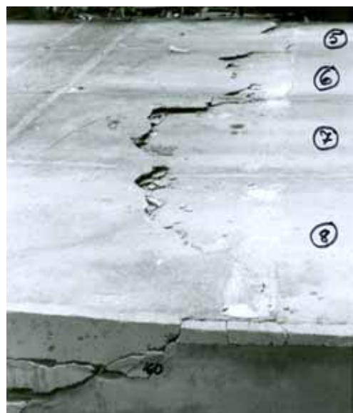
Fig. 12. Failure pattern of slab units 5–8 seen from above.
