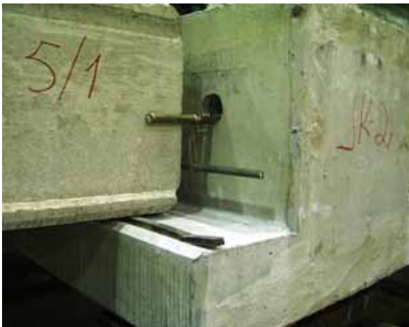
Fig. 3. Reinforcement at the end of middle beam. One rebar parallel to the beam on the top of the joint is still missing.
