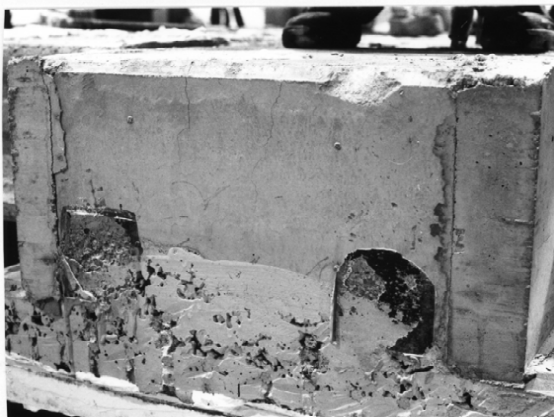
Fig. 23. Cracking of end 1 of middle beam.
