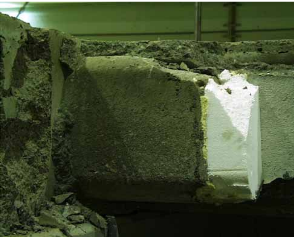
Fig. 26. The only observed incomplete filling in hollow core.
