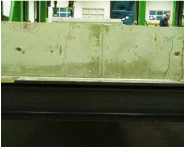
Fig. 19. Cracks in Eastern tie beam after failure. Slabs 7–8.
