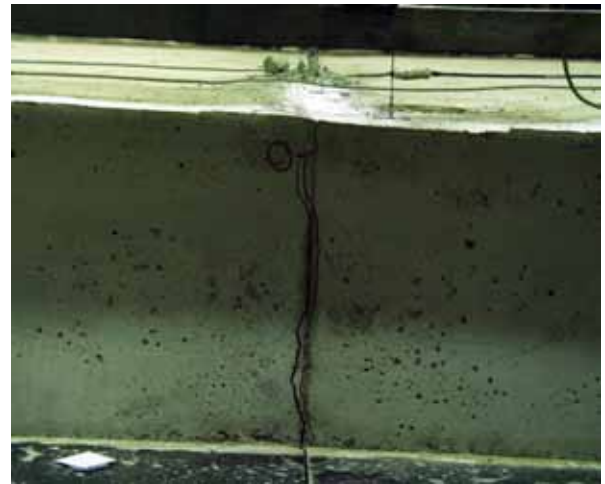
Fig. 12. Vertical cracking of end beam between slabs 6 and 7.
