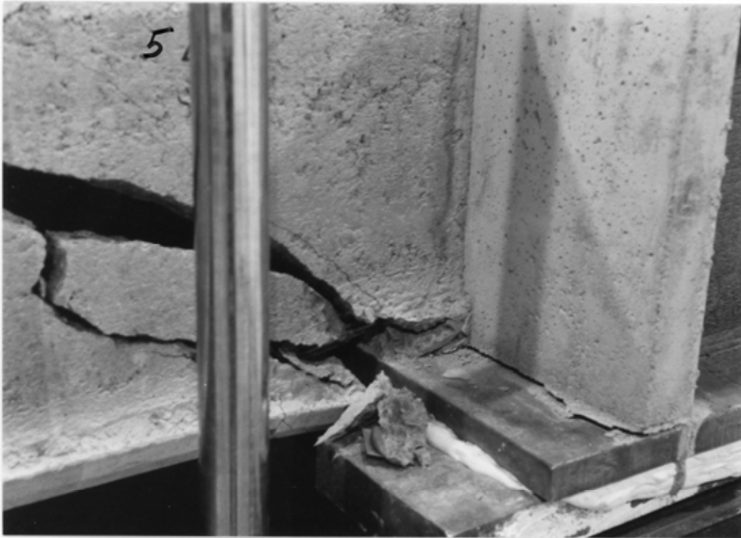
Fig. 5. Failure at stage 1. The narrow crack above the failure crack appeared first. Its growth could be followed visually until failure.
