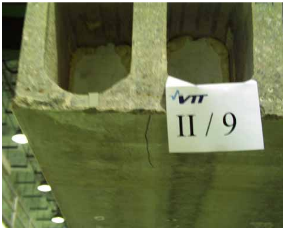
Fig. 7. Initial crack in slab 9.
