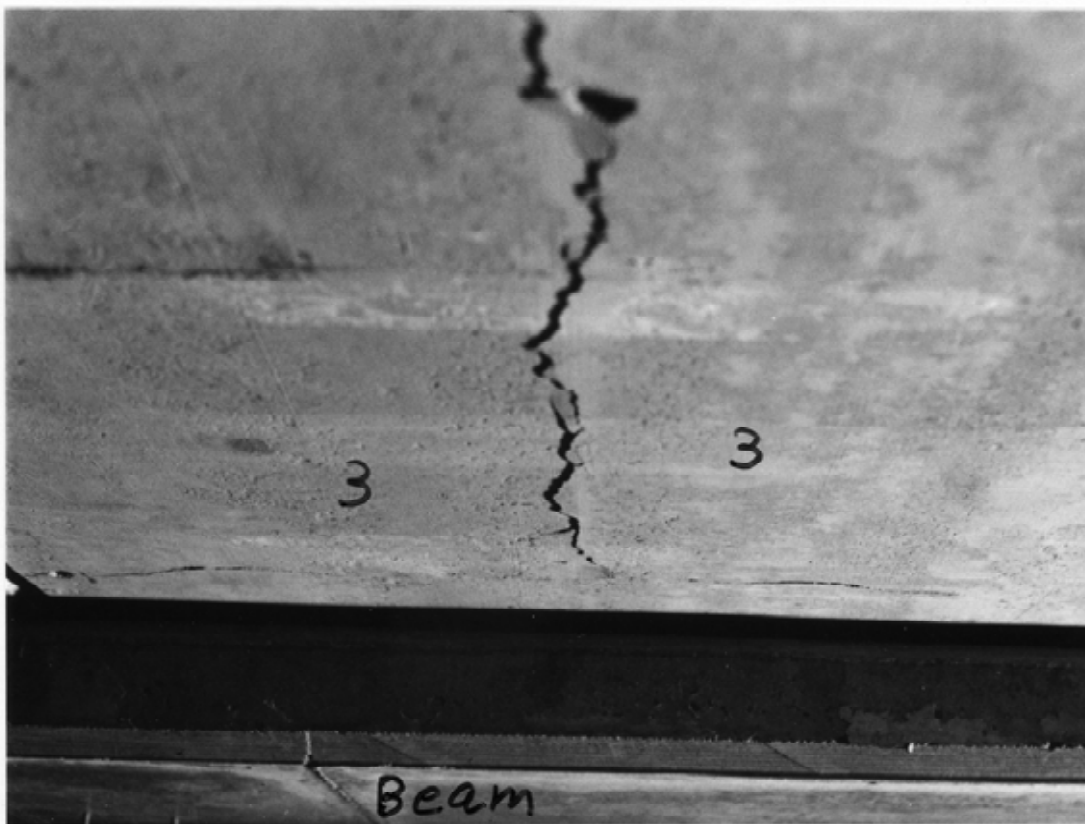
Fig. 18. Longitudinal and transverse cracking of slab unit no 3 seen from below.
