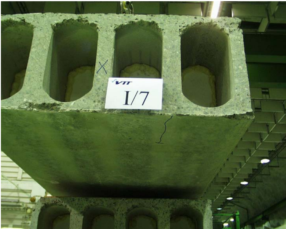
Fig. 7. Initial crack in slab 7.
