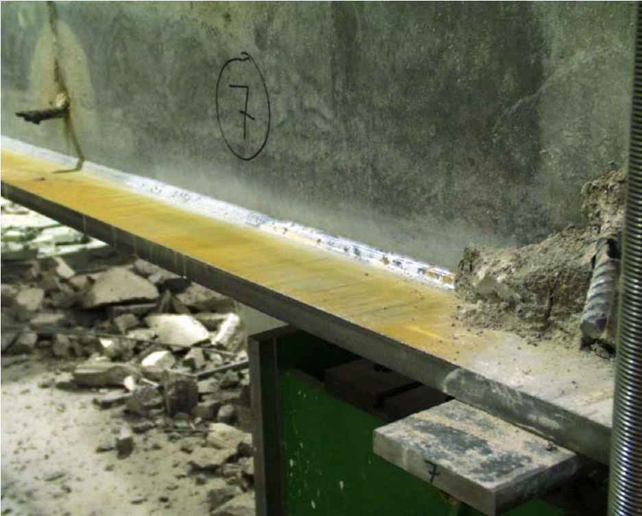
Fig. 59. Steel flange below slab 7. No clear sign of grout can be seen below the slab and above the flange.
