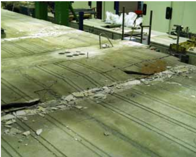
Fig. 21. Failure in slabs 5–7.
