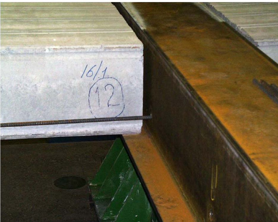
Fig. 12. Slab 12 on WQ beam and a tie bar 20 mm.
