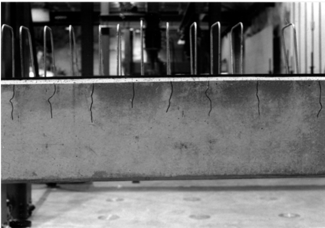
Fig. 2. Cracking of the middle beam before the loading test.
