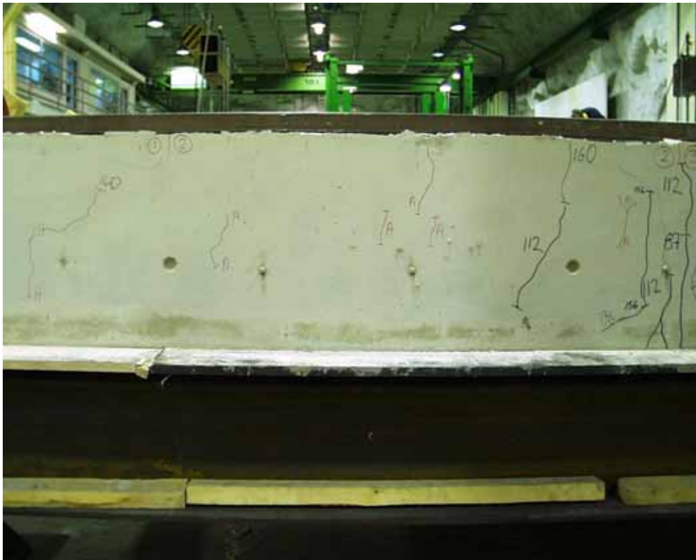
Fig. 25. Western end beam. Cracks in cast in-situ concrete at the end of slabs 1 and 2.
