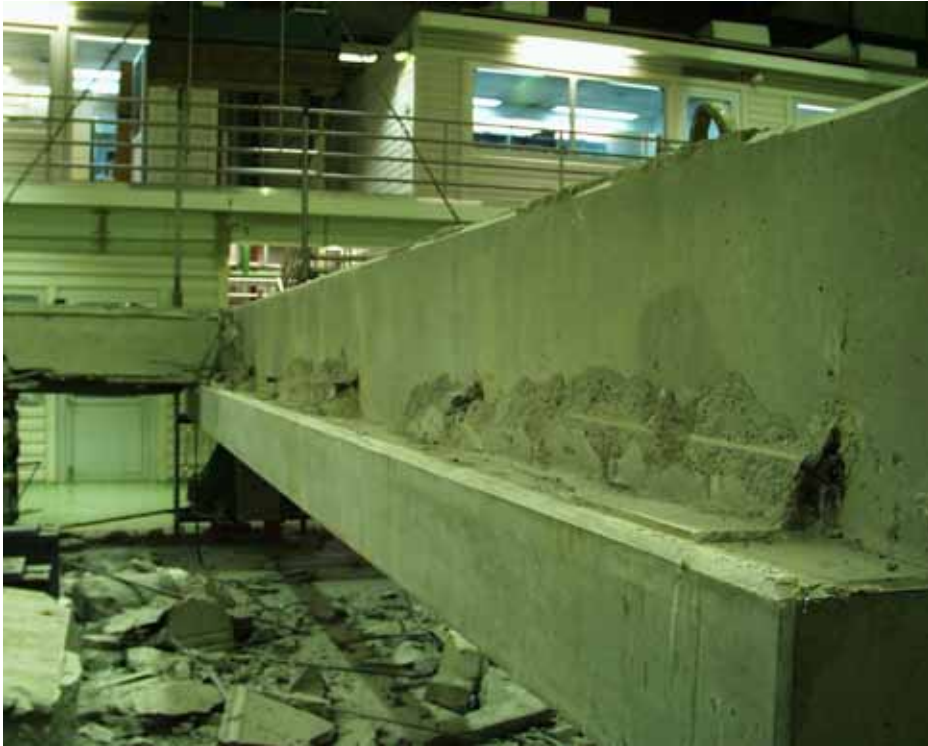
Fig. 29. Vertical cracking at slab ends took place along the web of the beam.
