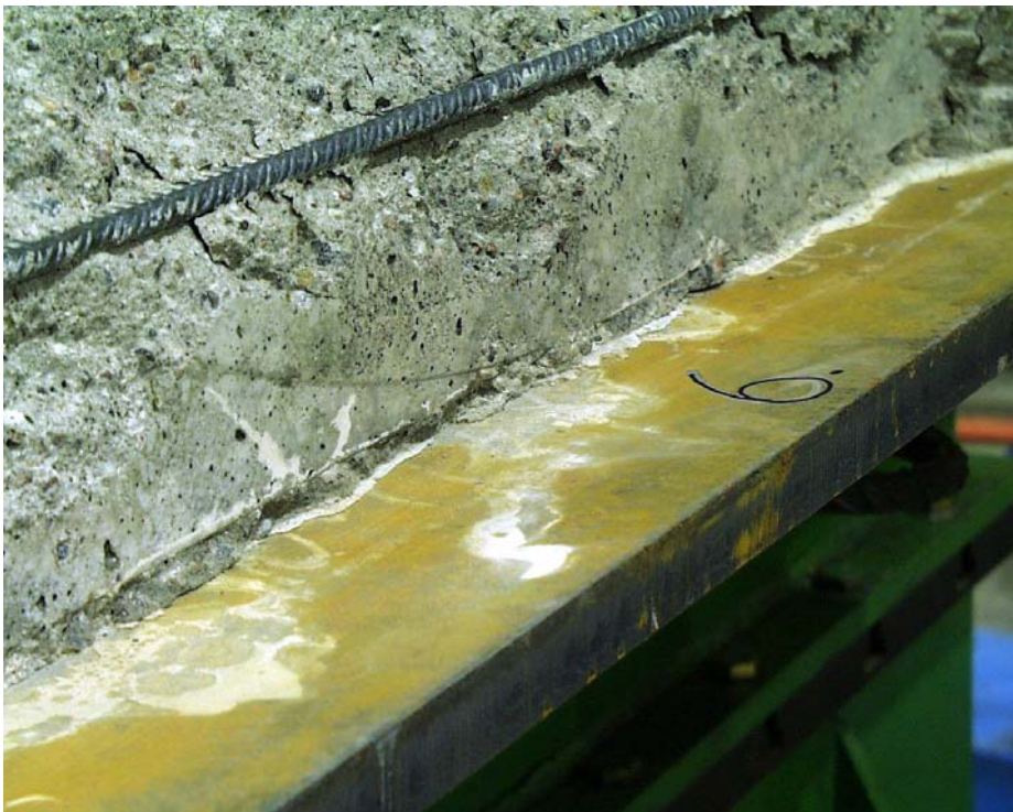
Fig. 56. Thin layers of grout as well as changes in colour on the flange below slab 1 due to the grout intruding into the gap between the soffit of the slab and the steel flange.
