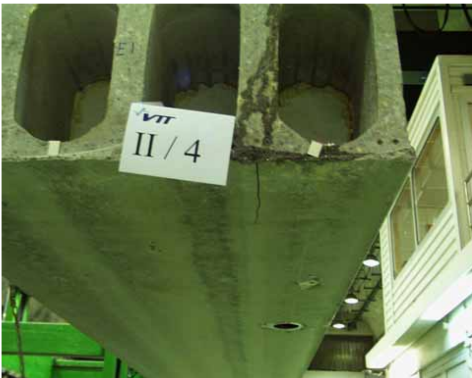
Fig. 6. Initial crack in slab 4.
