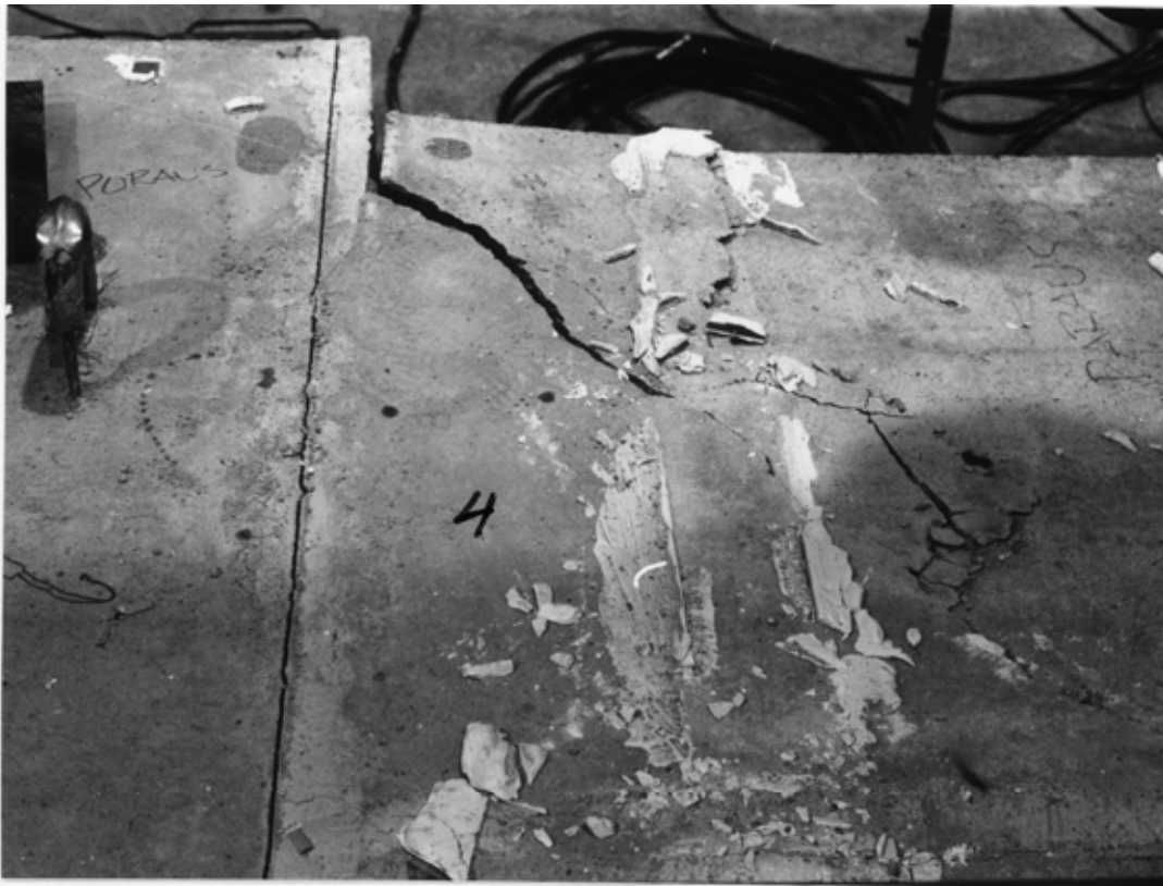
Fig. 13. Failure of slab unit no 4 seen from above.
