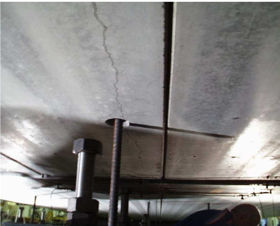
Fig. 24. Longitudinal crack in the soffit of slab 10 at P_a = 160 kN. The cracking took place at P_a = 109 kN.
