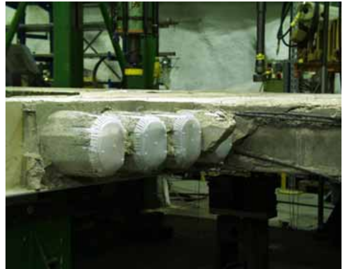
Fig. 22. Western side of middle beam. Note the bond failure along the vertical interface of the cast-in-situ concrete and the precast beam as well as the intact core fillings.
