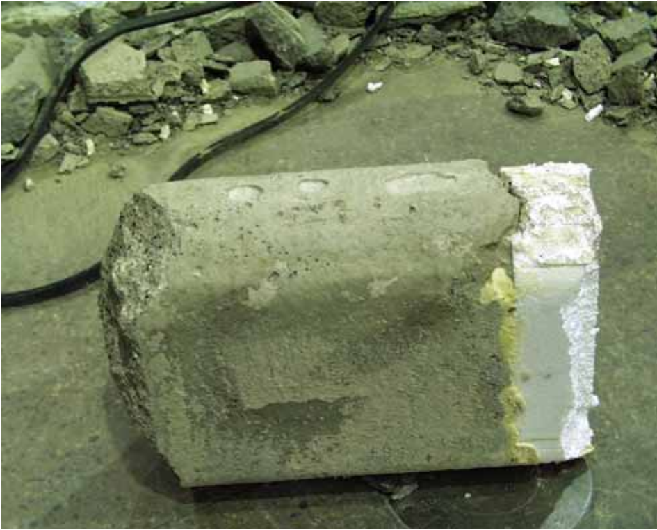
Fig. 25. Perfect filling of hollow core. Note the lack of bond between the cast-in-situ and precast concrete.
