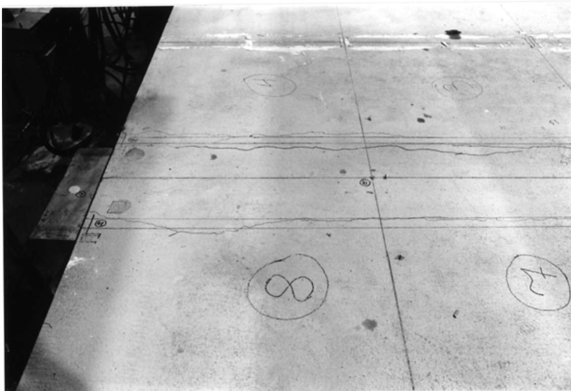
Fig. 16. The cracking of the concrete topping along the joint between the middle beam and the ends of the slab units no 3 - 4 and no 7 - 8.
