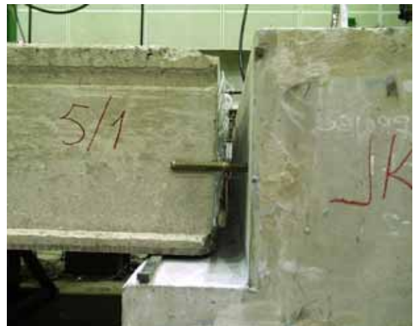
Fig. 4. Reinforcement at the end of middle beam. One rebar parallel to the beam on the top of the joint is still missing.
