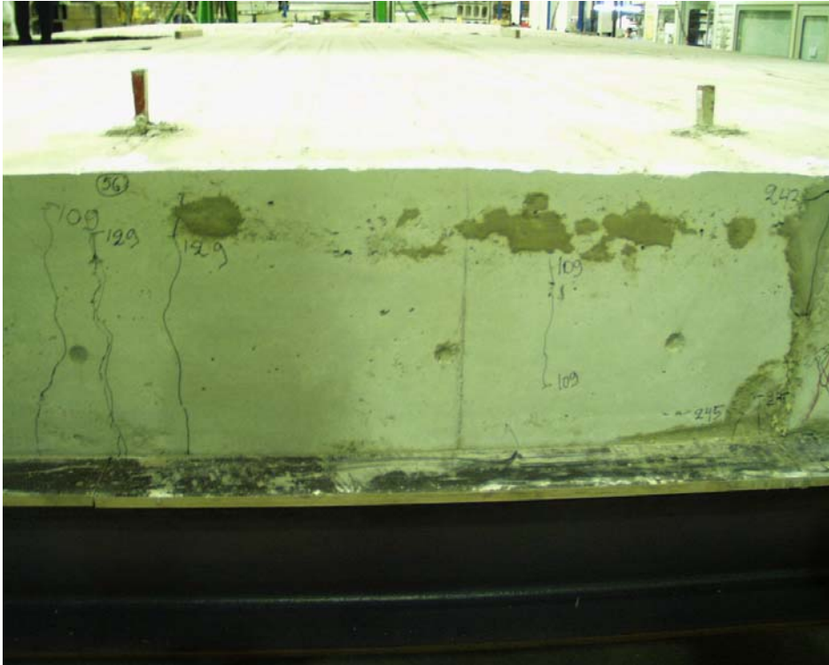
Fig. 36. Slab 9 after test. Cracks in tie beam.
