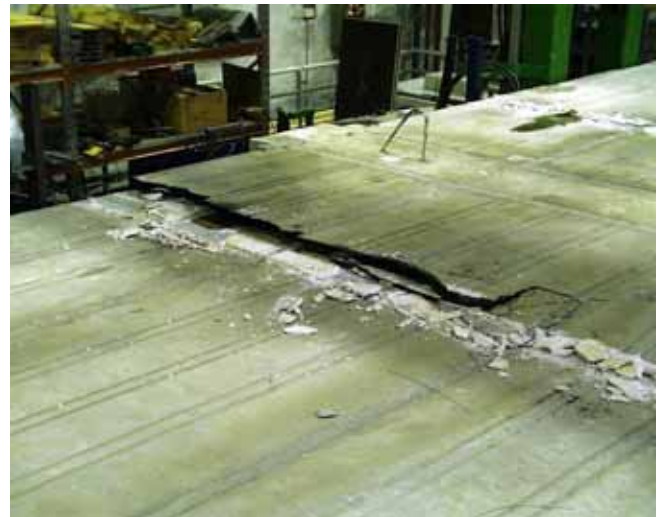
Fig. 22. Failure in slabs 6–8.
