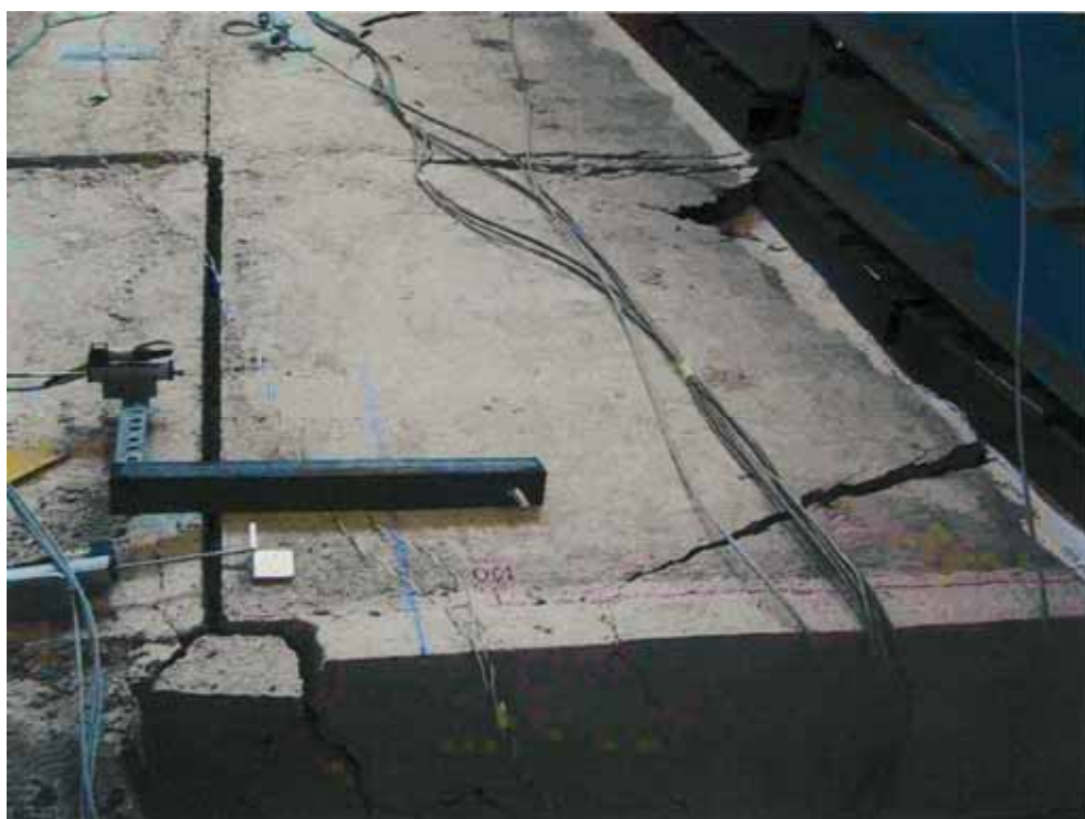
Fig. 4. Failure in slab 8.
