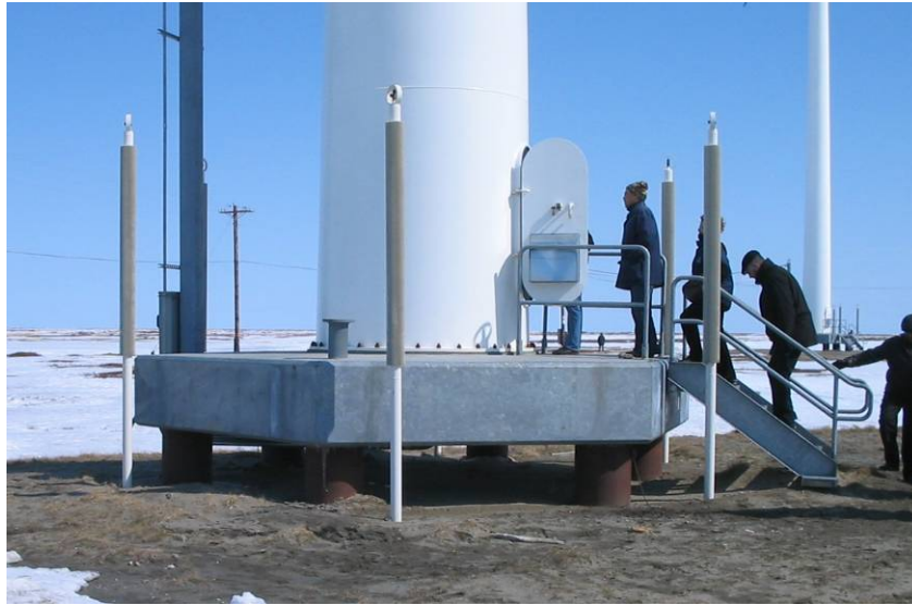
Figure 12. Permafrost foundation for a 100 kW wind turbine in Alaska using thermo siphons and freeze back peers driven into the permanently frozen layers. Photo credit Ian Baring-Gould.
