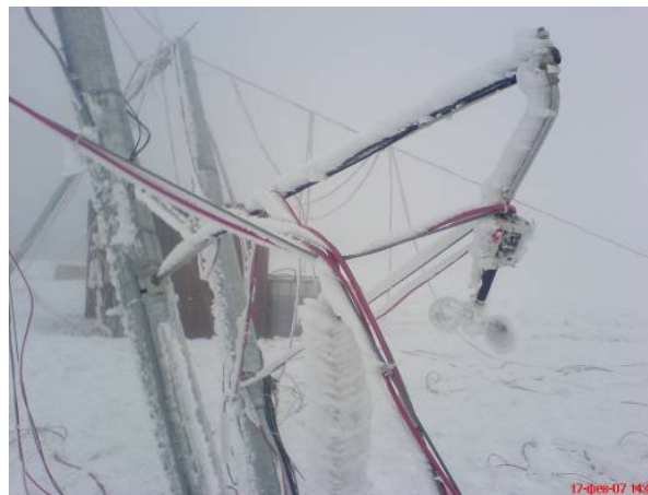
Figure 4. Collapsed meteorological tower, likely due to heavy icing.
