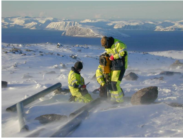
Figure 16. Work in extreme and cold climates requires specialized equipment, increased focus on personnel safety and expanded planning. Photo credit: Lars Tallhaug, Norway.
