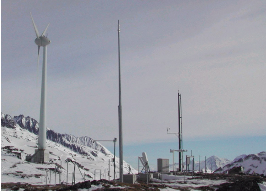
Figure 12. Installation on Mt. Gütsch with Enercon E-40 and test bench of the Swiss Met Institute.
