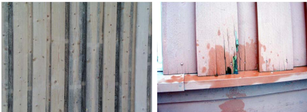
Figure 6. Mould and blue stain are the first step for the development of grayish color of wood surface. The response of wood to ambient humidity and discoloring vary (left). The decay damages are located in the details where water will be accumulated (right).
